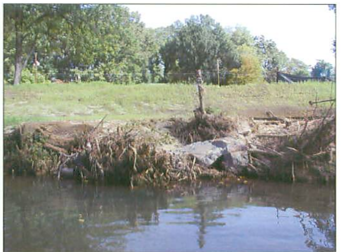
PP33B Reach 2 Rootwad #2 Before Repairs
