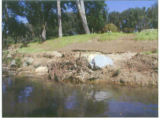
PP34B Reach 2 Rootwad #3 Before Repairs
