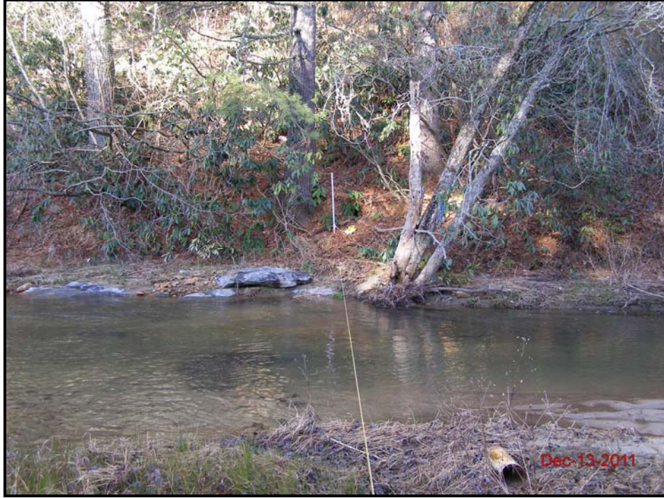
Glade Creek – Cross-Section 2 – Pool (Looking at Left Bank Descending) Monitoring Year 1 – December 13, 2011
