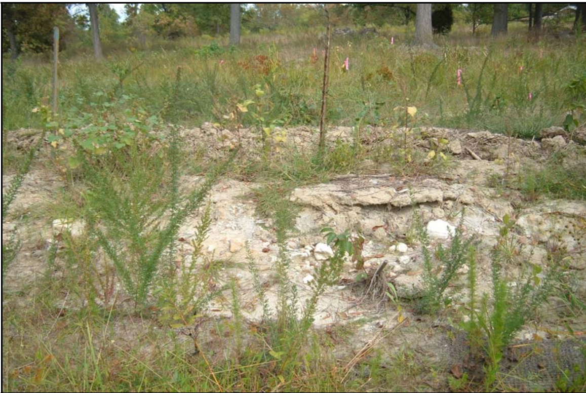
SP2 – Problem Area #4. Bank erosion beneath washed away matting. 10/3/07 - MY 01
