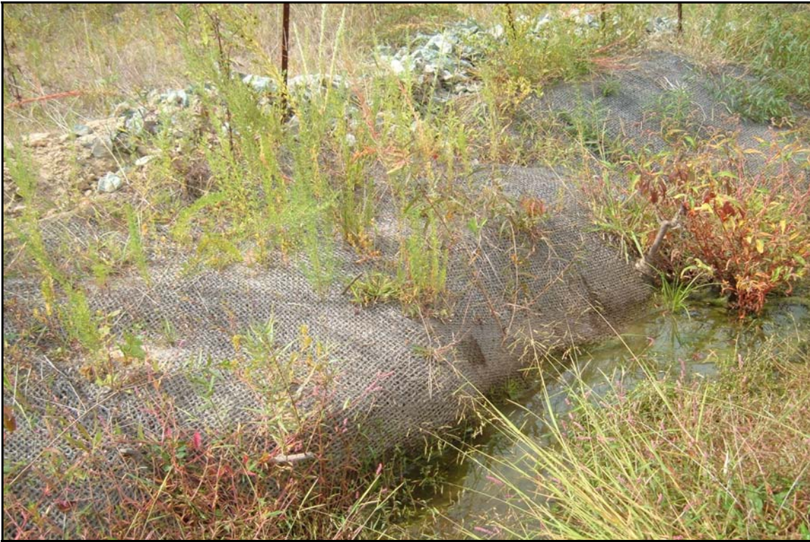
SP3 – Problem Area #11. Bank erosion on toe of bank beneath matting. 10/3/07 - MY 01
