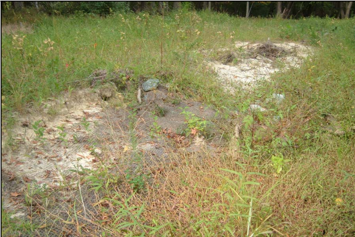
SP4 – Problem Area #17. Bank and floodplain erosion beneath washed away matting and remaining matting. 10/3/07 - MY 01
