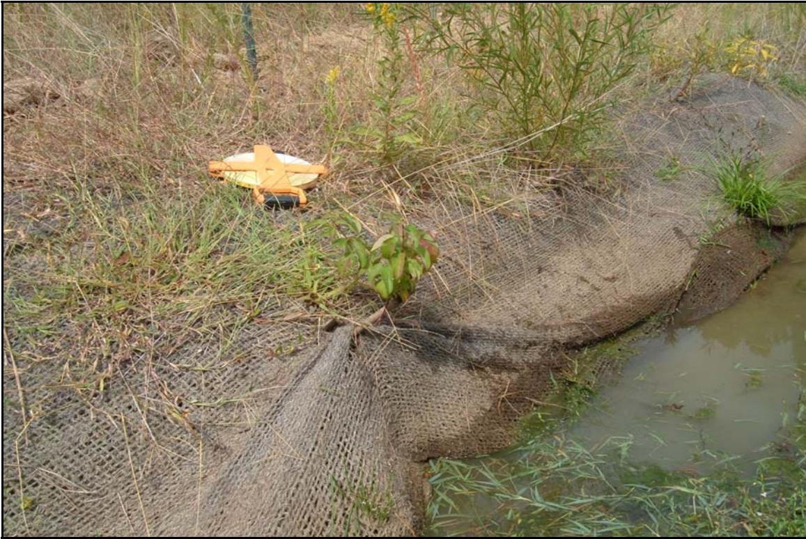
SP1 – Problem area #1. Erosion on toe of bank beneath matting. 10/3/07 - MY 01
