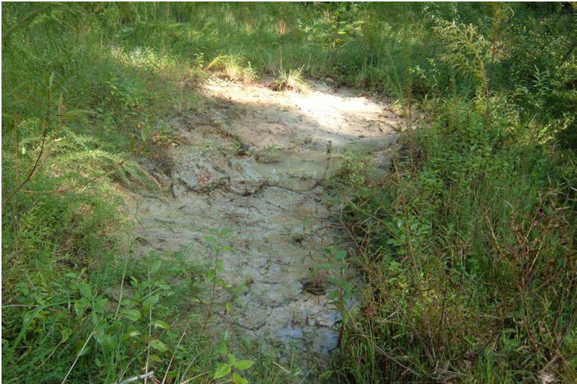
Floodplain Erosion – Stationing 36+20 – 36+40 09/29/08 - MY 02
