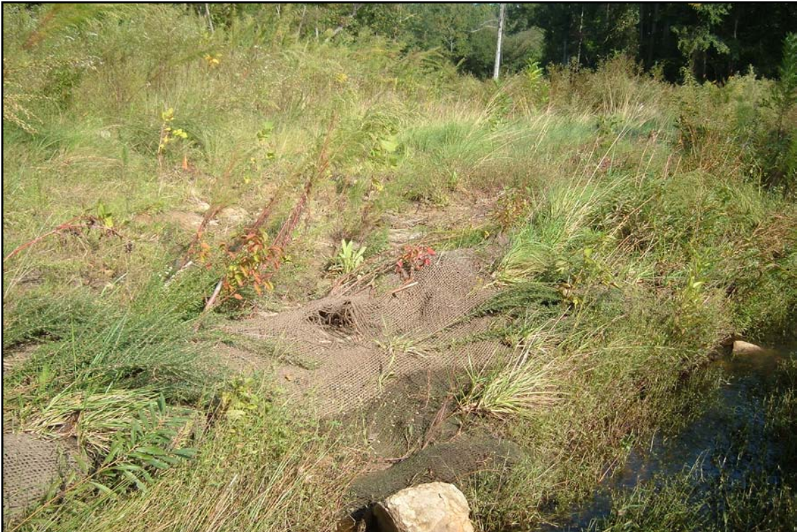
Bank/Floodplain Erosion – Bank erosion under matting and upper bank and floodplain erosion. Stationing 28+80 – 28+95 09/29/08 - MY 02
