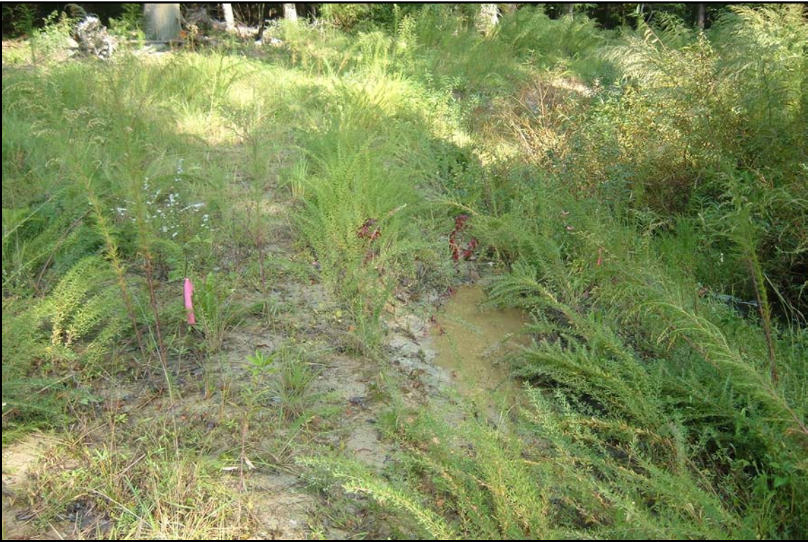
Floodplain Erosion – Upper bank and floodplain erosion. Stationing 36+00 – 36+10 09/29/08 - MY 02
