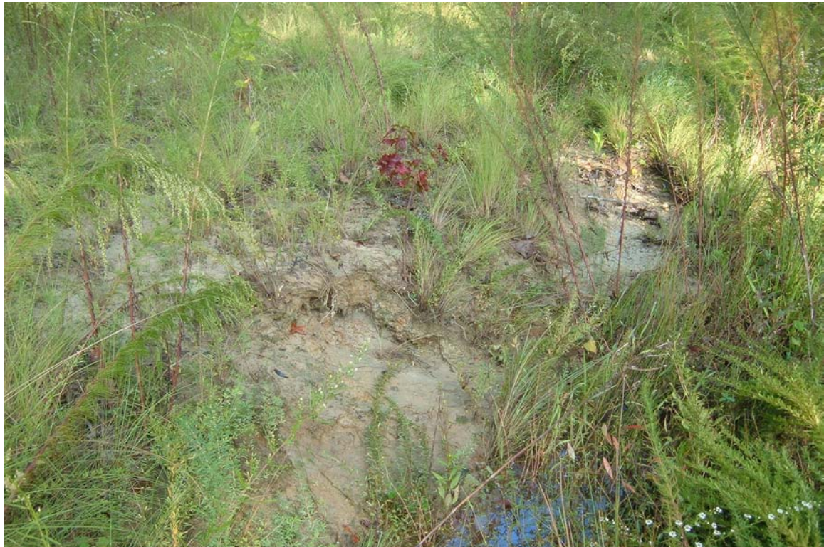
Floodplain Erosion – Stationing 34+40 – 34+60 09/29/08 - MY 02
