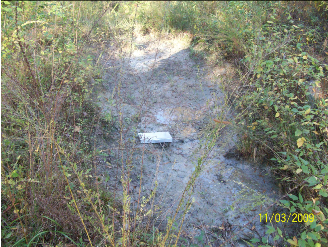
SP1 – Upper bank and floodplain erosion. Stationing 36+20 – 36+50 11/3/09 - MY 03
