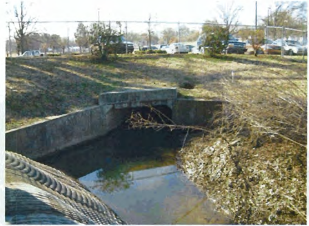
Photograph 2. Looking upstream at culvert outfall from Taylor Street and parking lot at Eastway Elementary School, demarking upstream limit of Eastway Elementary School Reach. (1/21/04)
