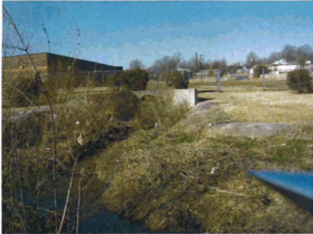
Photograph 7. Looking at concrete headwall and 60" RCP draining west side of Goose Creek. (1/21/04)
