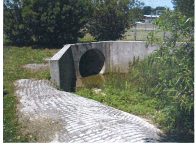
Photograph 8. Closer view of concrete headwall and 60" RCP draining west side of Goose Creek midreach. (5/23/05)
