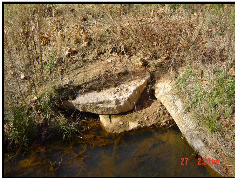
Typical Stressed Structure/Bank Scour—Reach 2—Year 1 (2006)
