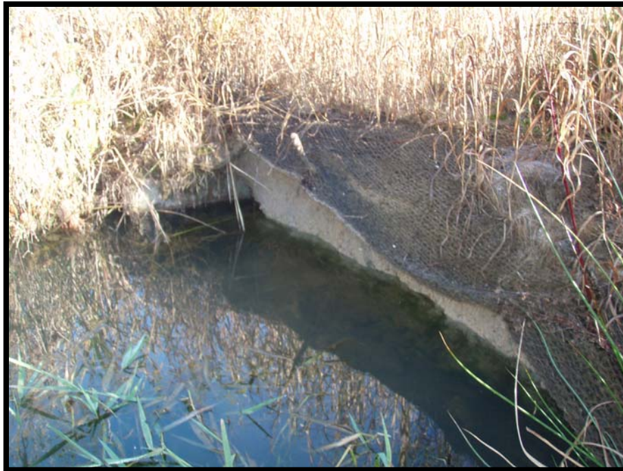
Photo 1—Typical Bank Scour—Reach 1—Year 2 (2007)
