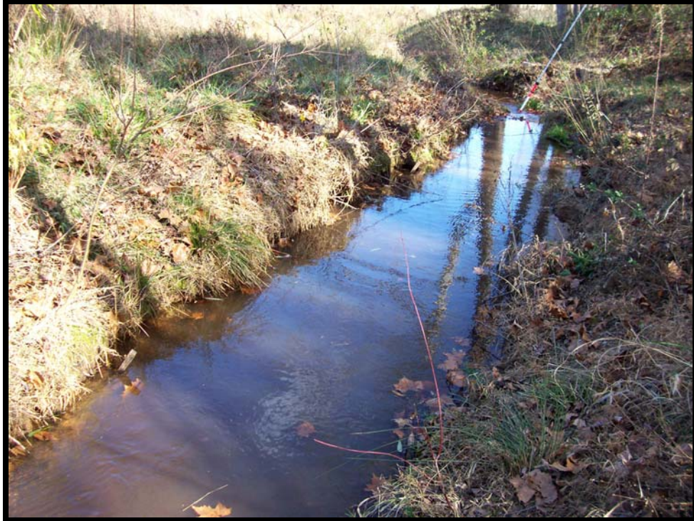
Photo 5 – Undercut Bank – Reach 1 – Year 3 (2008)
