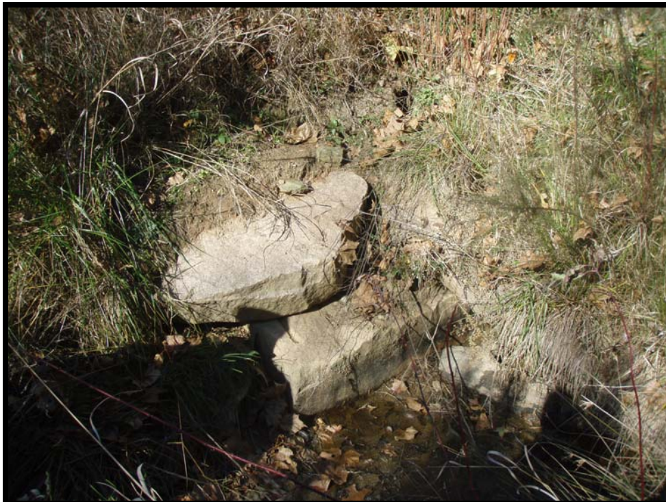
Photo 4 – Typical Stressed Structure/Bank Scour – Reach 2 – Year 3 (2008)
