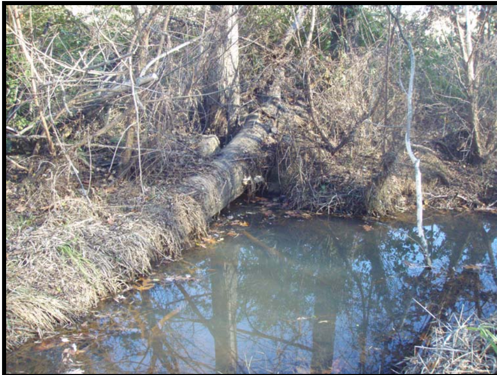
Photo 2 – Typical Stressed Structure/Bank Scour – Reach 1 – Year 3 (2008)
