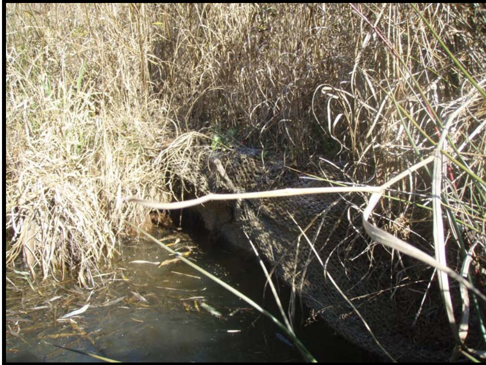
Photo 1 – Typical Bank Scour – Reach 1 – Year 3 (2008)
