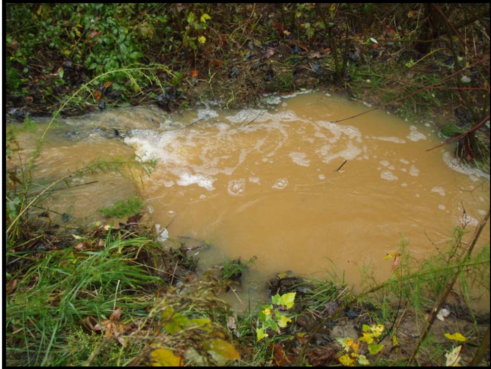
Photo 7 – Area of Channel Scour (Station 16+10 in Long Profile Section 2) – Reach 2 – Year 4 (2009)
