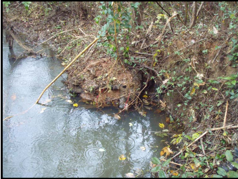
Photo 1 – Typical Stressed Structure/Bank Scour – Reach 1 – Year 4 (2009)
