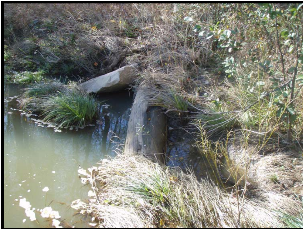
Photo 2 – Typical Stressed Structure/Bank Scour – Reach 1 – Year 4 (2009)
