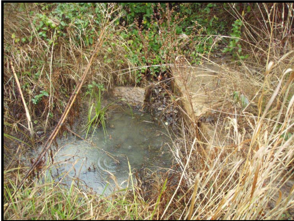
Photo 6 – Typical Stressed Structure/Bank Scour – Reach 2 – Year 4 (2009)
