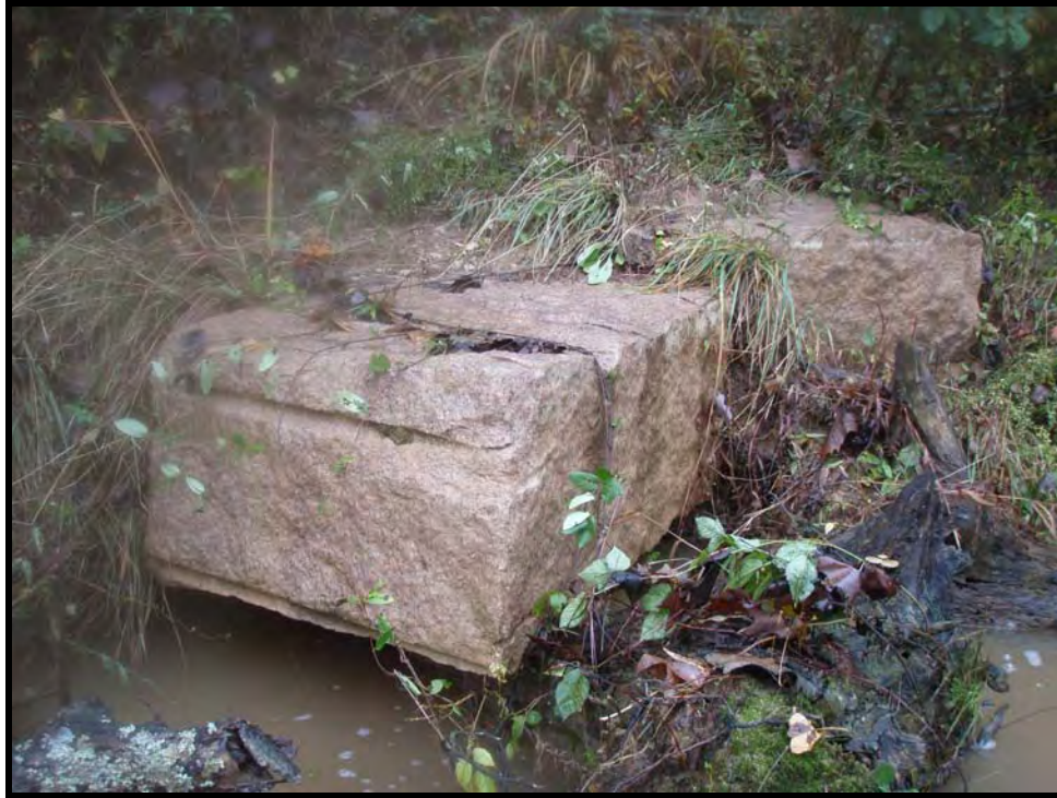
Photo 1 – Typical Stressed Structure/Bank Scour – Reach 1 – Year 5 (2010)
