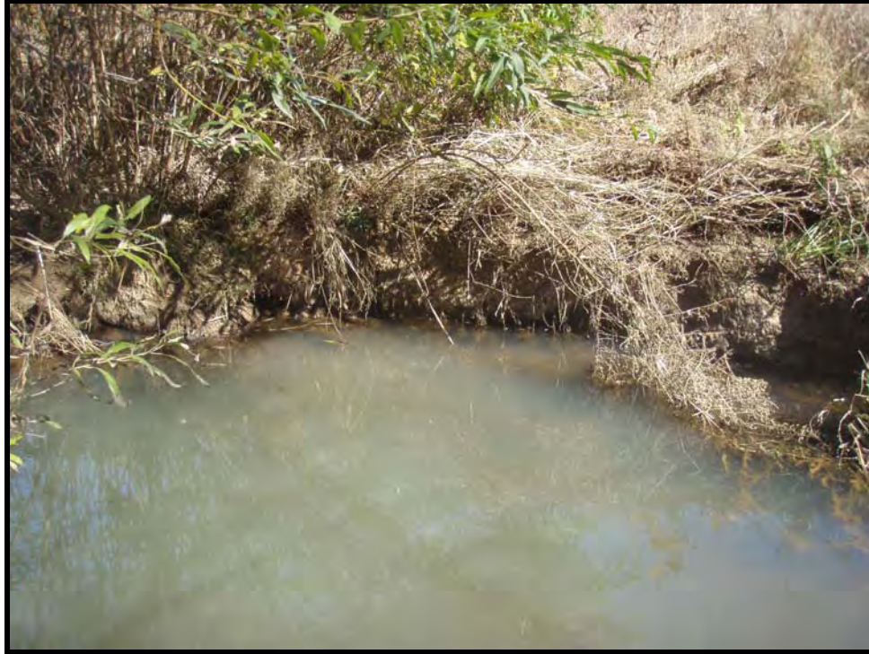
Photo 3 – Typical Undercut Bank – Reach 1 – Year 5 (2010)
