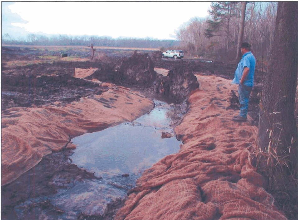
Photo P2. Root wads and coir fiber matting installed around a meander bend for bank stabilization and habitat improvement.
