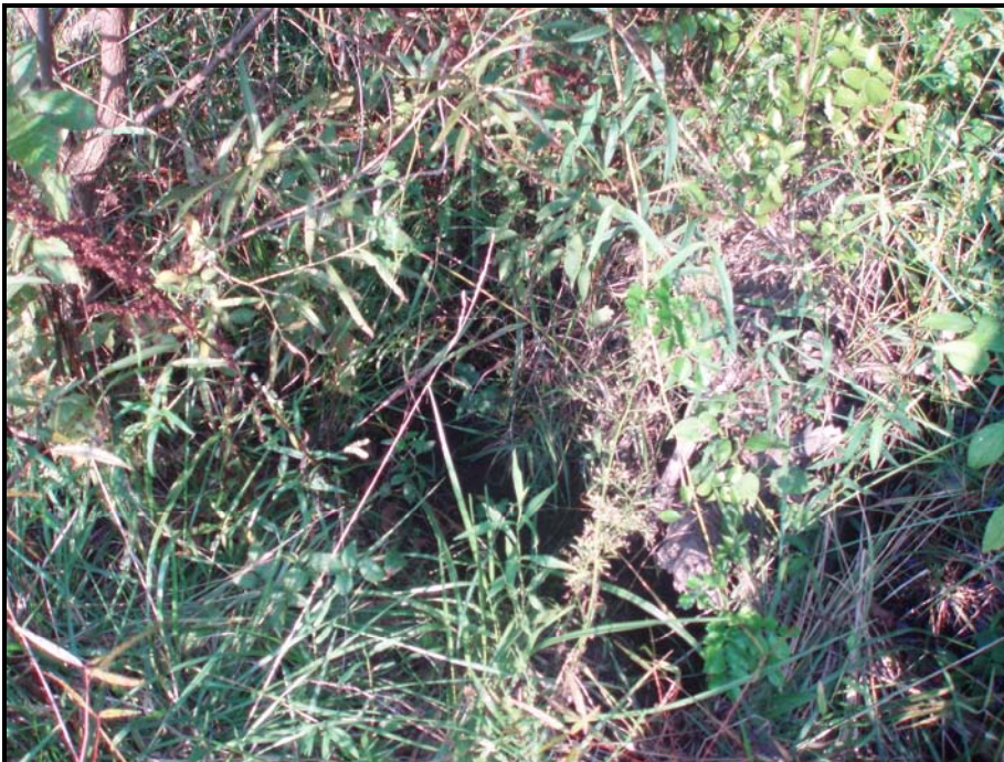
SPA 2. Erosion occurring between the left bank and installed root wad. STA 17+75
