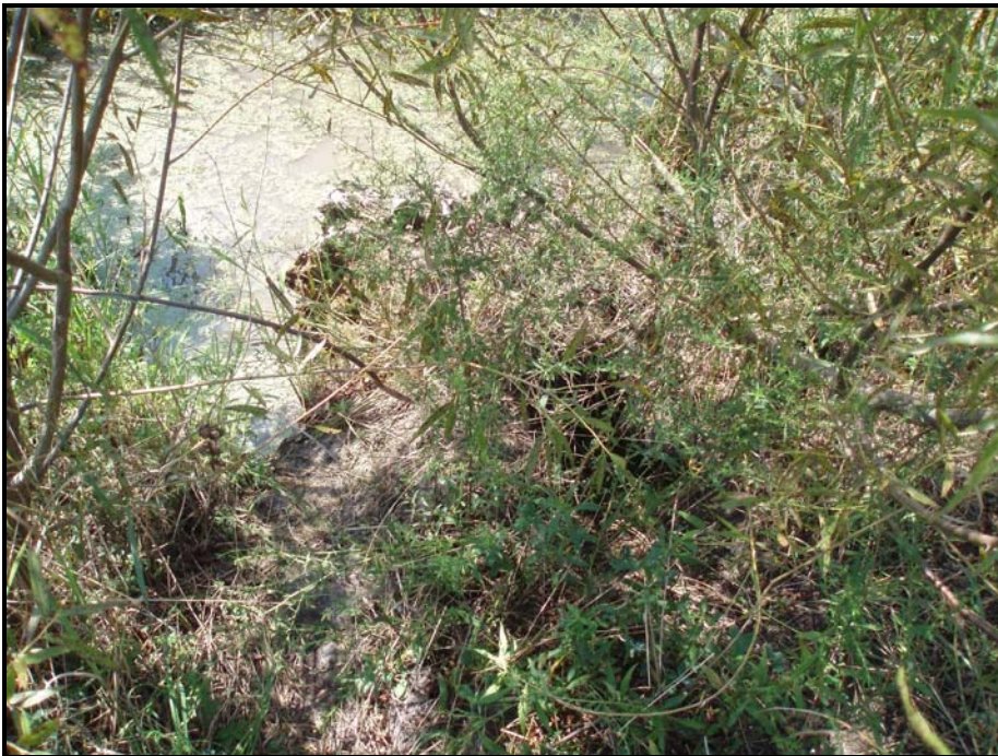
SPA 4. Erosion between left bank and installed root wad STA 42+00
