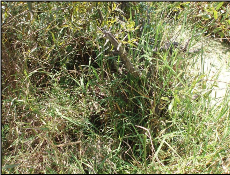
SPA 5. Erosion between left bank and installed root wad. Root wad is in the middle of the channel.
