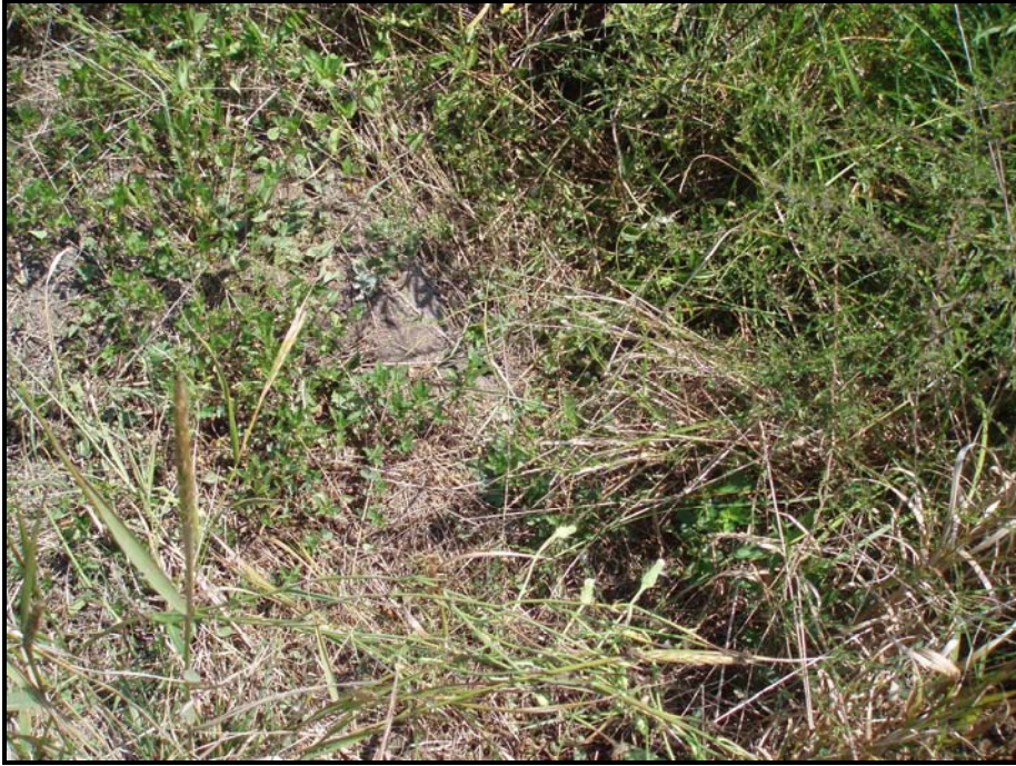
SPA 3. Erosion on left bank STA 37+80
