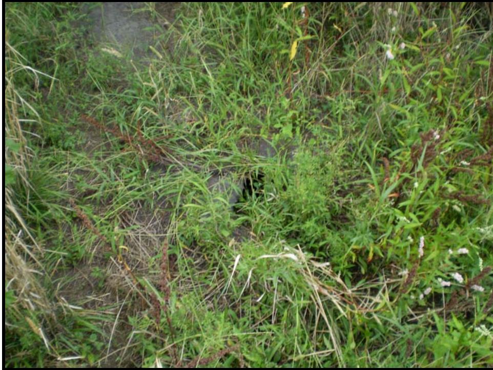
SPA 1. Right bank erosion at station 37+25.
