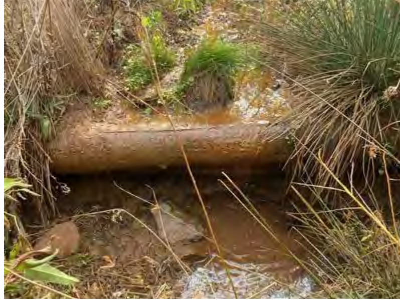
Structure Decline GF4-A
