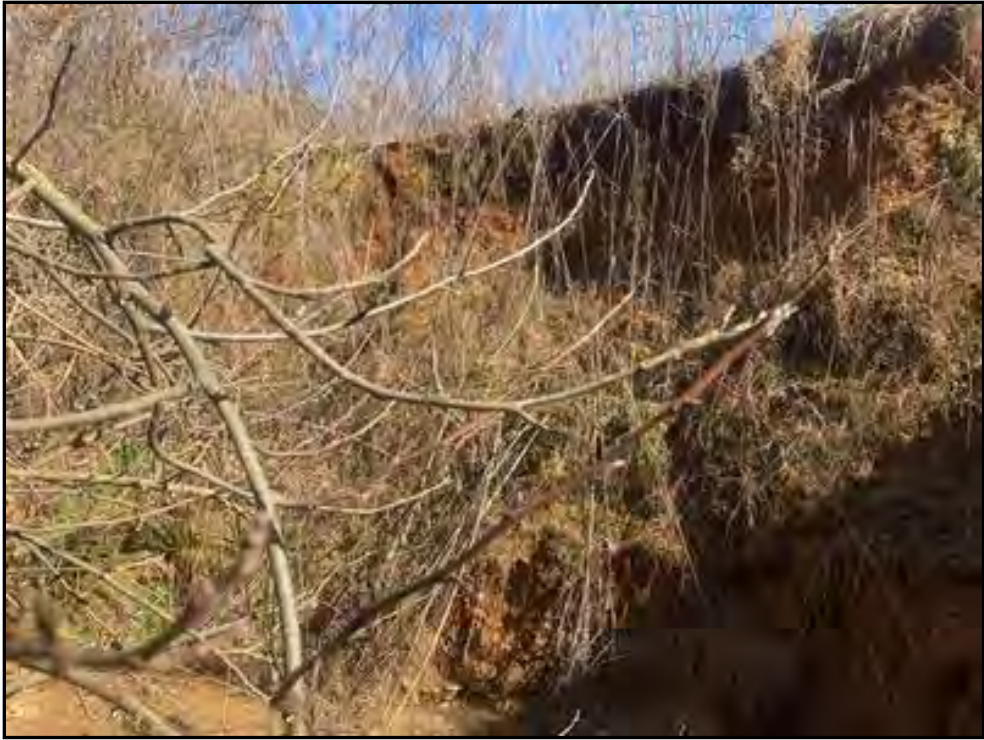
Eroding Slope – GF3A (02/13/2024)
