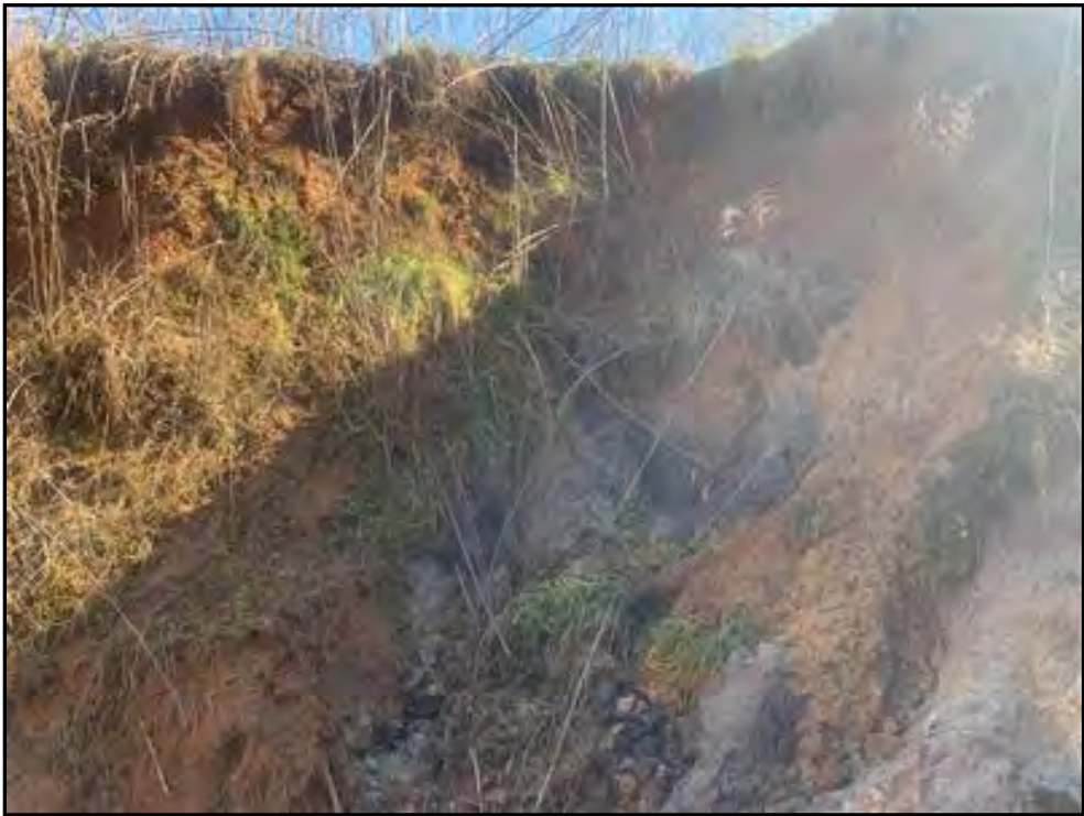
Eroding Slope – GF3A (02/13/2024)
