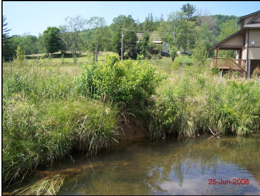
Stream Problem Area (SPA 3) – Bank scour Monitoring Year 5 – June 25, 2008
