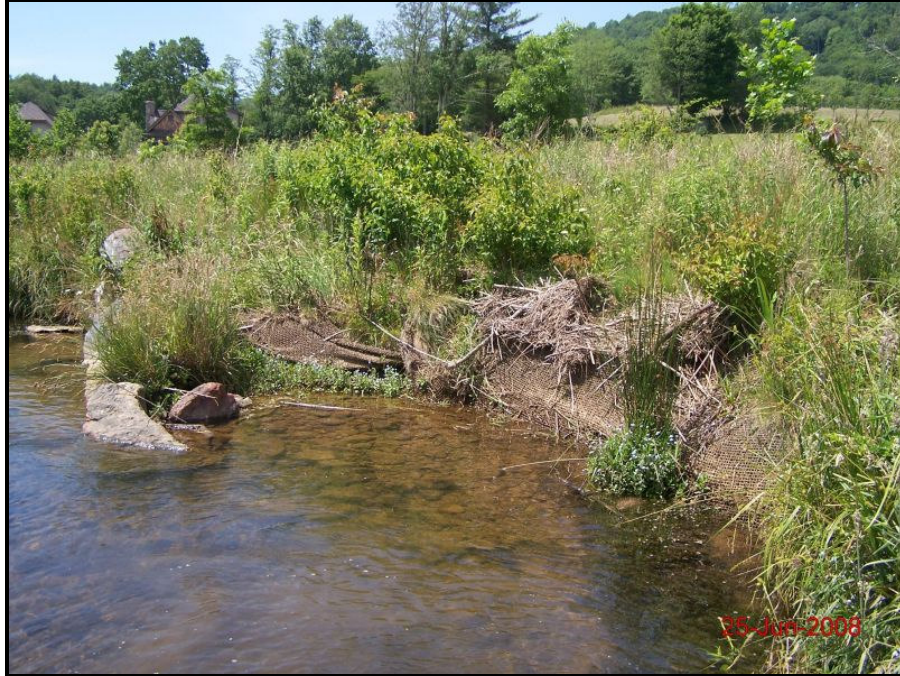
Stream Problem Area (SPA 5) – Stressed engineered structure Monitoring Year 5 – June 25, 2008
