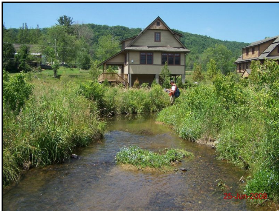
Stream Problem Area (SPA 2) – Mid channel bar associated with failing structure Monitoring Year 5 – June 25, 2008
