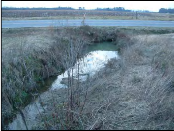
Beginning of the project stream as it leaves the culvert and enters the Harrell Property.
