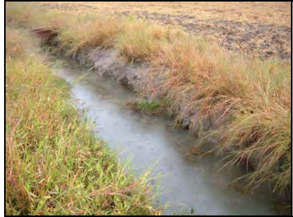
Exposed banks along the project stream.
