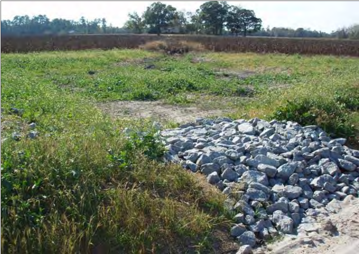
Photo Point S4: View of water quality treatment structure near Station 32+25. 11/7/07 – As-Built
