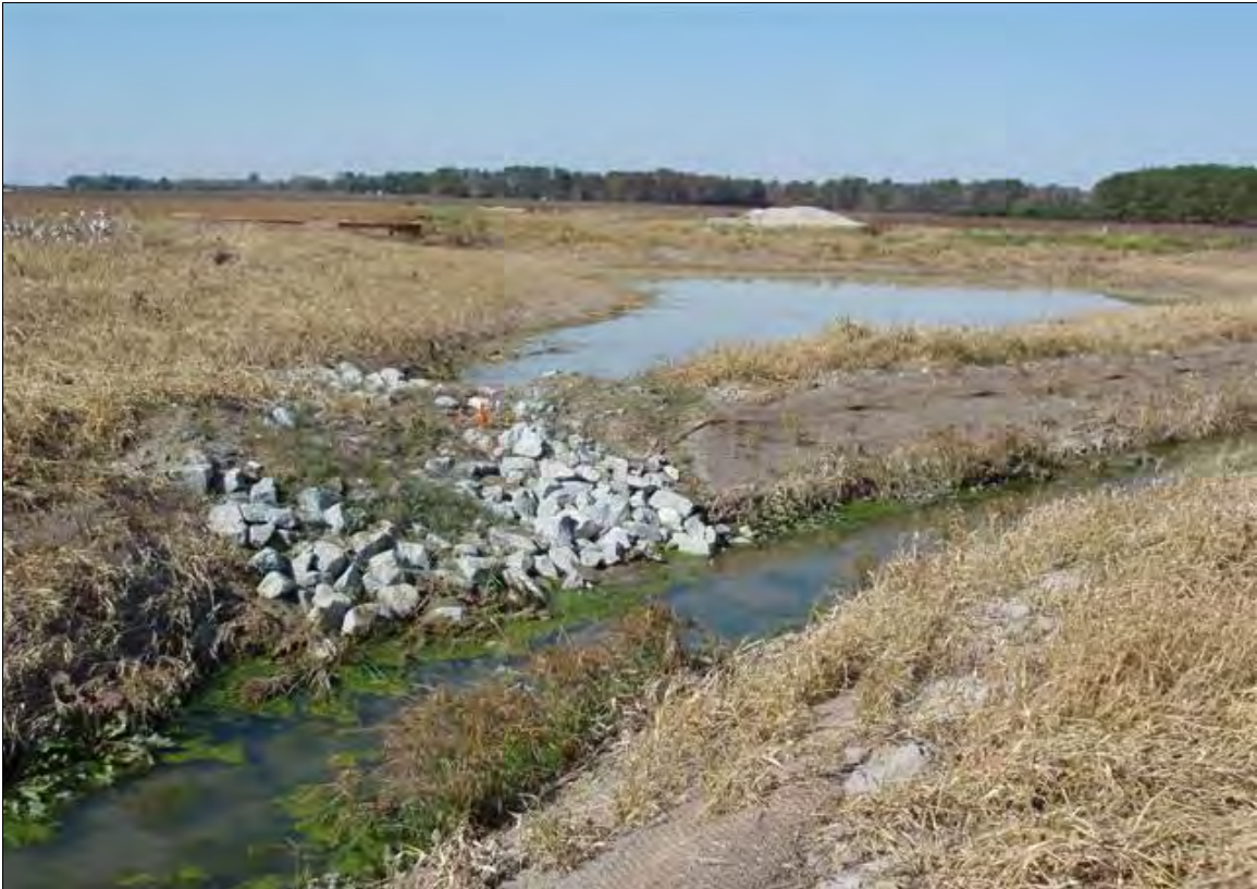
Photo Point S14: View of water quality treatment structure near Station 62+60. 11/7/07 - As-Built
