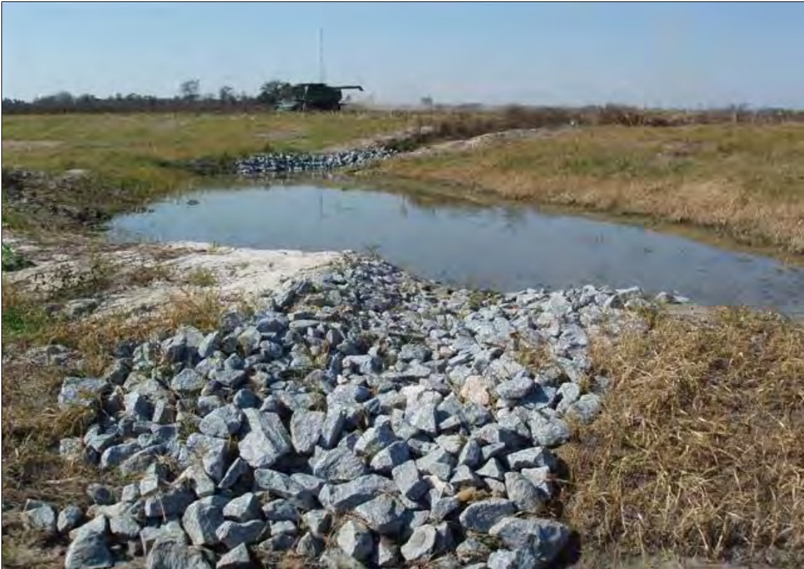
Photo Point S11: View of water quality treatment structure near Station 47+00. 11/7/07 - As-Built
