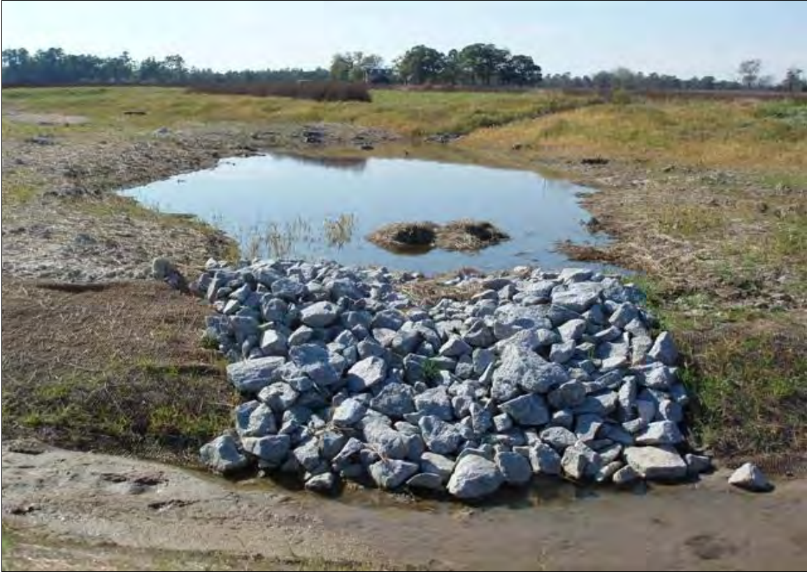
Photo Point S9: View of water quality treatment structure near Station 41+75. 11/7/07 – As-Built
