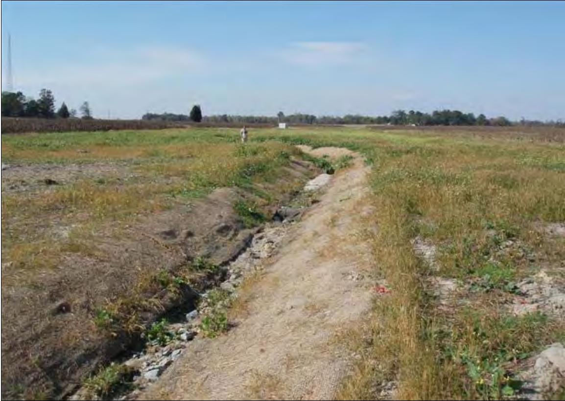
Photo Point S5: View looking at log drop structures, near Station 33+35. 11/7/07 – As-Built
