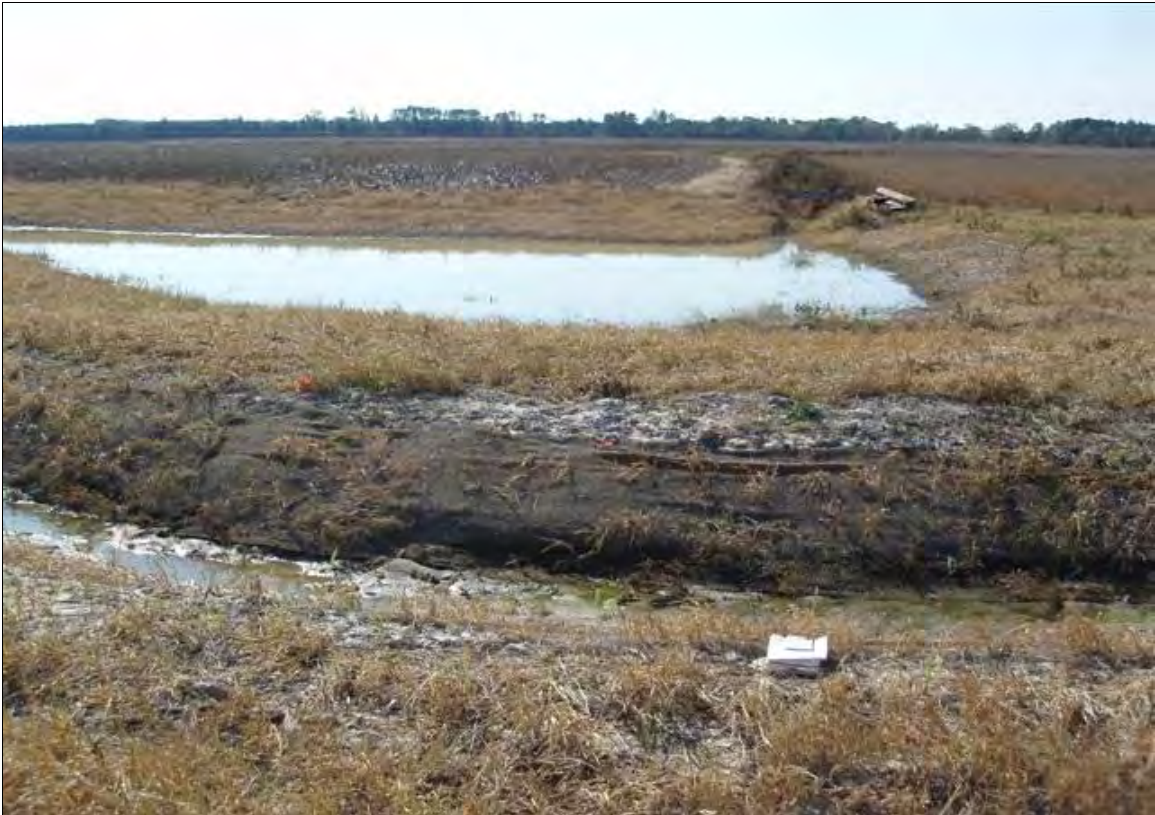
Photo Point S13: View of water quality treatment structure near Station 61+50. 11/7/07 - As-Built
