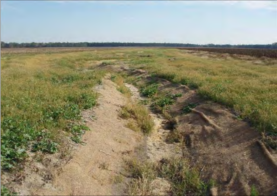
Photo Point S2: View looking downstream from farm road near Station 21+30. 11/7/07 - As-Built
