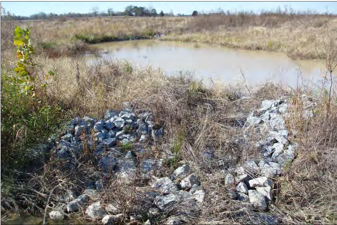
Photo Point S11: View of water quality treatment structure near Station 47+00. 11/19/08 - MY-01
