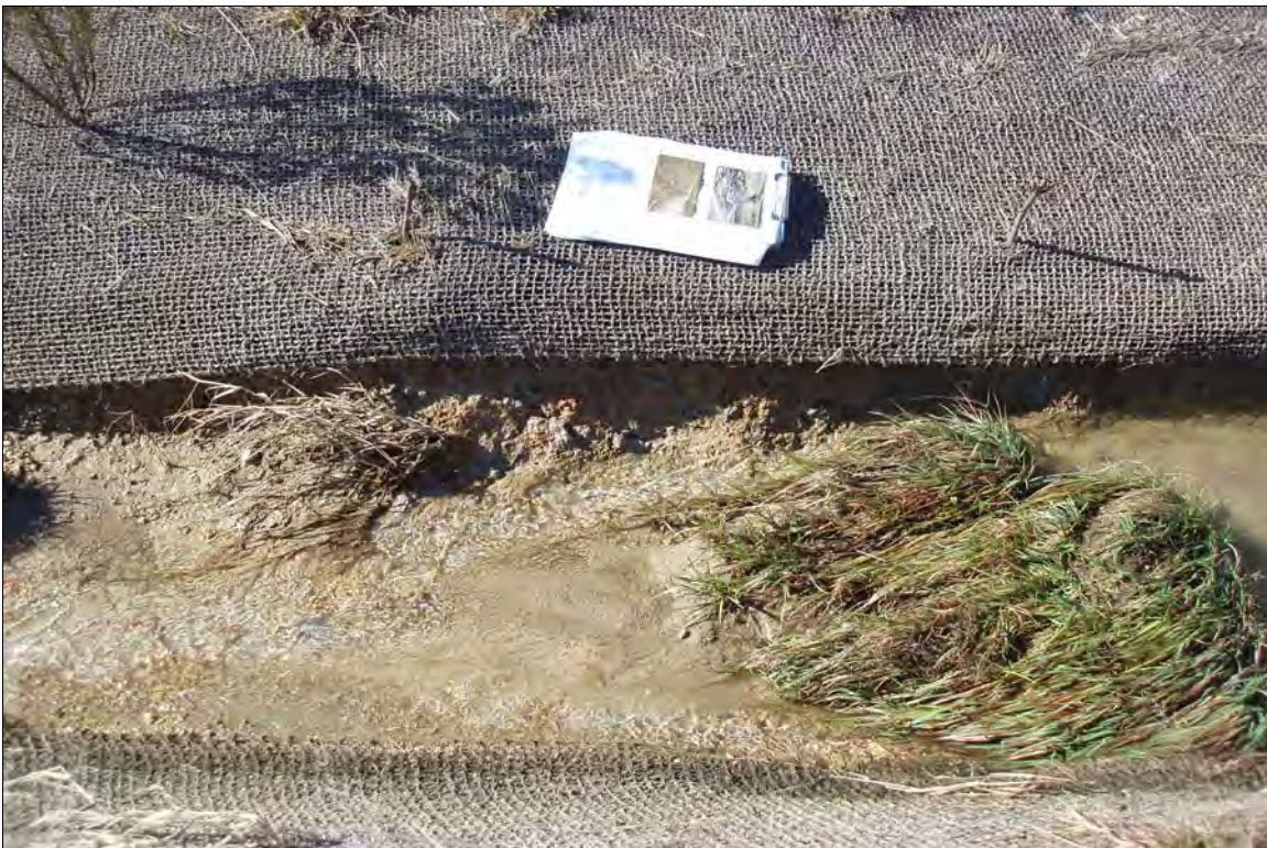
SP2 – Bed degradation near Station 33+40. 11/19/08 – MY-01
