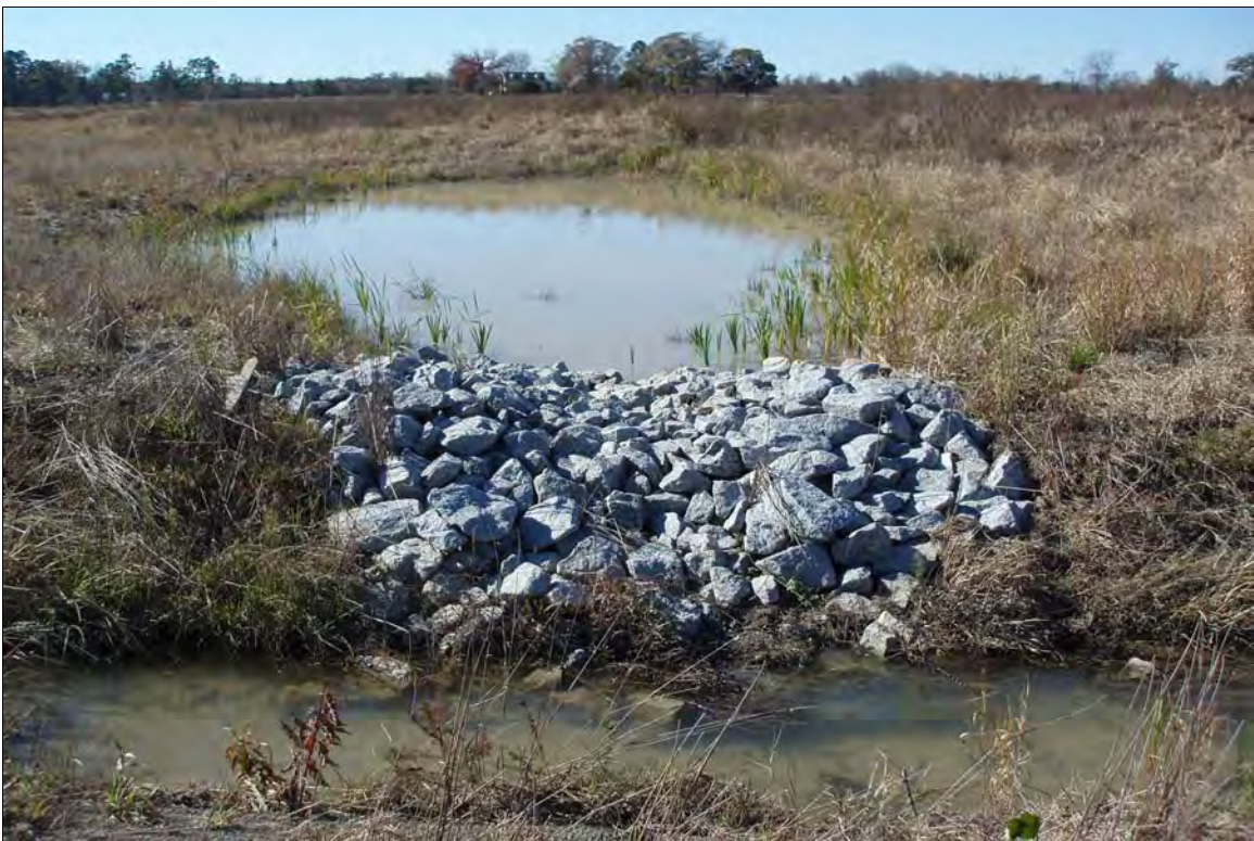
Photo Point S9: View of water quality treatment structure near Station 41+75. 11/19/08 – MY-01
