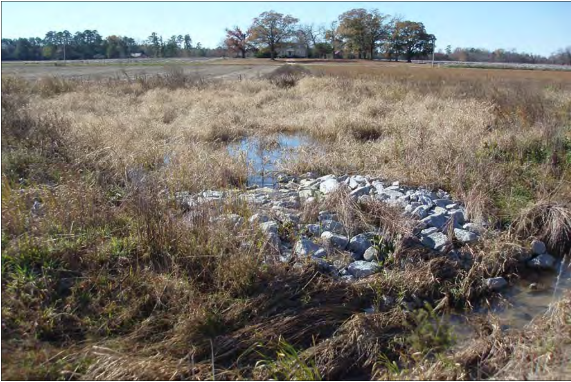
Photo Point S4: View of water quality treatment structure near Station 32+25. 11/19/08 – MY-01
