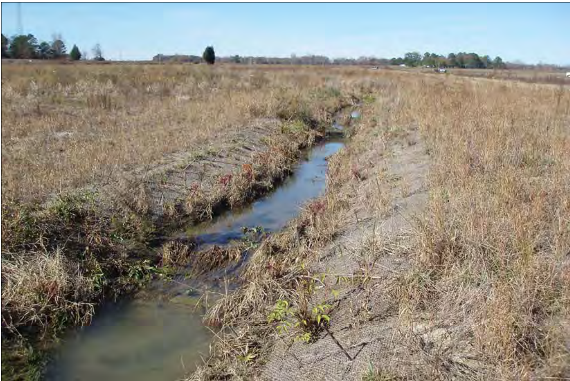
Photo Point S5: View looking at log drop structures, near Station 33+35. 11/19/08 – MY-01
