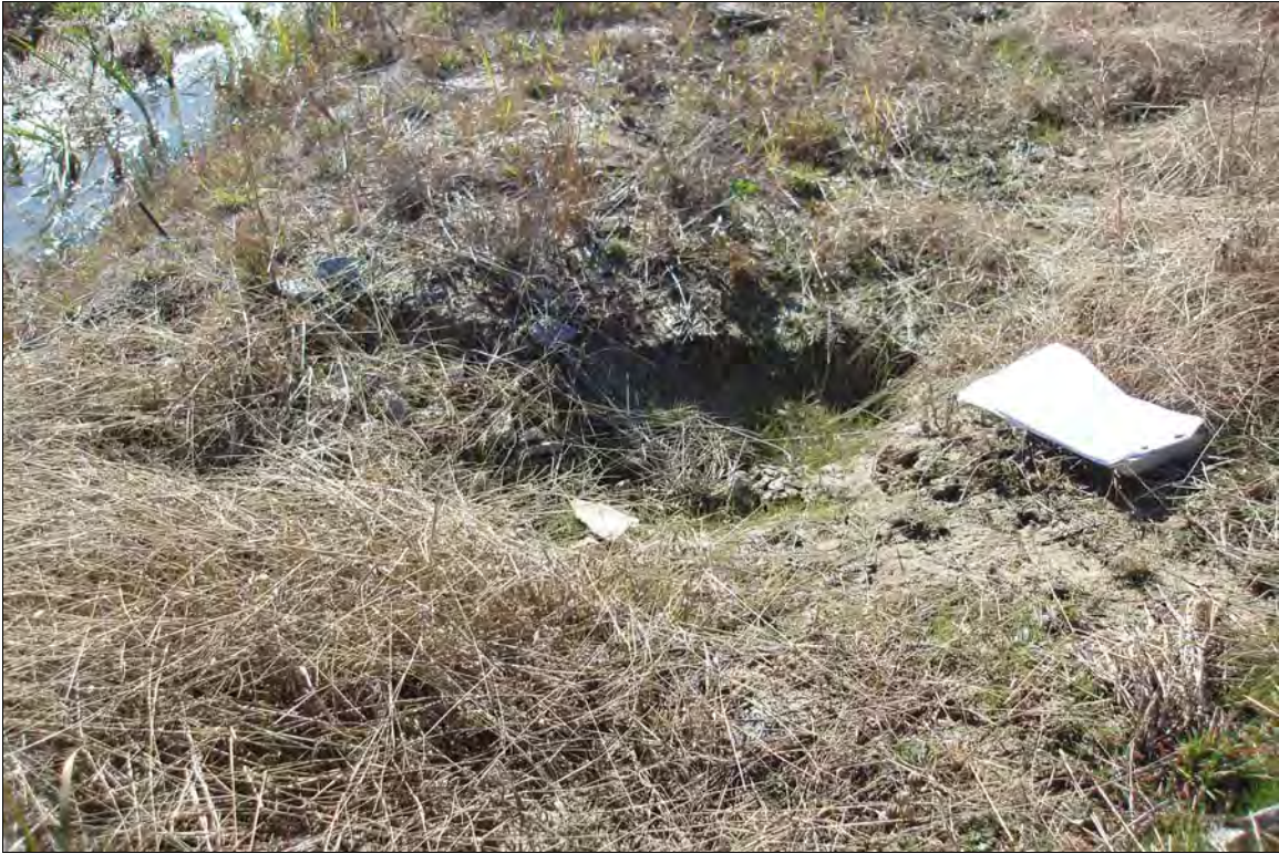
SP3 – Floodplain erosion near Station 43+95. 11/19/08 – MY-01
