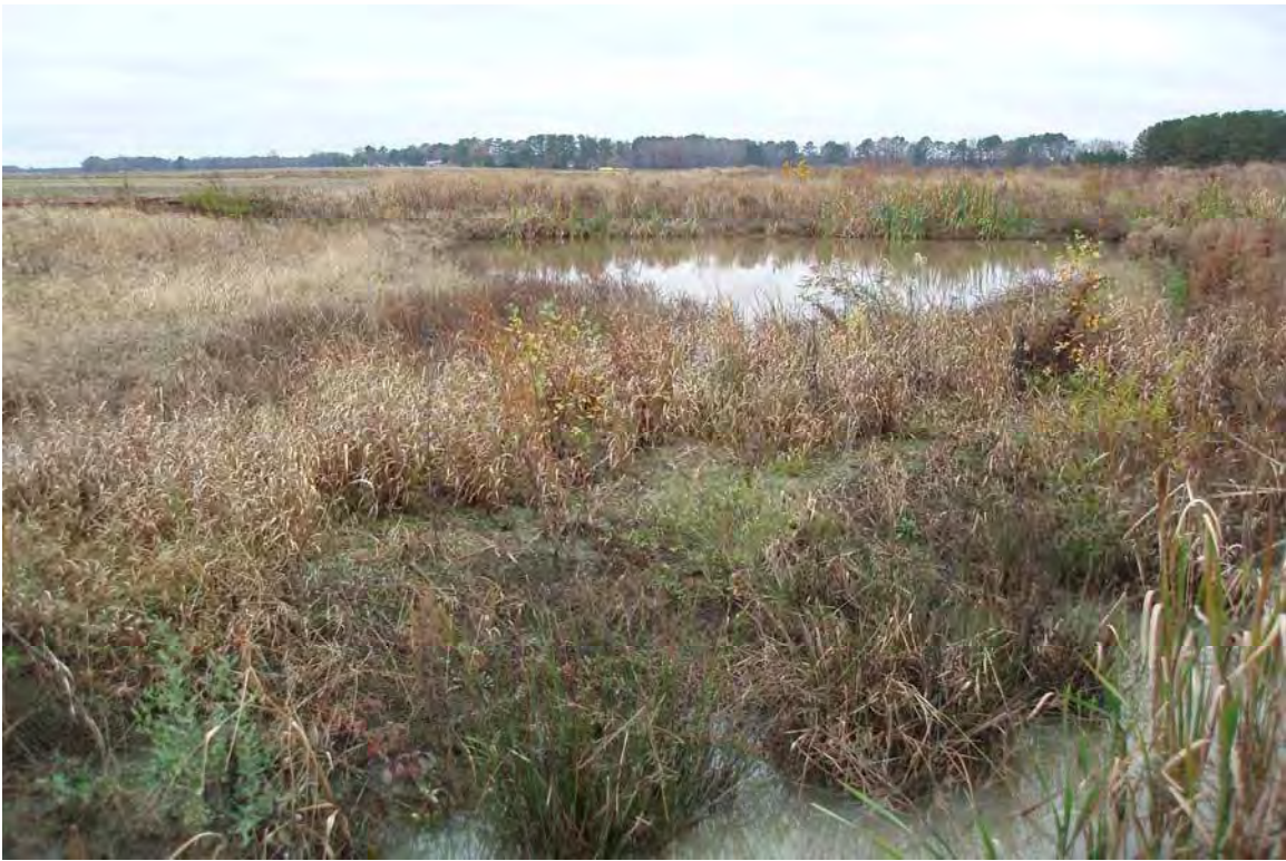
Photo Point S14: View of stream with water quality treatment structure in the background near Station 62+60. 11/24/09 – MY-02
