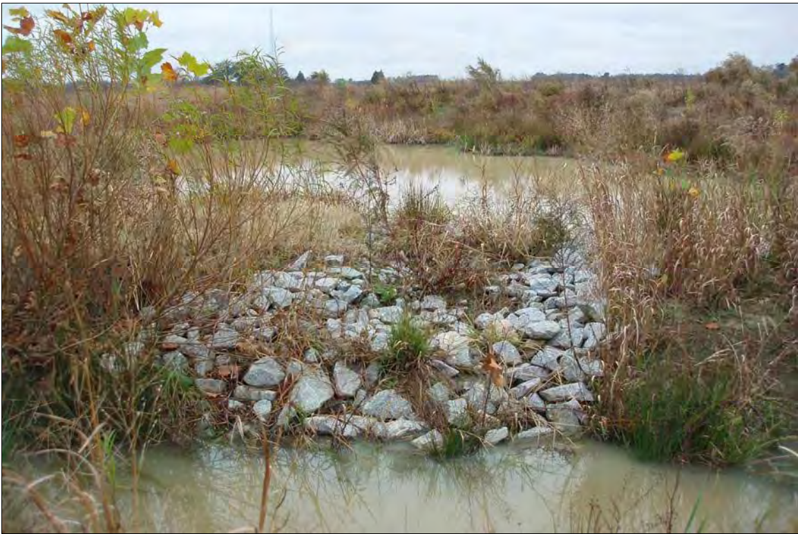
Photo Point S11: View of water quality treatment structure near Station 47+00. 11/24/09 – MY-02
