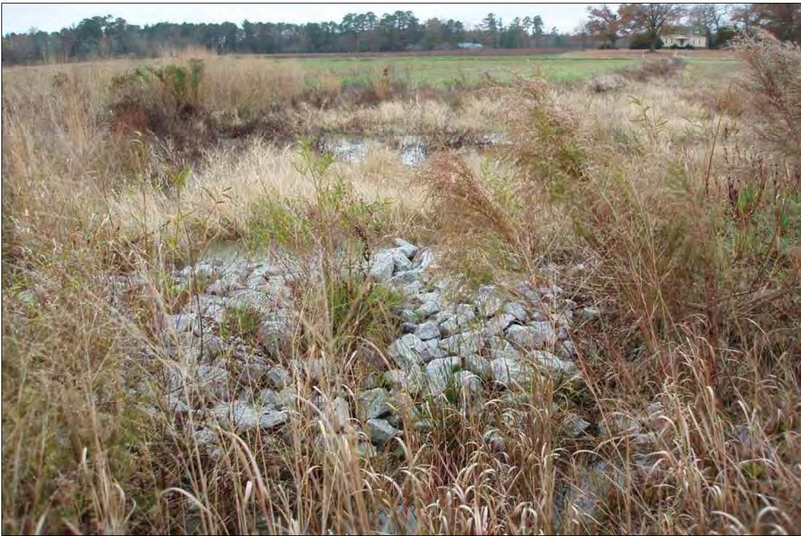
Photo Point S4: View of water quality treatment structure near Station 32+25. 11/24/09 – MY-02
