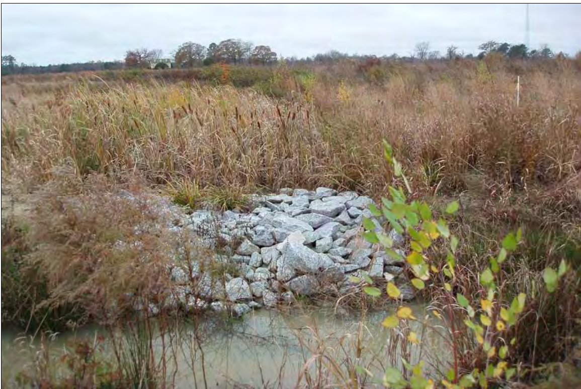
Photo Point S9: View of water quality treatment structure near Station 41+75. 11/24/09 – MY-02
