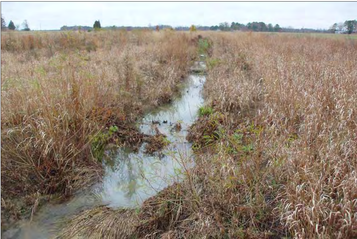
Photo Point S5: View looking at log drop structures, near Station 33+35. 11/24/09 – MY-02
