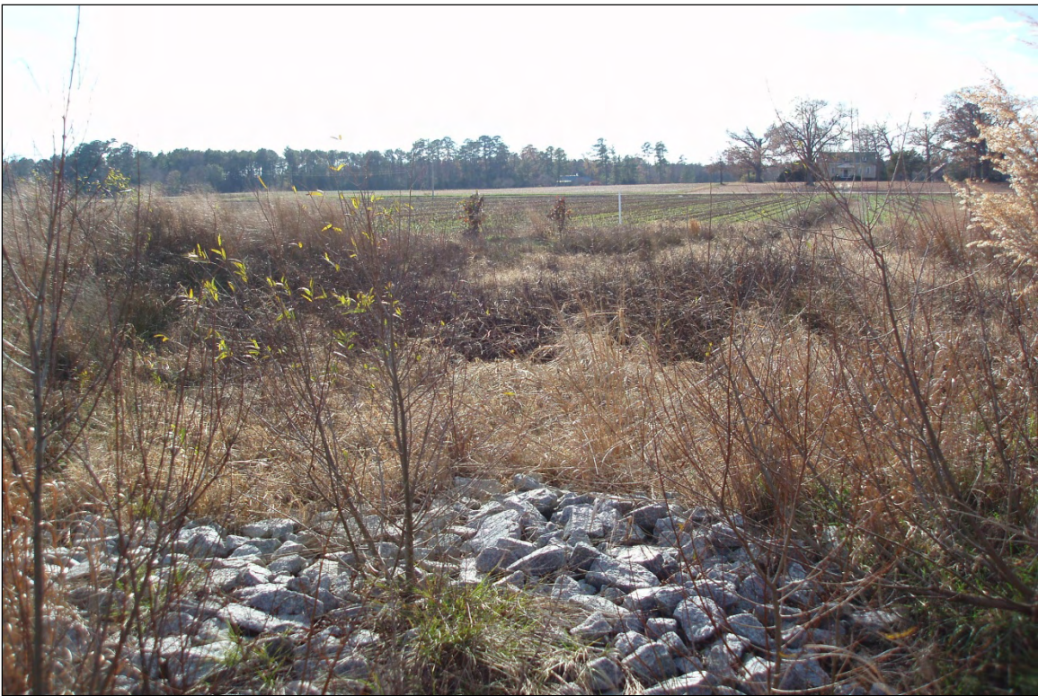
Photo Point S4: View of water quality treatment structure near Station 32+25. 12/6/10 – MY-03
