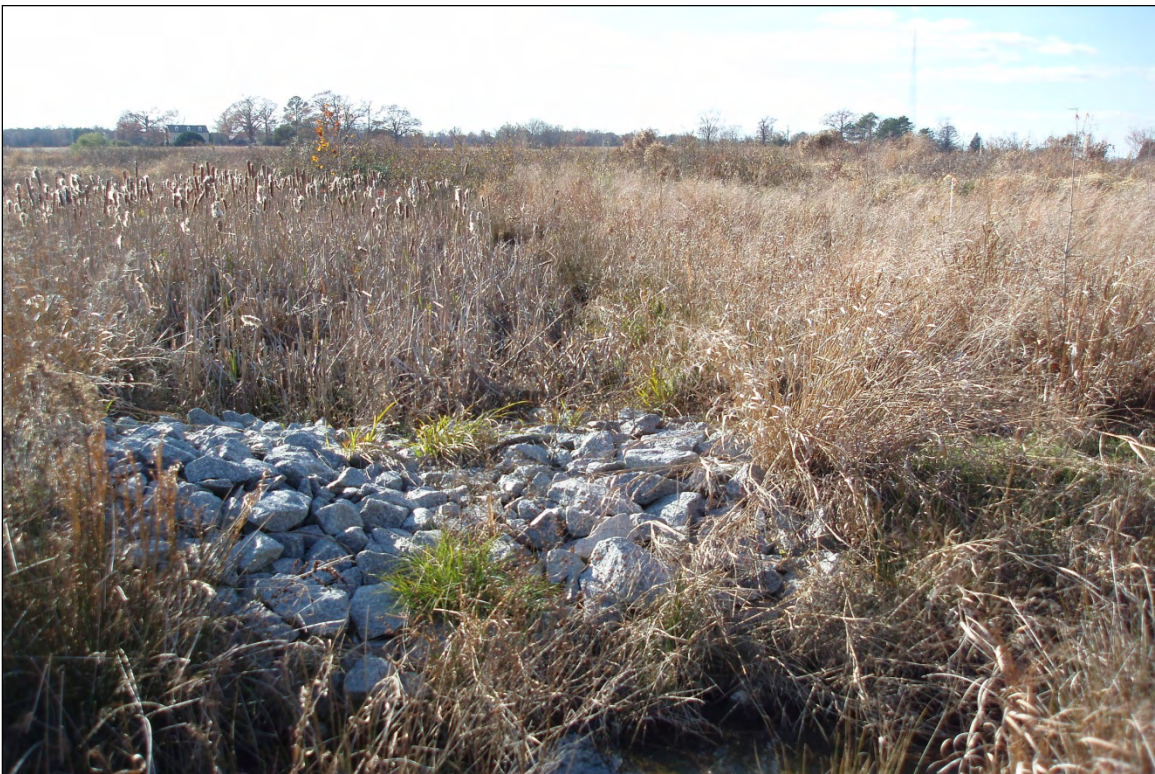
Photo Point S9: View of water quality treatment structure near Station 41+75. 12/6/10 – MY-03
