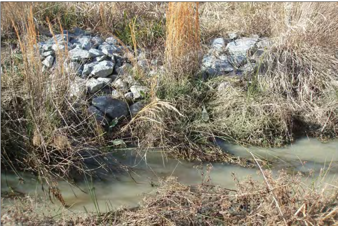
Photo Point S9: View of water quality treatment structure near Station 41+75. 1/12/12 – MY-04
