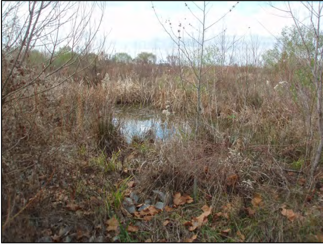
Photo Point S11: View of water quality treatment structure near Station 47+00. 12/18/12 – MY-05
