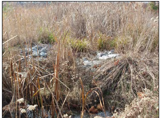
Photo Point S9: View of water quality treatment structure near Station 41+75. 12/18/12 – MY-05
