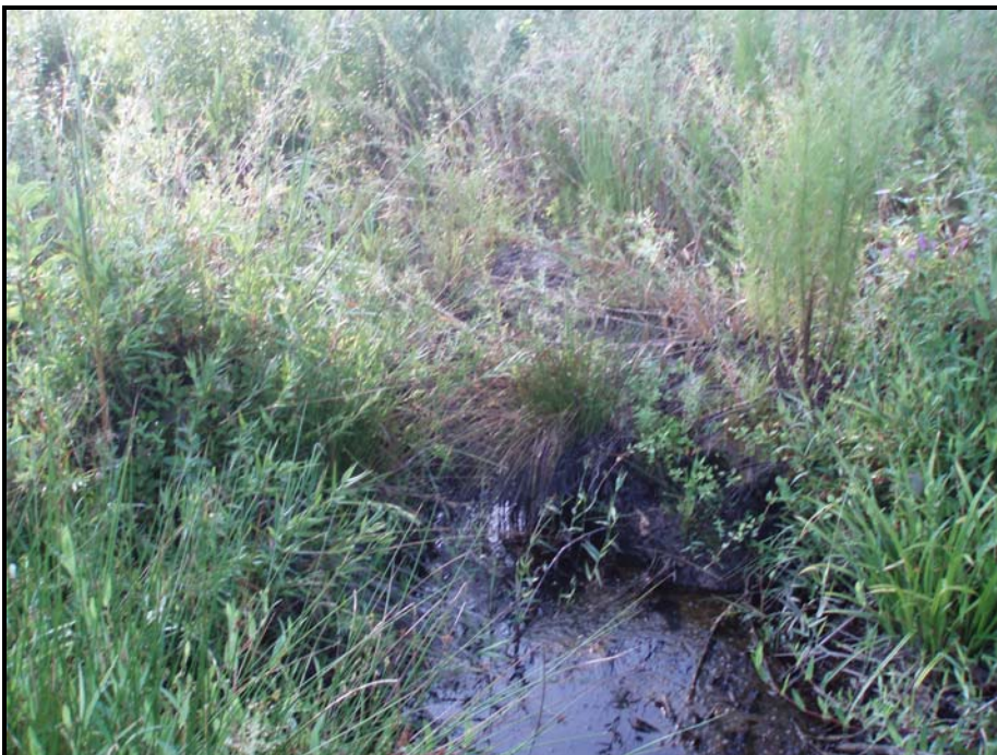
12+00 UT-3 US. Left bank ditch plug washed out
