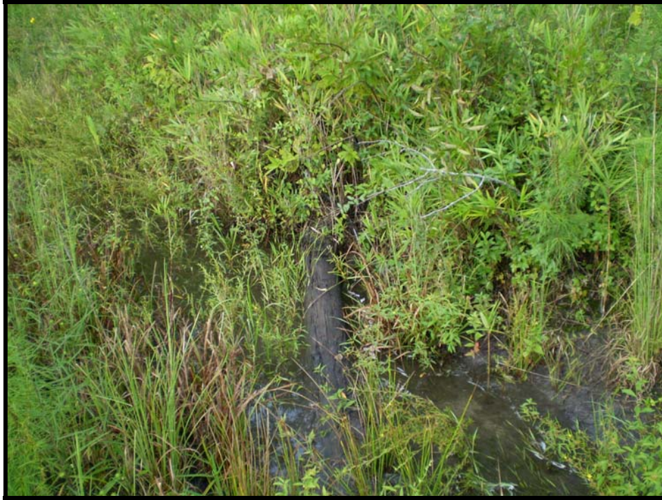
SPA 3. UT1-B Sta. 68+85 Log vane undercutting
