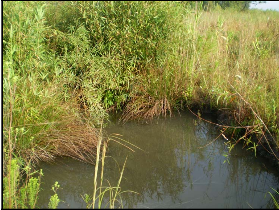
SPA 7. UT2 Sta. 16+75 Erosion on both banks at log weir
