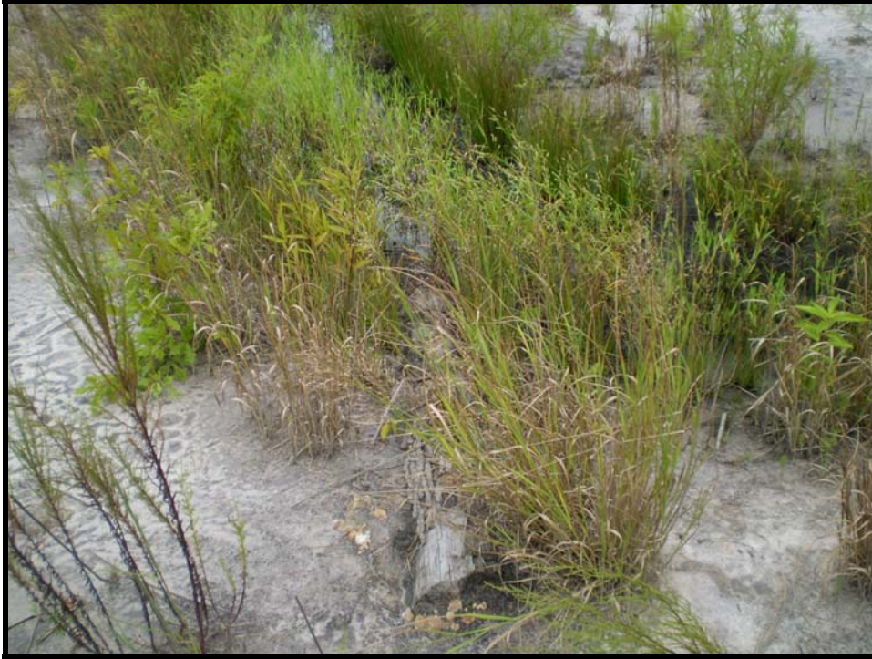
SPA 5. UT2 Sta.33+00 Log vane exposed on top of right bank
