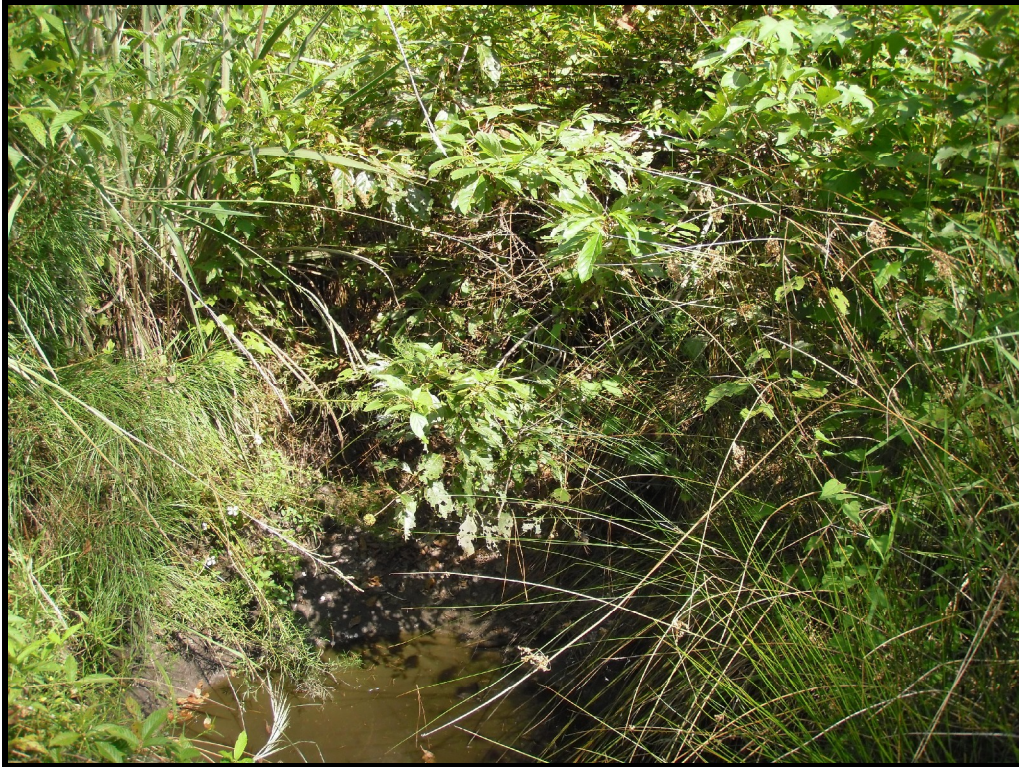
ID #1 – Beaver dam, STA 10+50
