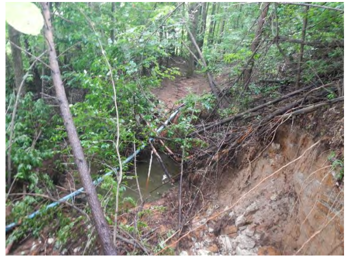
Eroding spillway below Pond 2 (8/22/2013)
