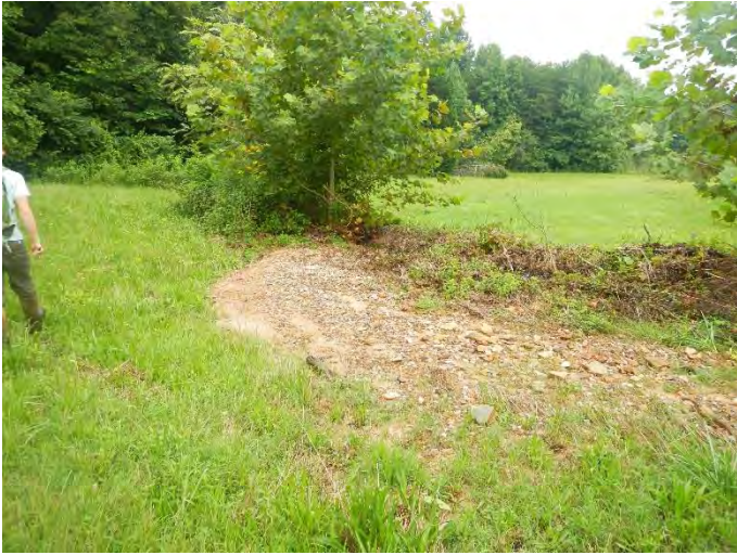
Sediment deposition along UT1 A (8/22/2013)
