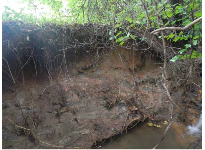
Bank scour along UT1 above Pond 2 (8/22/2013)
