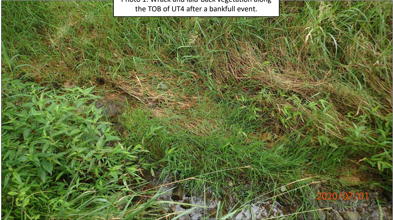
Photo 2: Wrack and laid-back vegetation along the TOB of UT1 after a bankfull event.
