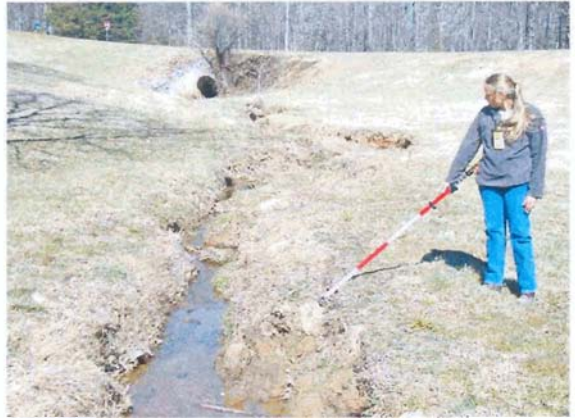
Bank Erosion - Downstream
