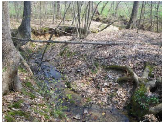
UT1 looking downstream from station 10+00; bank erosion at confluence with Hogan Creek; March 8, 2011
