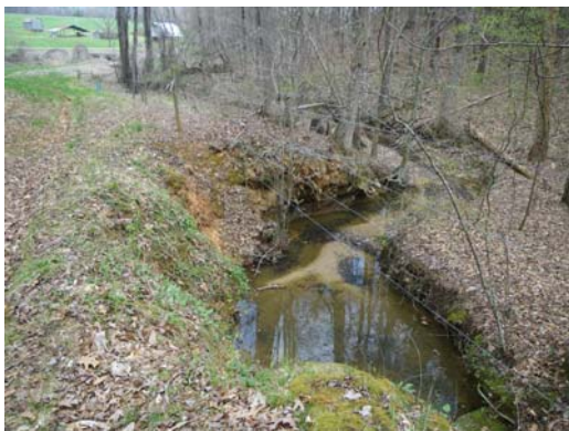
UT2, looking downstream from station 10+50; bank erosion threatening farm road on left; April 8, 2011
