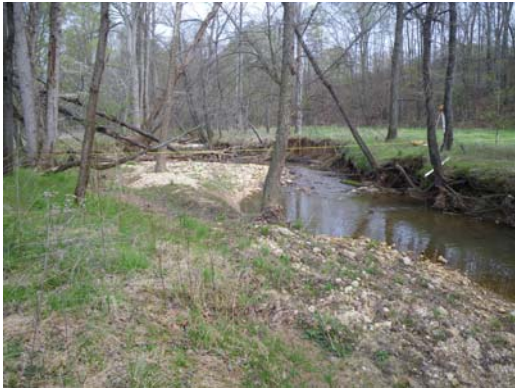
Hogan Creek looking downstream from station 35+00; bank erosion and mid-channel deposition; April 8, 2011
