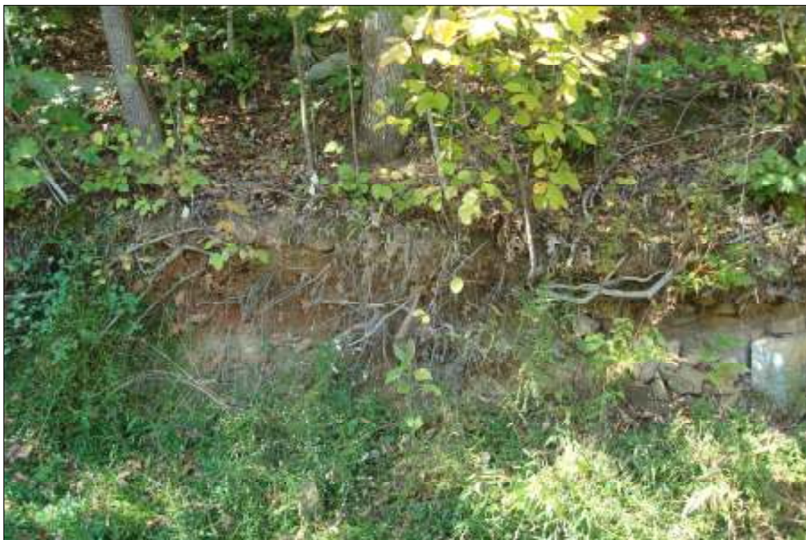
Buckhorn Creek, minor scour , Sta 187+70 9/26/11 Photo No. 50
