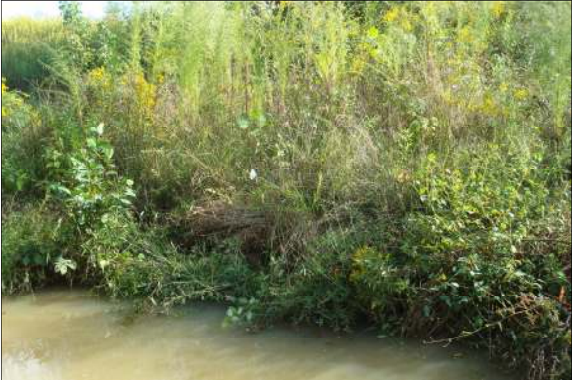
Buckhorn Creek, minor bank scour , Sta 152+90 9/26/11 Photo No. 48
