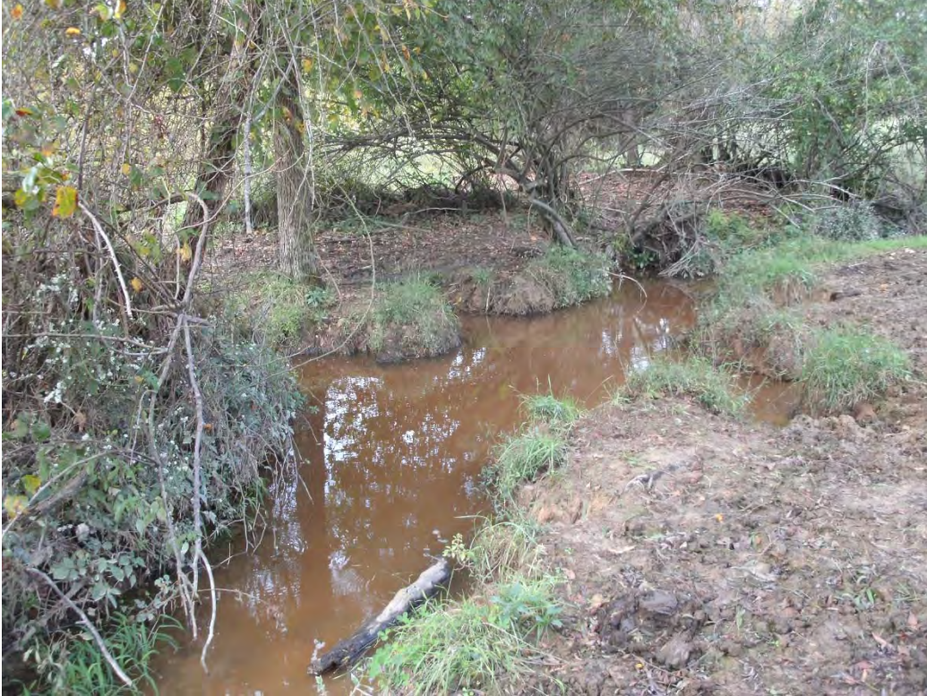
Photo 5. Damage to UT1 due to cattle
