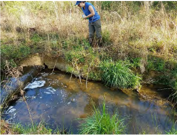
Before - Localized Erosion (4/7/2020)
