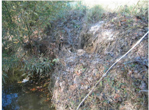
Issue Photo 5 station XX+XX. Bank slump
