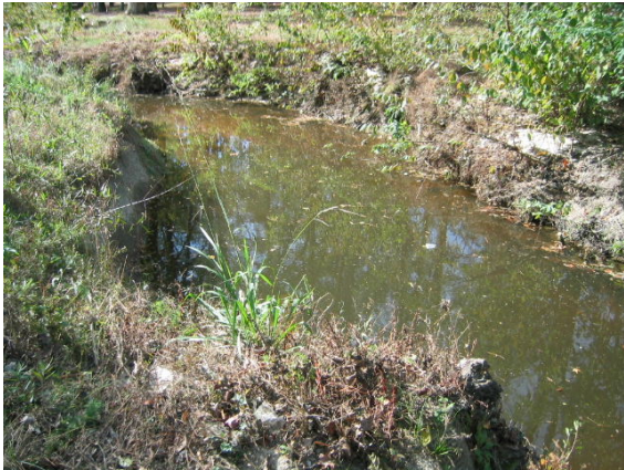
Issue Photo 4 station XX+XX. Overland flow resulting in bank erosion.
