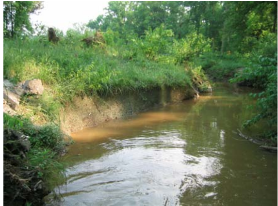
Issue Photo 5 station 6+50. Bank slump
