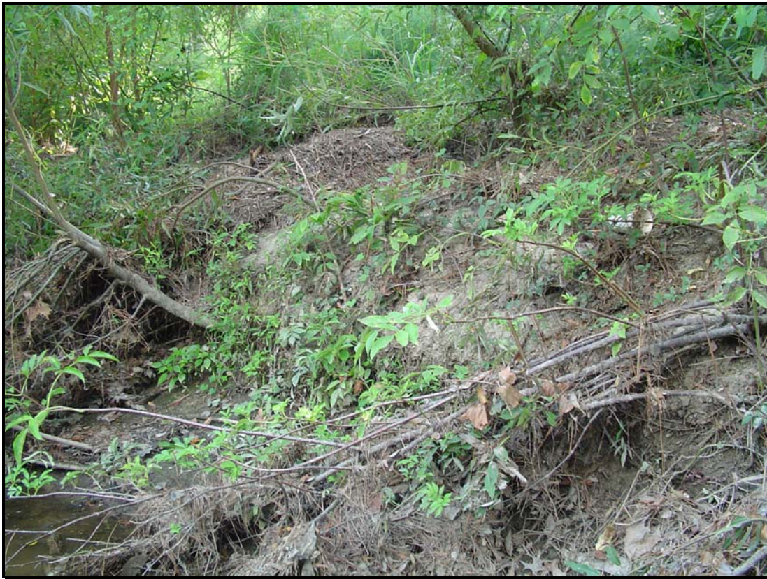
P63. Station 2+60. Erosion on right bank.
