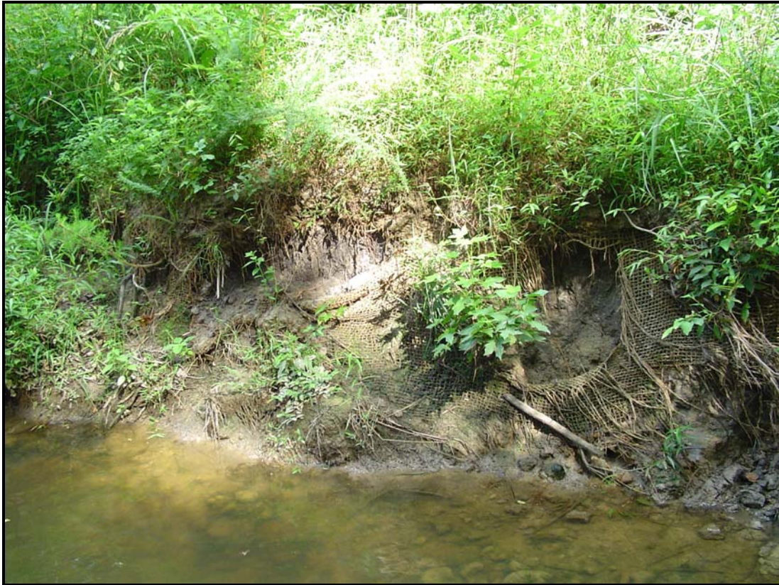
P48. Station 6+25. Erosion on right bank.
