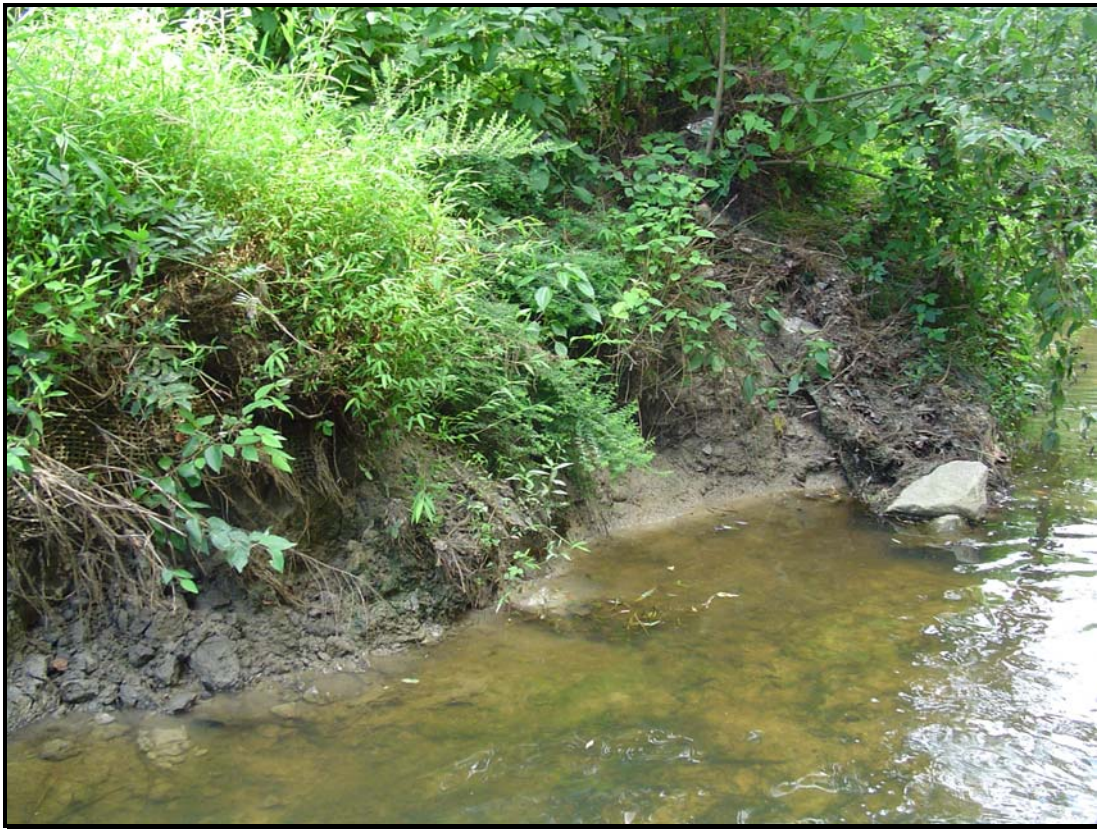
P49. Station 6+25. Erosion on right bank.
