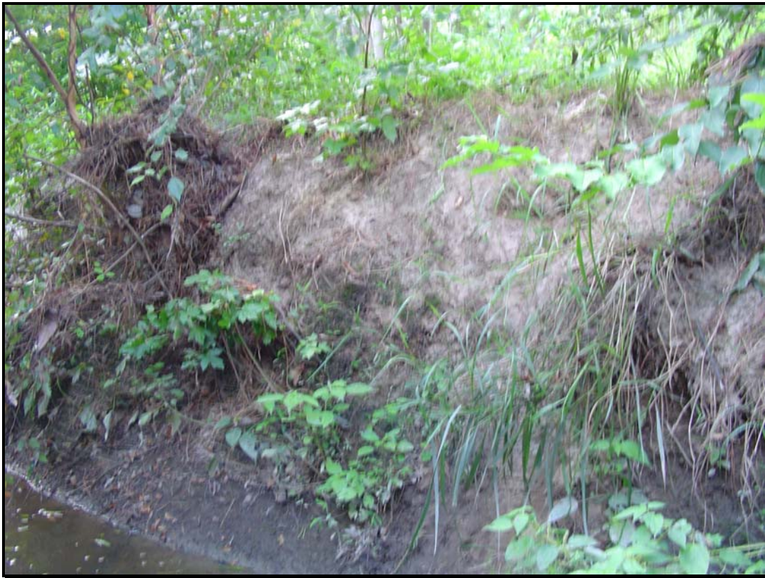
P57. Station 4+10. Erosion on right bank.
