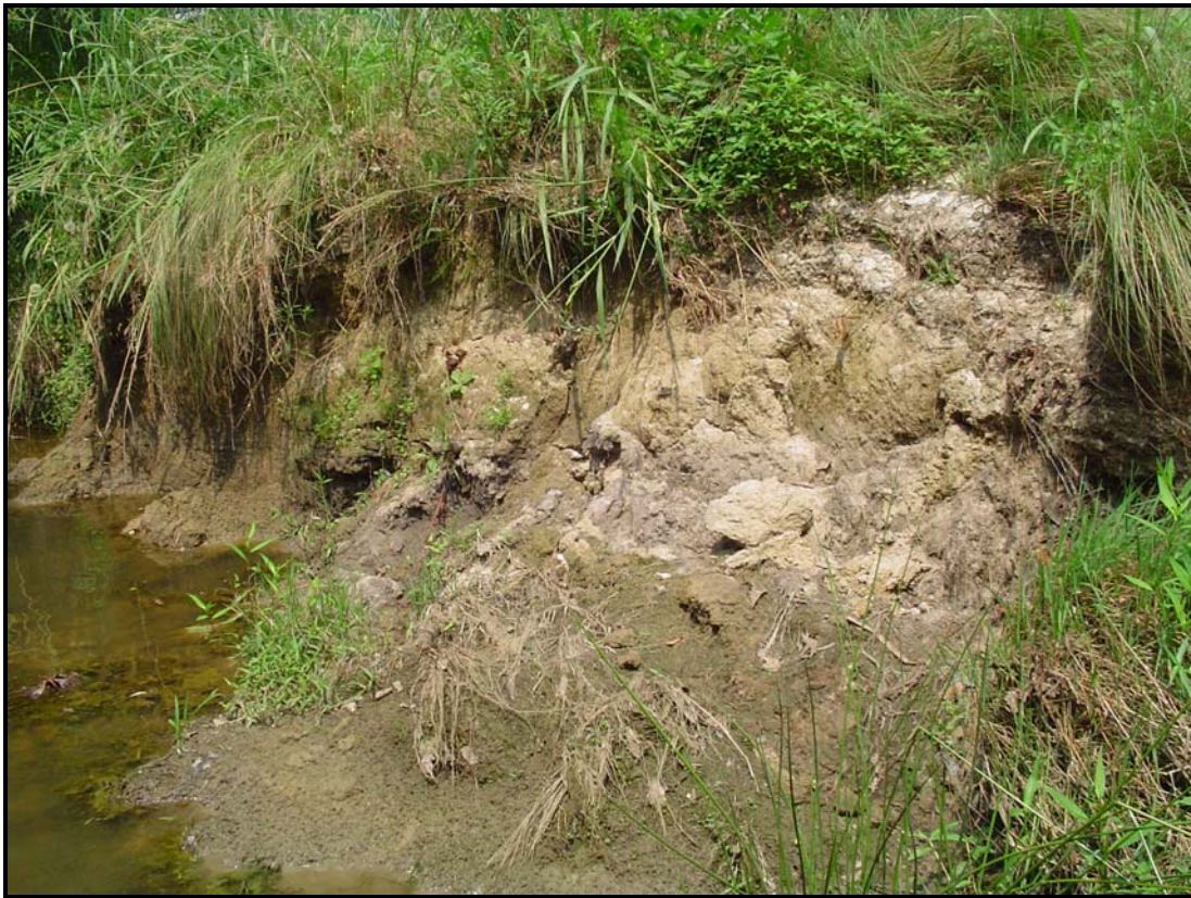
P22. Station 15+30. Erosion on left bank
