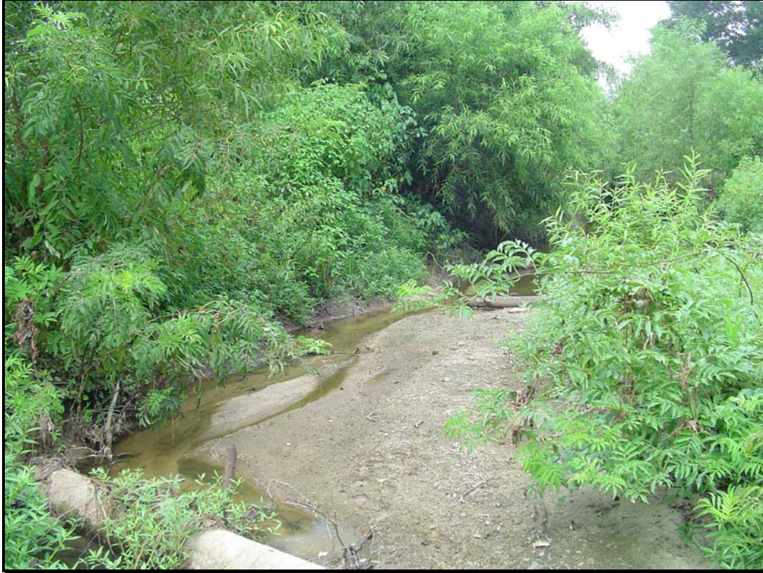
P3. Station 21+30. Aggregation.
