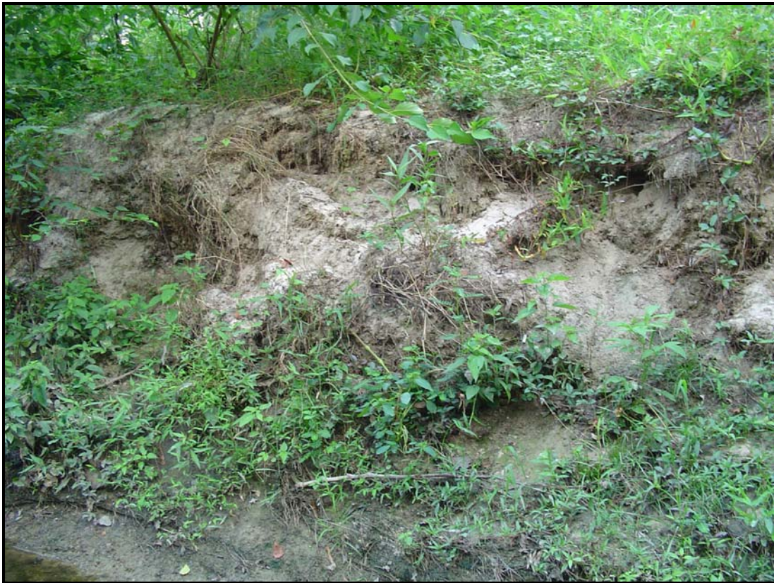
P61. Station 2+65. Erosion on left bank.
