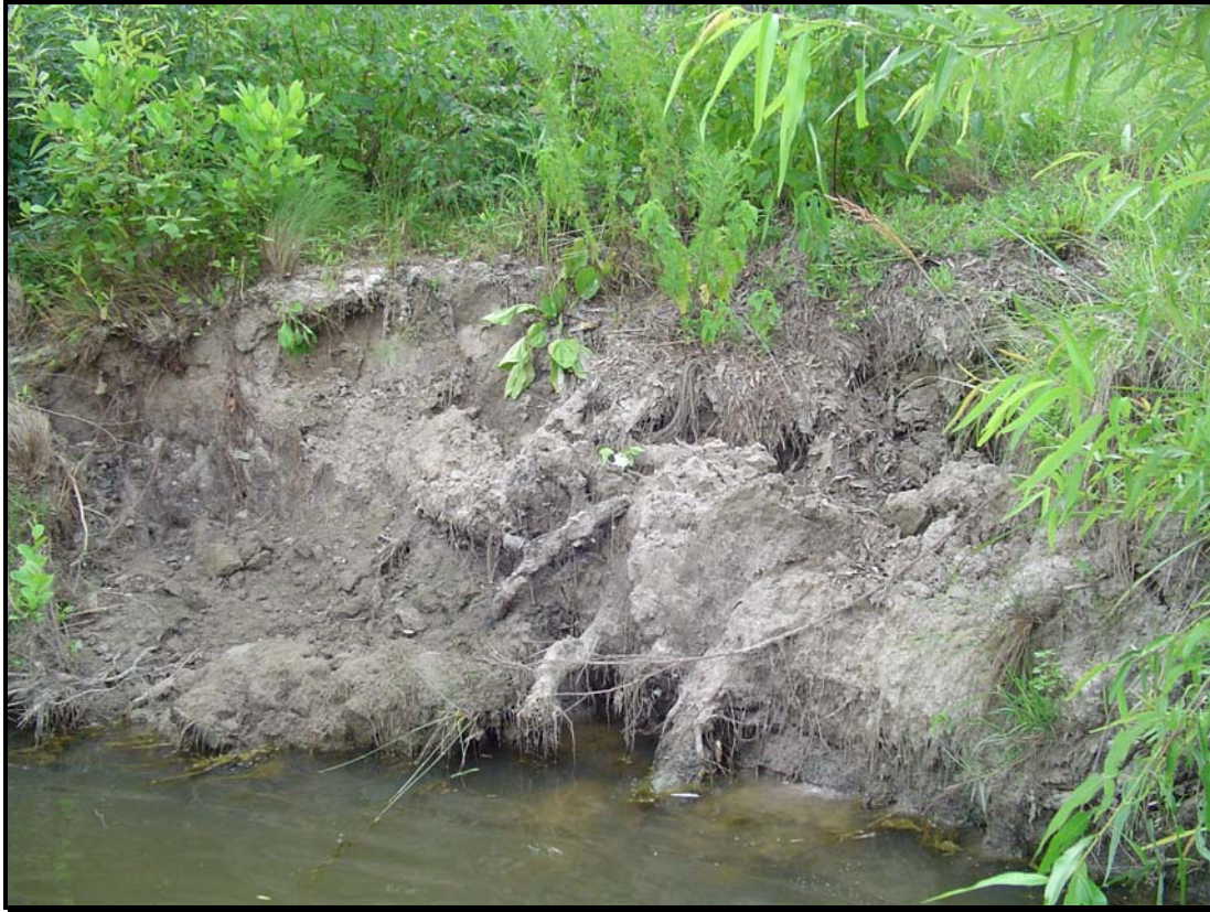
P20. Station 15+70. Erosion on left bank.
