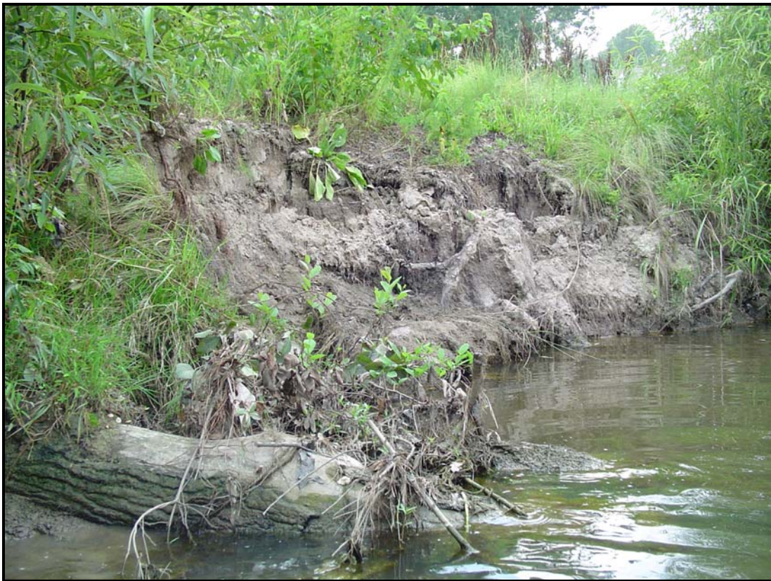
P19. Station 15+80. Erosion on right bank looking upstream.
