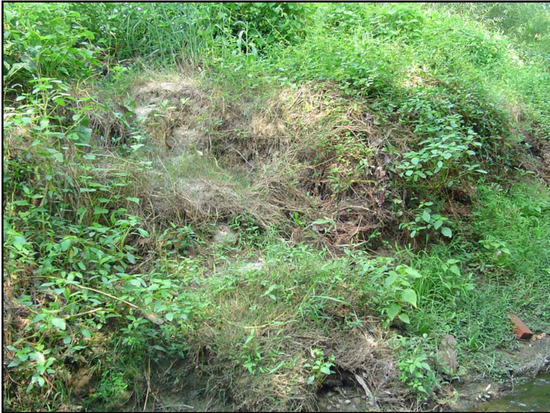
P67. Station 1+20. Erosion on right bank.
