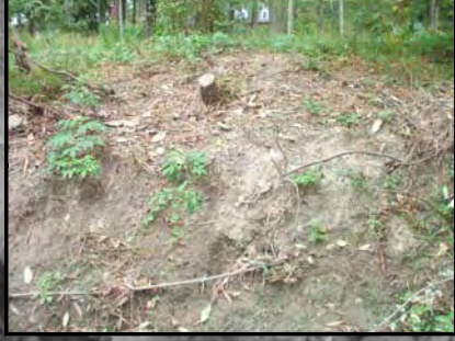
P42 - Right Bank Erosion
