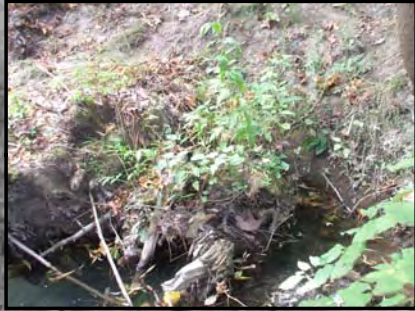
P28 - Right Bank Erosion
