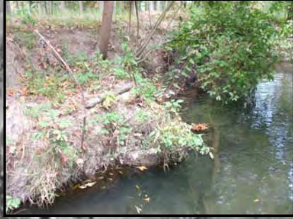
P27 - Right Bank Erosion
