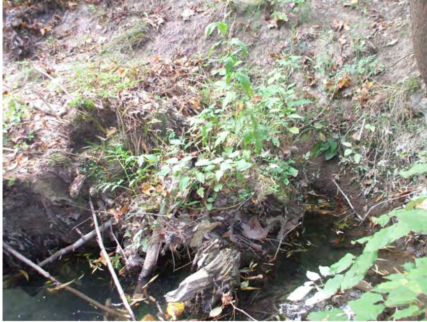
P28 – Sta. 7+90, left bank erosion, 10/22/07
