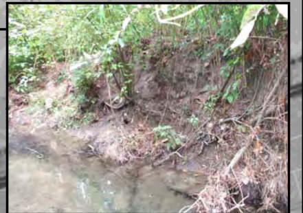
P24 - Left Bank Erosion
