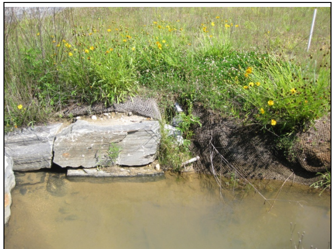
SPA4 – SFHC Reach 2 Scour around vane arm
