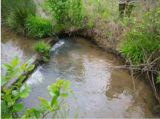
SPA1-1 – SFHC Reach 1 Left bank scour
