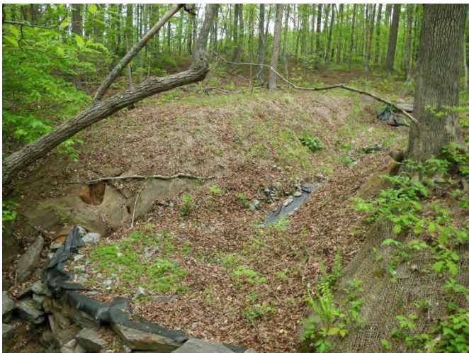
SPA1-6 – Ephemeral drainage channel bed erosion
