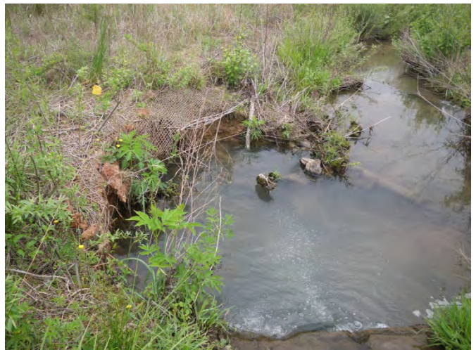
SPA2-1 – SFHC Reach 1 Rootwad failure along left bank due to undercutting along bank
