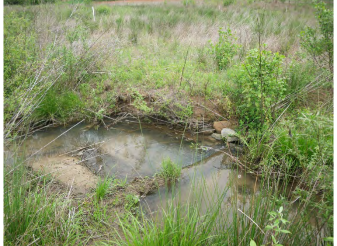
SPA1-2 – SFHC Reach 1 Right bank scour
