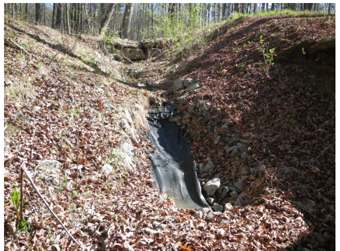
SPA1-6 – Ephemeral drainage channel bed erosion
