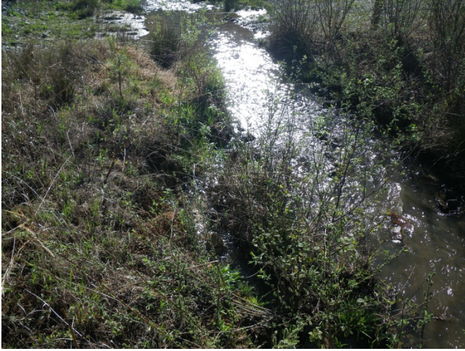
SPA2-3 – SFHC Reach 2 Left bank scour
