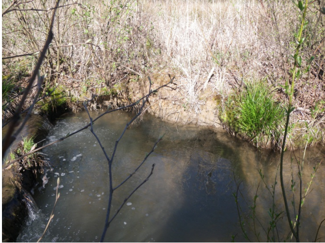
SPA1-1 – SFHC Reach 1 Left bank scour
