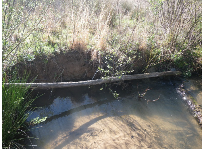
SPA1-2 – SFHC Reach 1 Right bank scour
