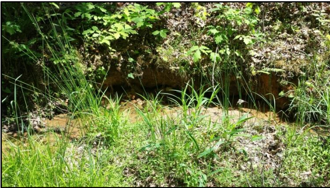
SPA4-3 – UT2 Reach A: Small area of erosion along the left bank.
