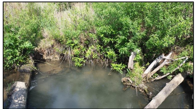
SPA4-2– SFHC Reach 2: Rootwad failure along left bank due to undercutting along bank.
