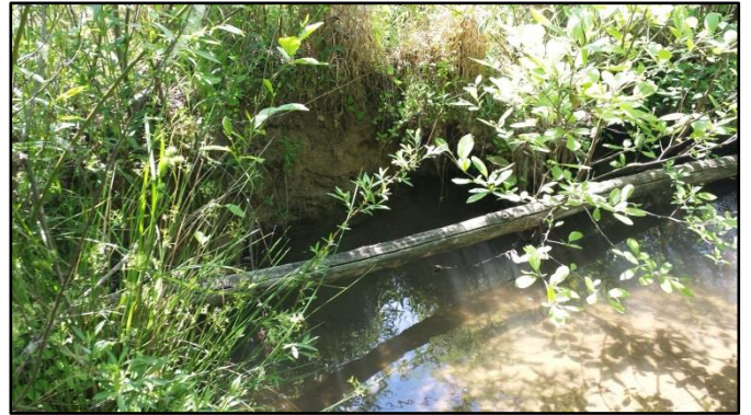
SPA1-2 – SFHC Reach 1: Right bank scour.
