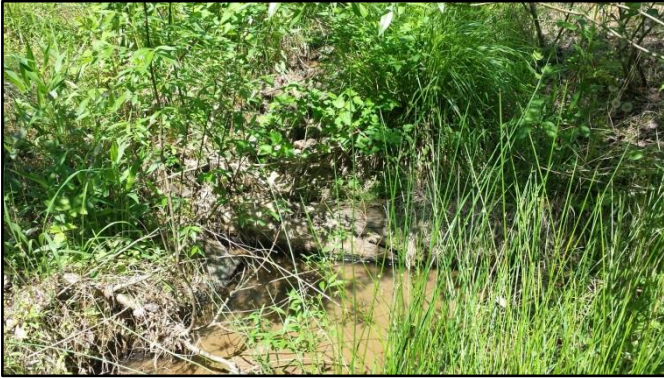
SPA1-5 – UT2 Reach A: Piping within riffle cascade around log sill.
