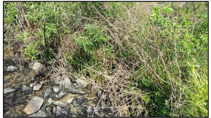
SPA2-3 – SFHC Reach 2: Left bank scour.
