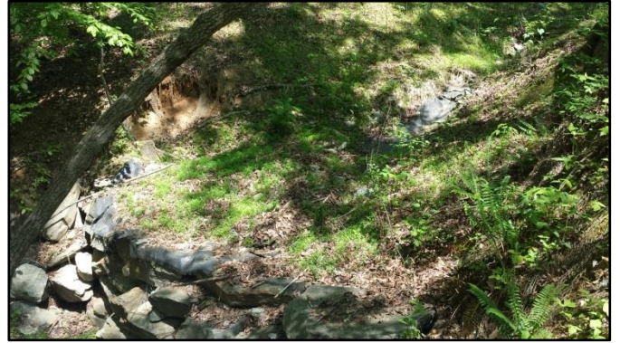
SPA1-6 – UT2: Bed erosion on ephemeral drainage channel.
