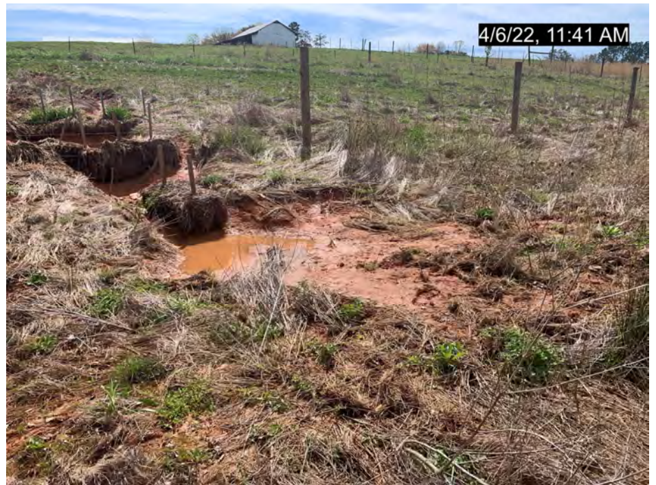
SPA5, R5 Side Slope, Minor deposition and erosion as a result of erosion outside of the easement (MY-03)
