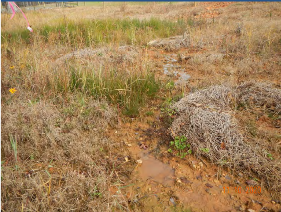
SPA5, R5 Left Floodplain, R5 Side Slope, Minor deposition and erosion as a result of erosion outside of the easement (MY-01)
