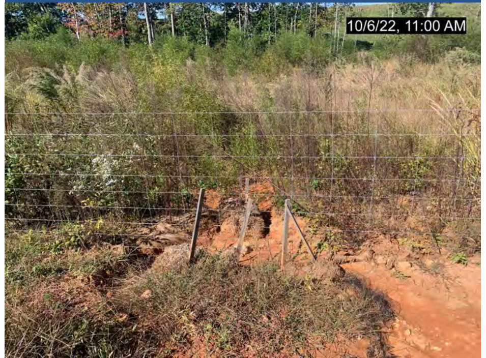
SPA5, R5 Side Slope, Minor deposition and erosion as a result of erosion outside of the easement (MY-03)
