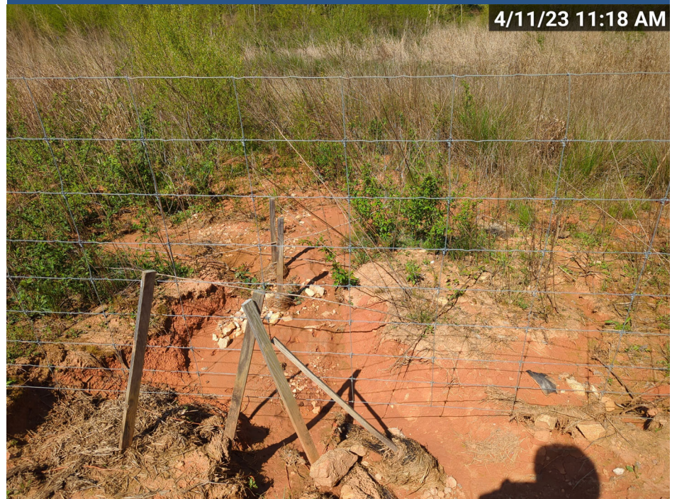
SPA5, R5 Side Slope, Minor deposition and erosion as a result of erosion outside of the easement (MY-04)
