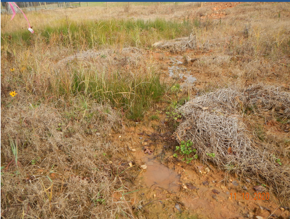
SPA5, R5 Left Floodplain, R5 Side Slope, Minor deposition and erosion as a result of erosion outside of the easement (MY-01)
