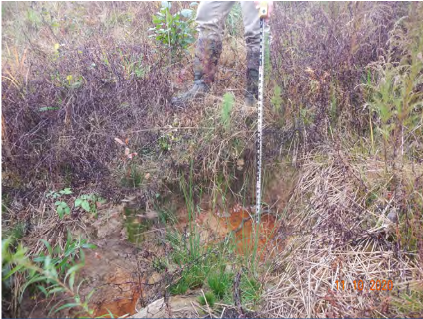
SPA1, R1 Right Floodplain, Minor Slumping (MY-01)
