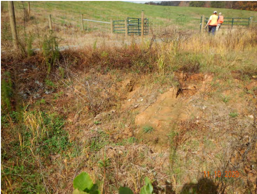
SPA4, R2 Left Floodplain, Minor Erosion (MY-01)
