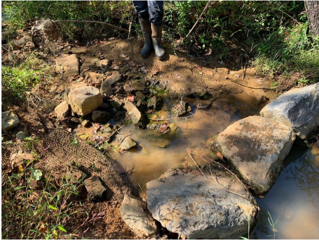
MY1-2 – UT1 Reach 3, station 218+23 – Rock sill piping before repairs (09/27/2022)
