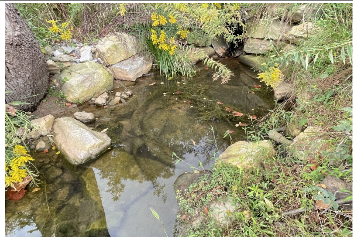
MY2-2 – UT1 Reach 3, station 218+23 – Rock sill piping, perched culvert before repairs (09/26/2023)
