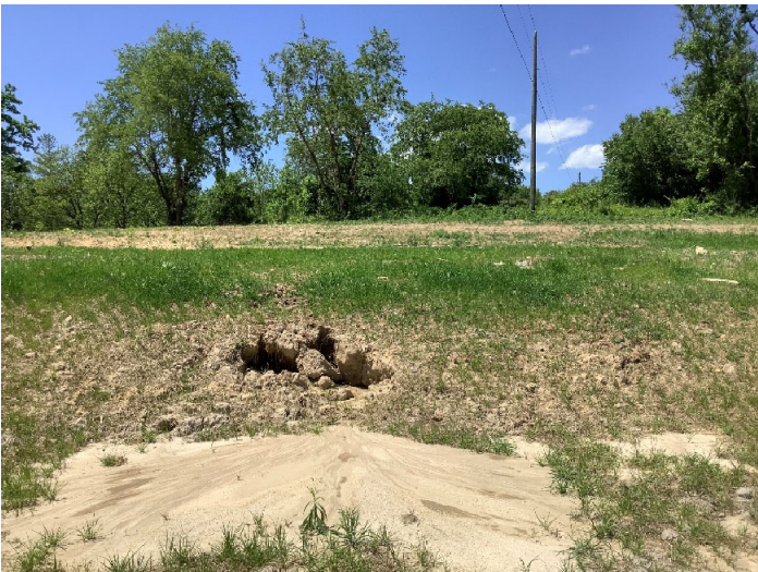
MY0-1 – NL Hunting Reach 1, 102+85 - 103+00 – Floodplain scour before repairs on left bank (05/24/2022)
