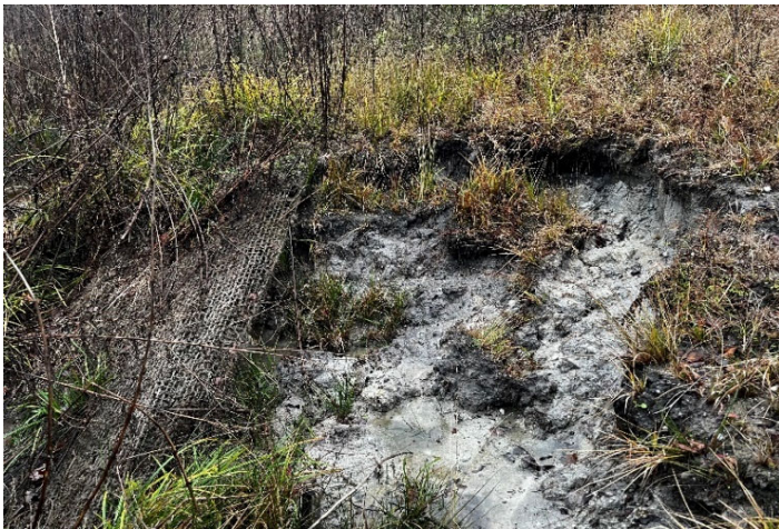
MY1-3 – UT2 Reach 3, station 308+00 to 308+36 – Bank scour before repairs (12/08/2022)
