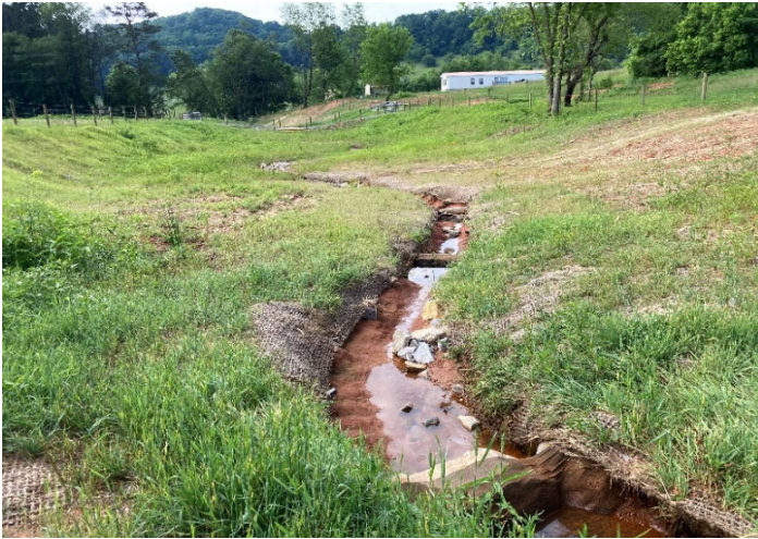
MY0-2 – UT1 Reach 1, station 210+50 to 212+00 – Riffle scour before repairs (06/01/2022)
