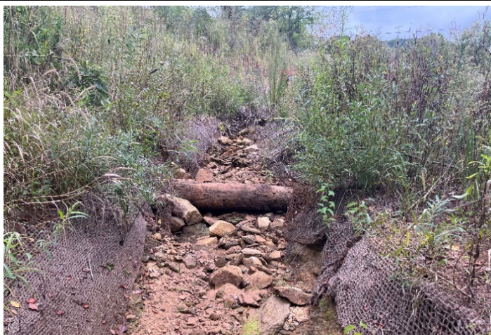
MY2-1 – UT1 Reach 2, station 216+00 to 216+75 – Lack of base flow (09/29/2023)
