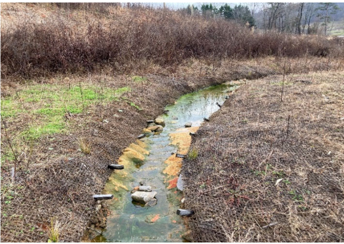
MY1-1 – UT1 Reach 1, station 210+50 to 210+70 – Riffle scour before repairs (12/08/2022)
