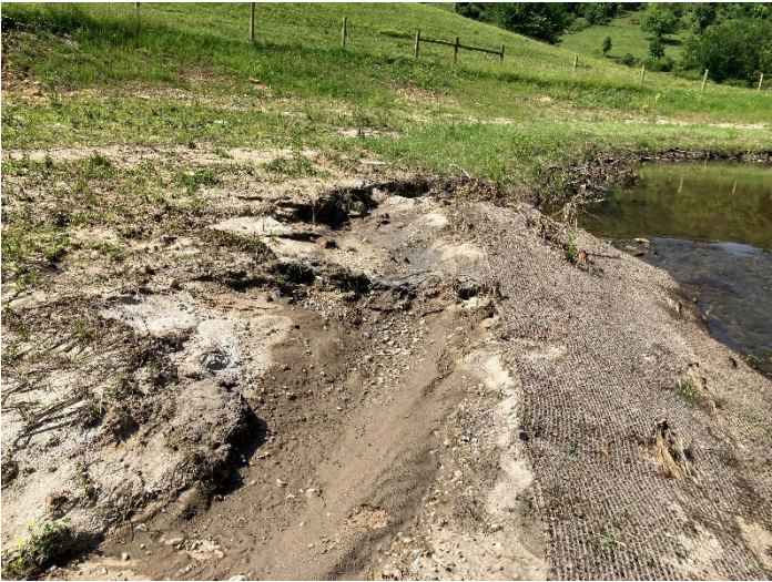
MY0-1 – NL Hunting Reach 1, 102+25 - 102+75 – Right bank scour before repairs (06/01/2022)
