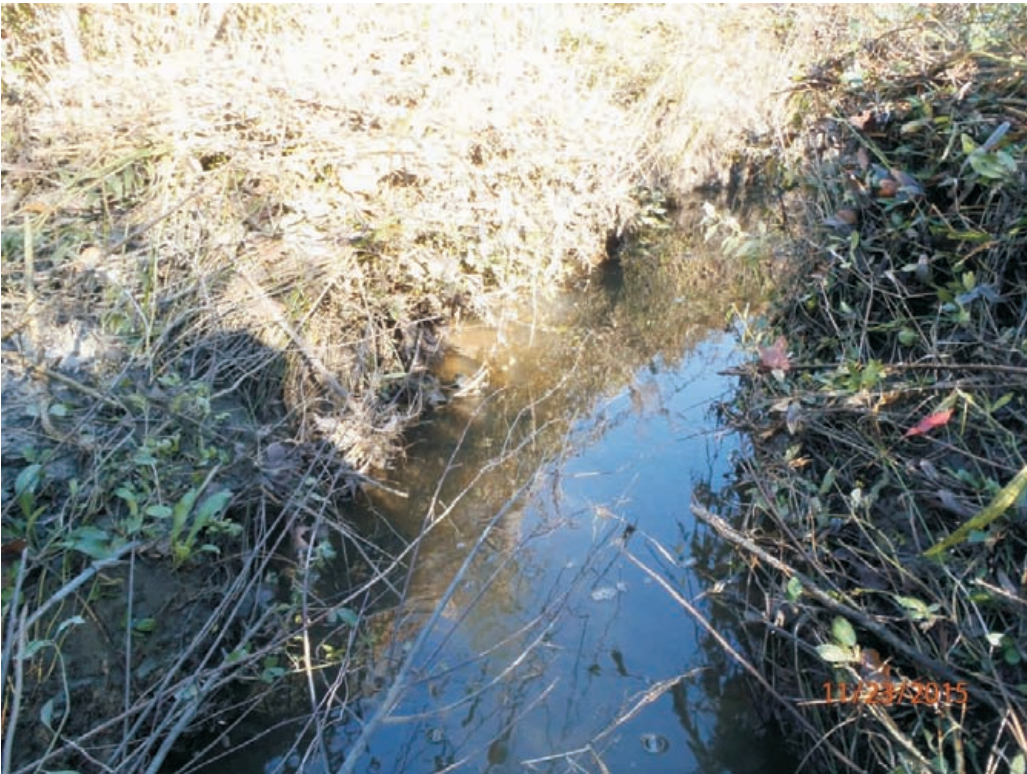
Reach 1A - Stream Problem Area #18; Scour
