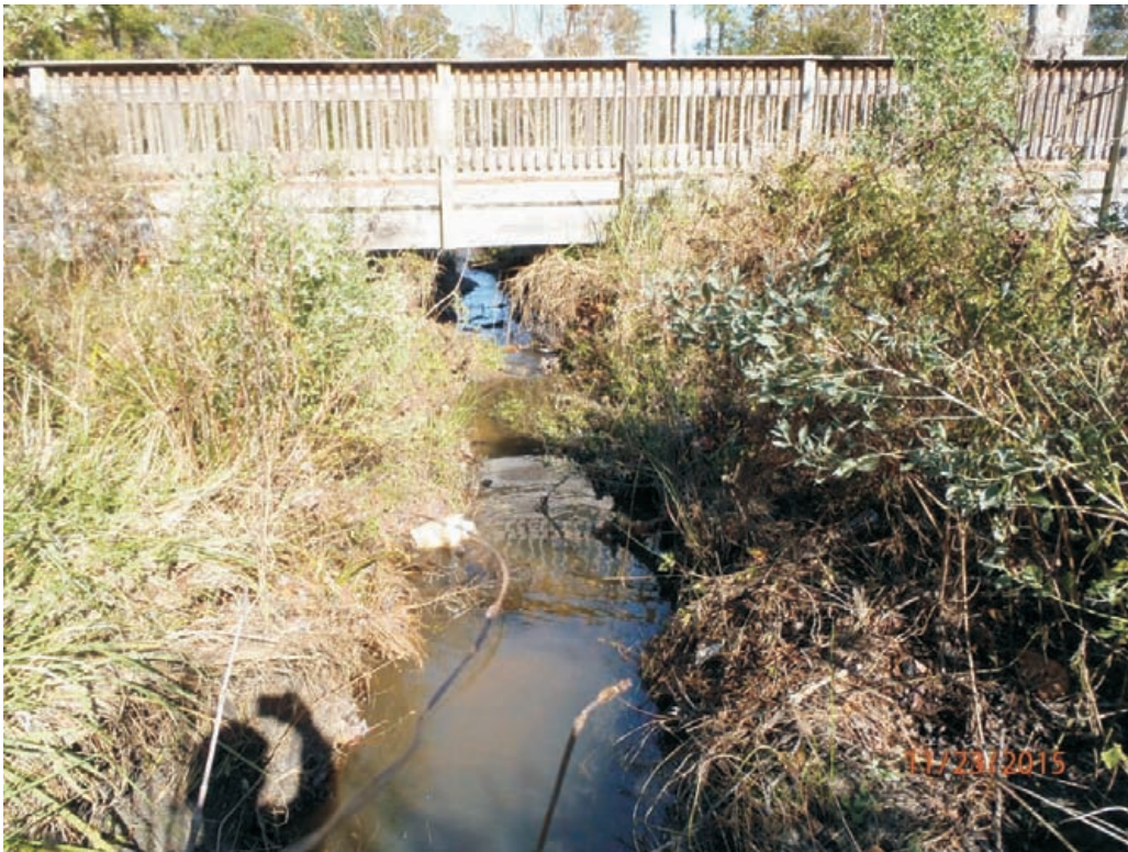
Reach 1A - Stream Problem Area #6; degradation
