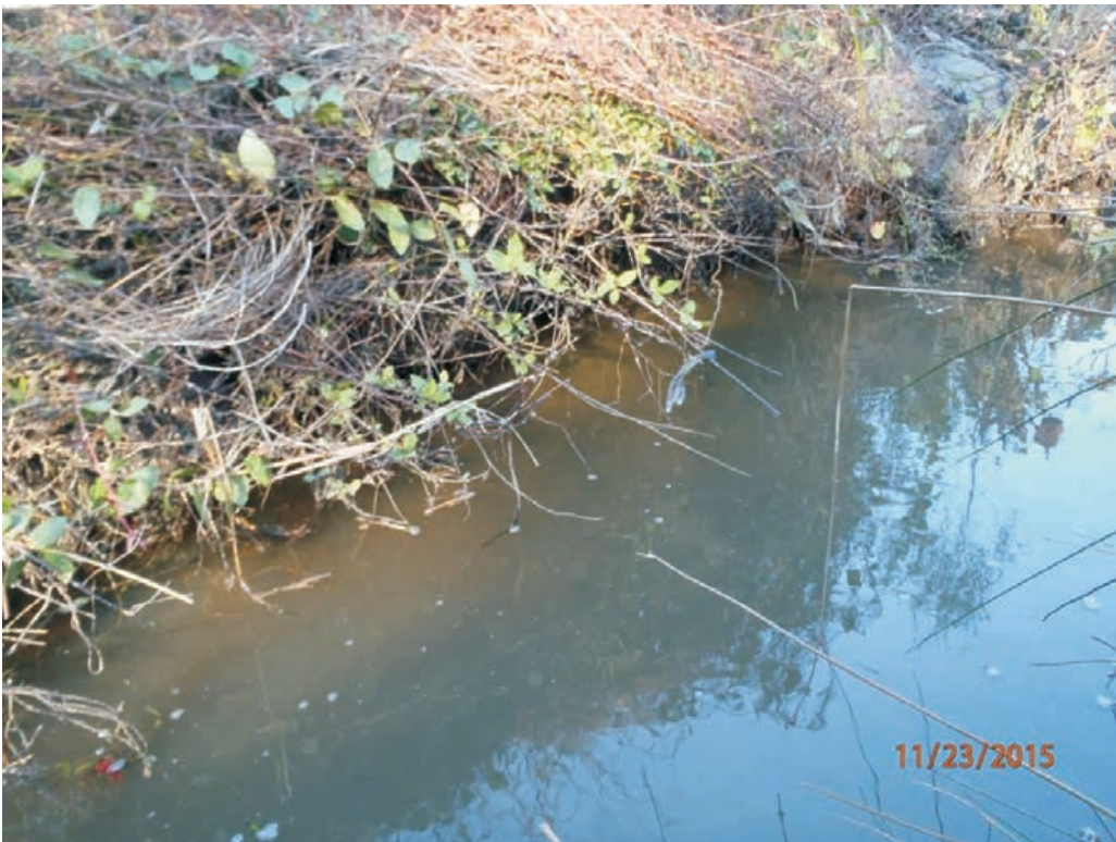
Reach 1A - Stream Problem Area #16; Bank Undercut
