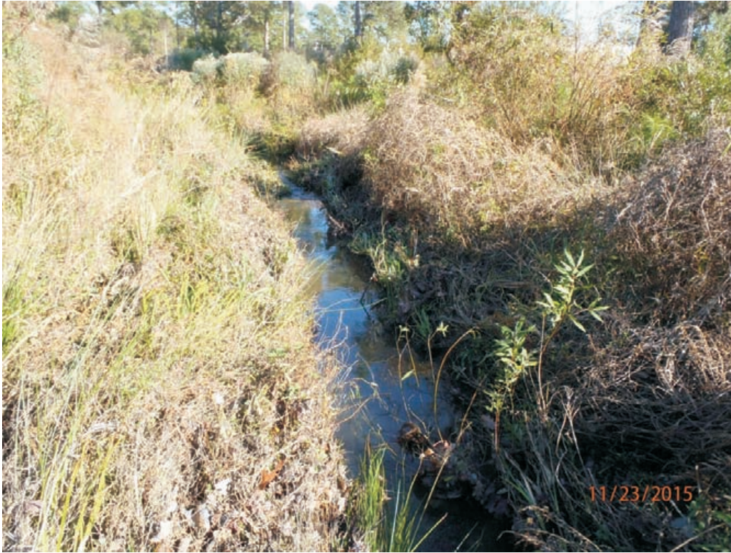
Reach 1A - Stream Problem Area #13; Degradation
