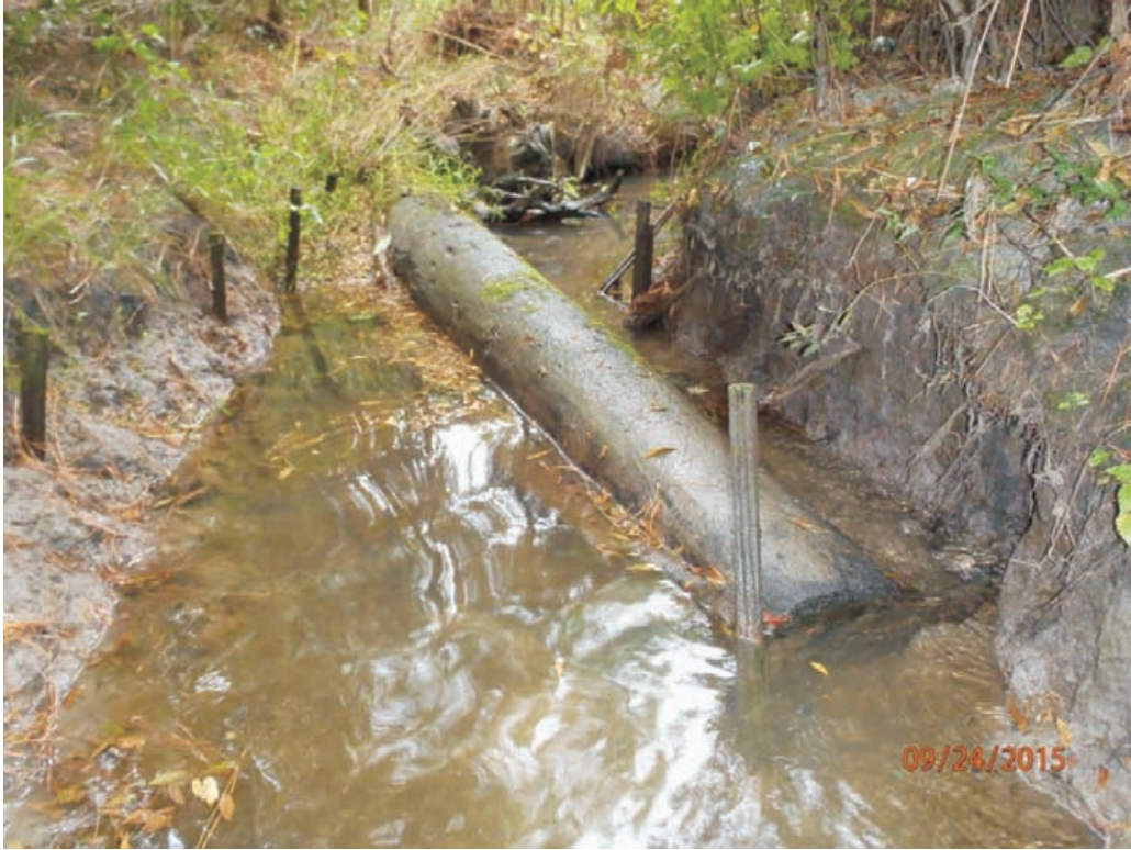
Reach 2A - Stream Problem Area #35; Log Vane Mass Wasting
