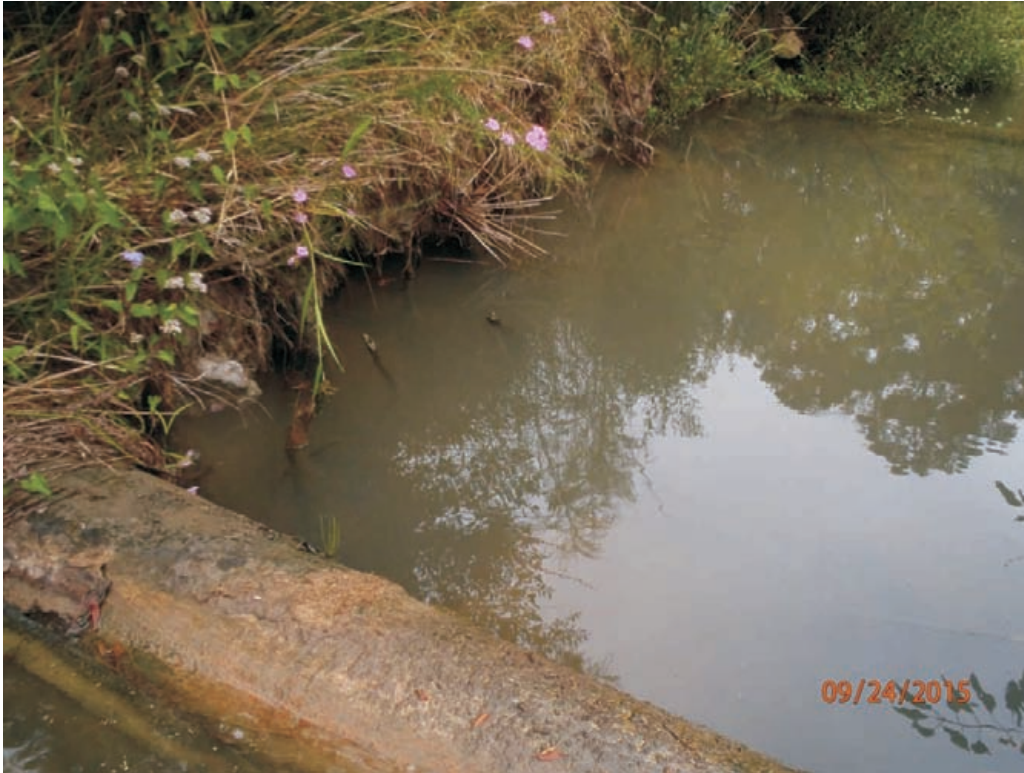
Reach 2A - Stream Problem Area #47; Log Vane Scour
