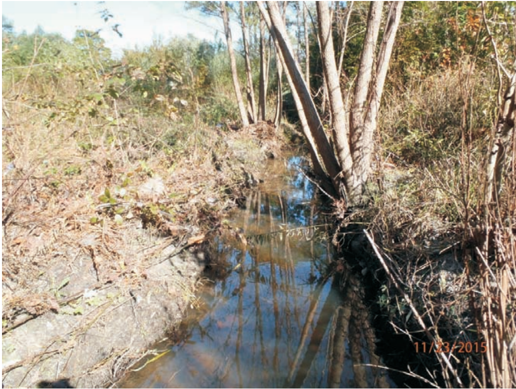
Reach 1A - Stream Problem Area #7; degradation
