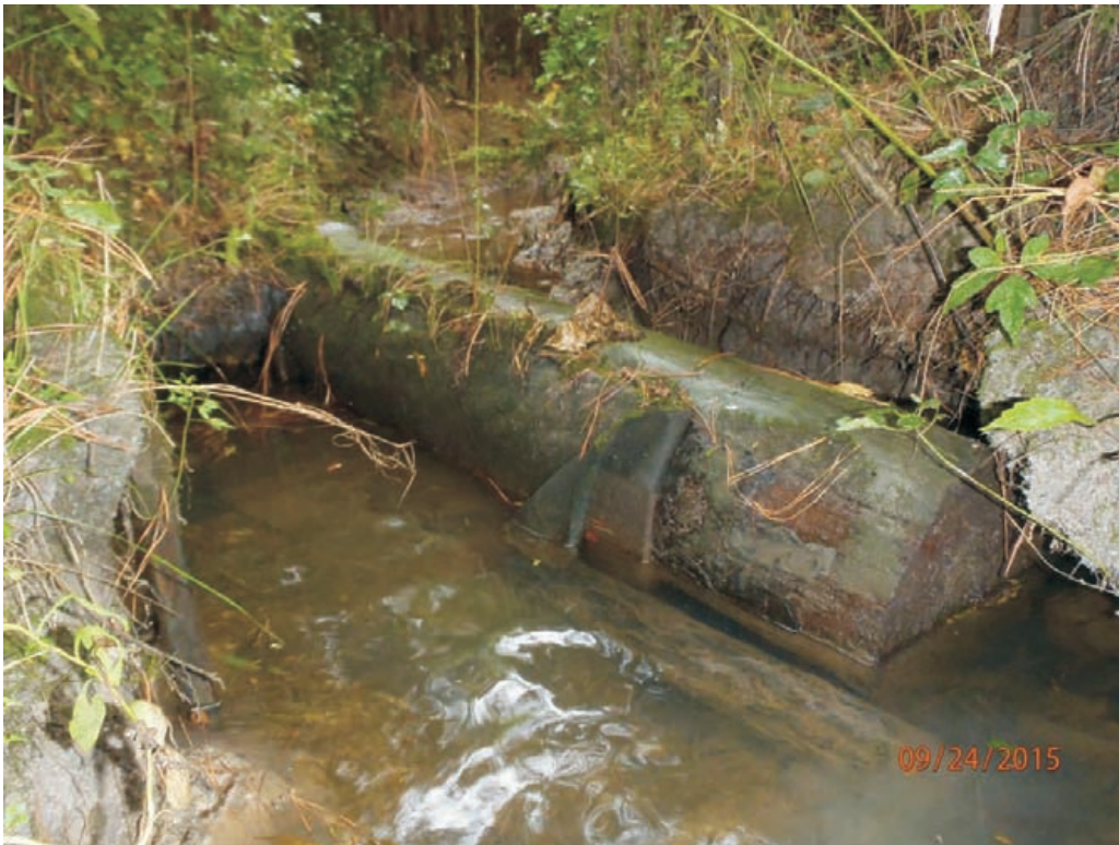
Reach 2A - Stream Problem Area #34; Log Vane Undercut
