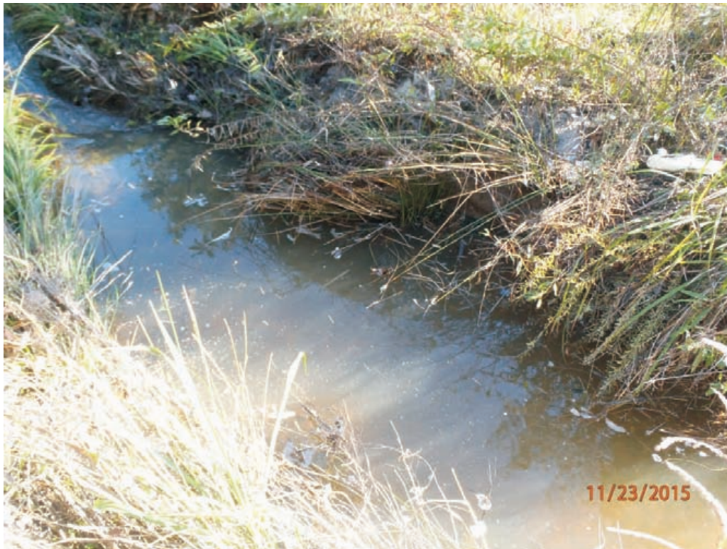
Reach 1A - Stream Problem Area #14; Scour
