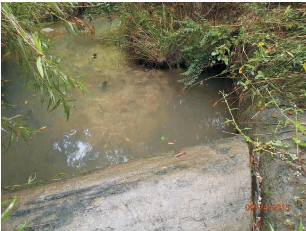
Reach 2A - Stream Problem Area #40; Log Vane Scour
