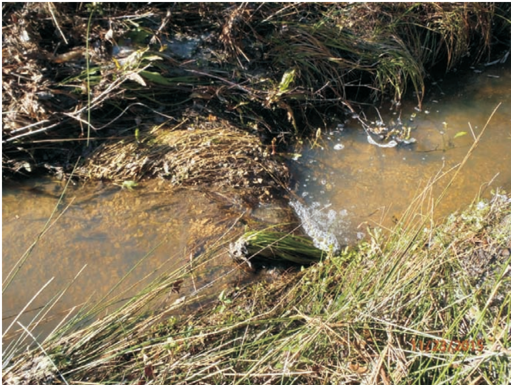
Reach 1A - Stream Problem Area #4; bank undercut
