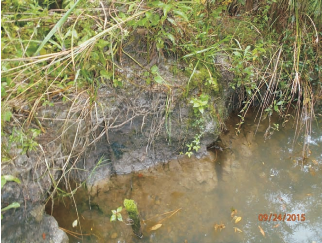
Reach 2A - Stream Problem Area #41; Scour
