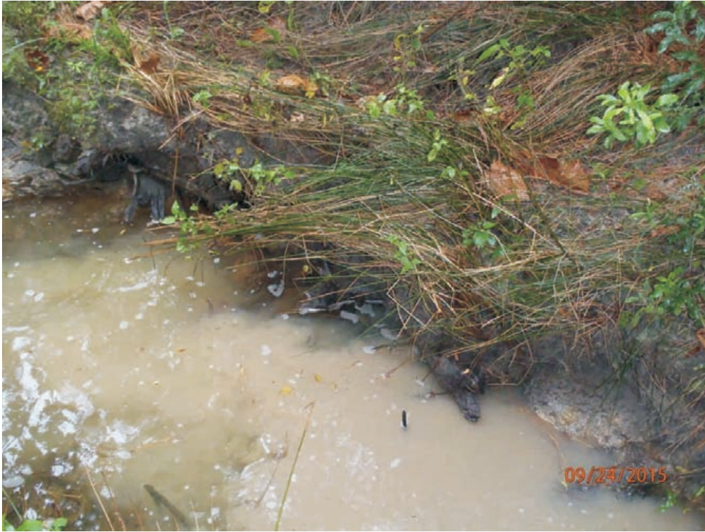
Reach 2A - Stream Problem Area #29; Scour
