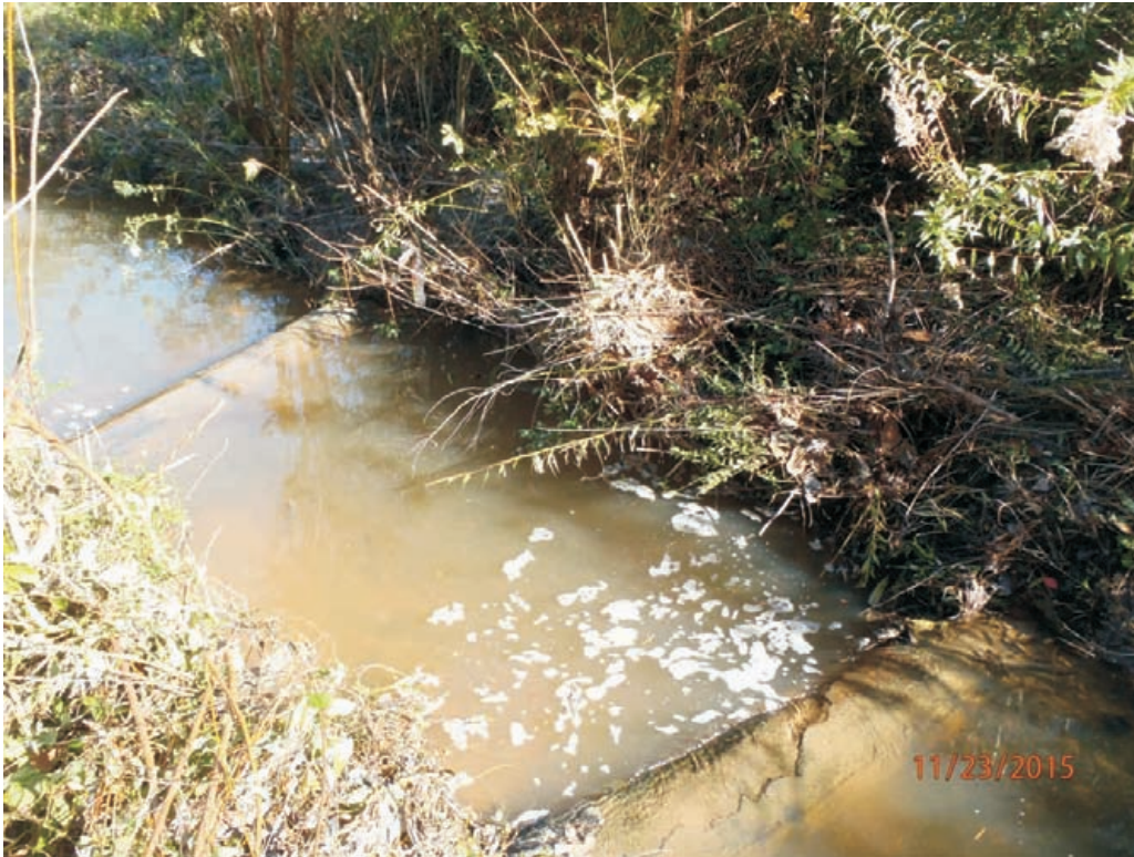
Reach 1A - Stream Problem Area #11; Log Vane Undercut
