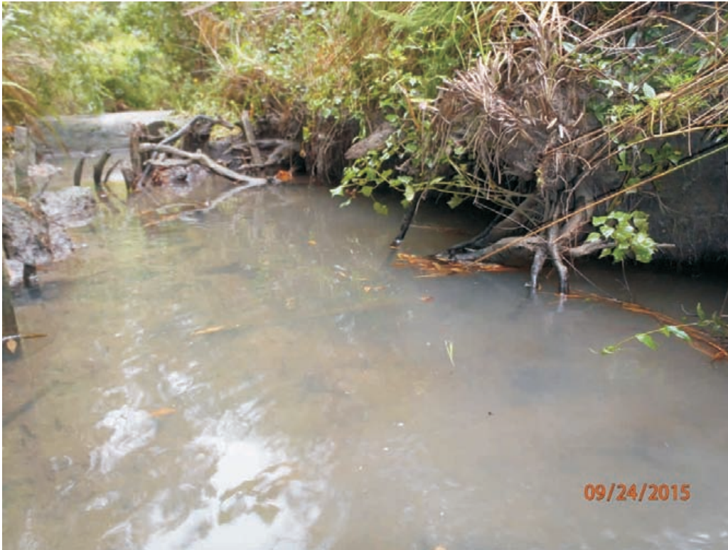
Reach 2A - Stream Problem Area #39; Undercut
