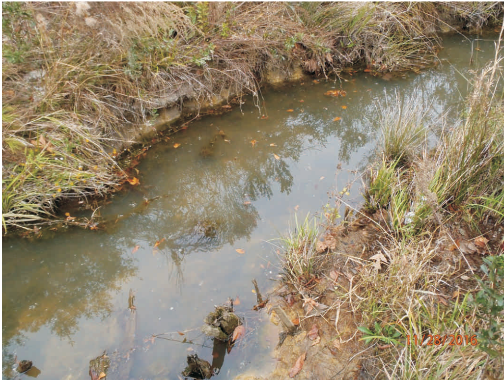
Reach 2A - Stream Problem Area #45; Scour
