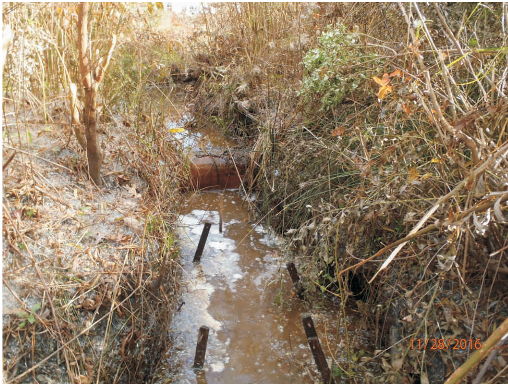
Reach B - Stream Problem Area #52b; Mass Wasting
