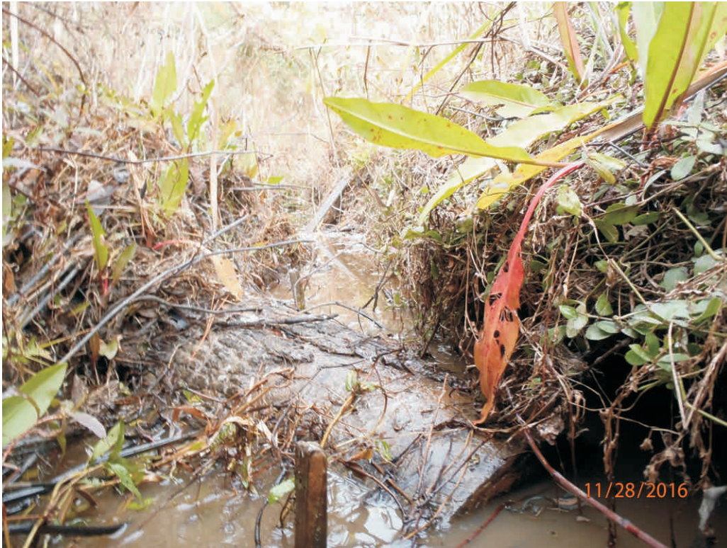
Reach 1A - Stream Problem Area #2a; scour along bank near log vane structure.
