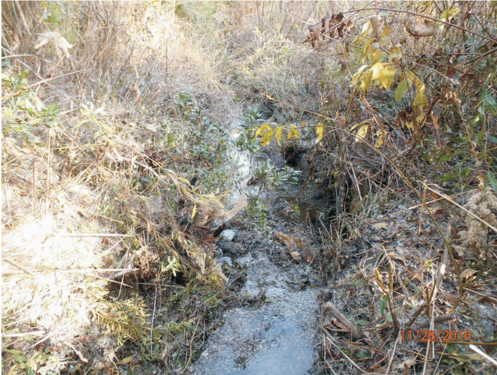
Reach 1A - Stream Problem Area #15; Degradation
