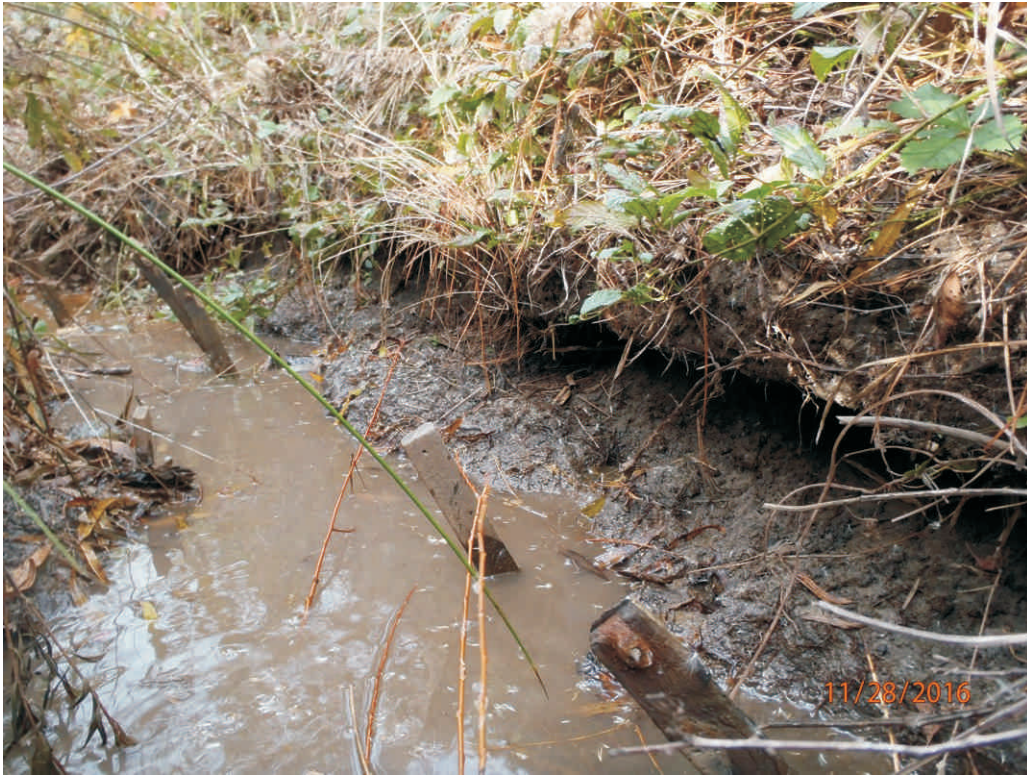
Reach B - Stream Problem Area #53; Undercut
