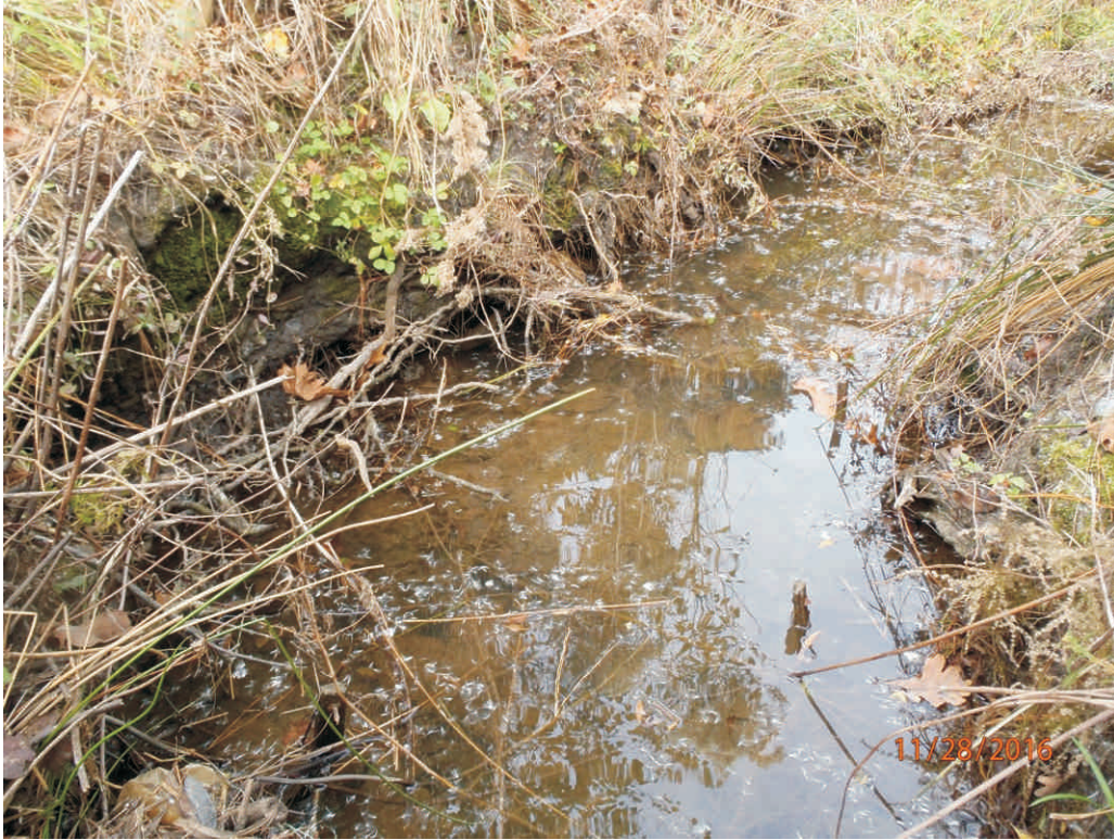
Reach 1A - Stream Problem Area #5; bank undercut becoming scour
