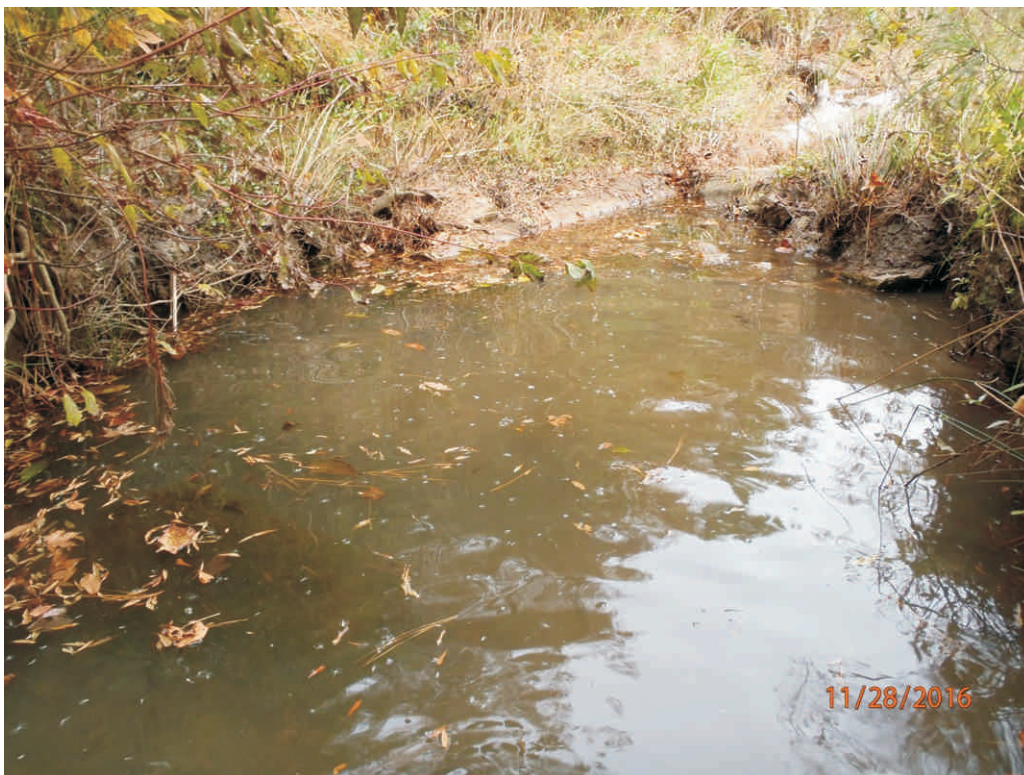
Reach 2A - Stream Problem Area #41; Scour
