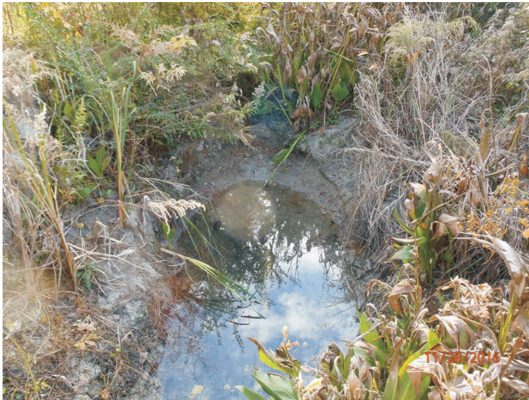
Enhancement Reach - Stream Problem Area #57c; Scour
