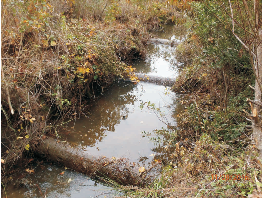
Reach 2A - Stream Problem Area #50a; Scour below Log Vanes
