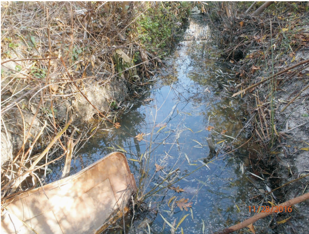
Reach 1A - Stream Problem Area #20a; Scour
