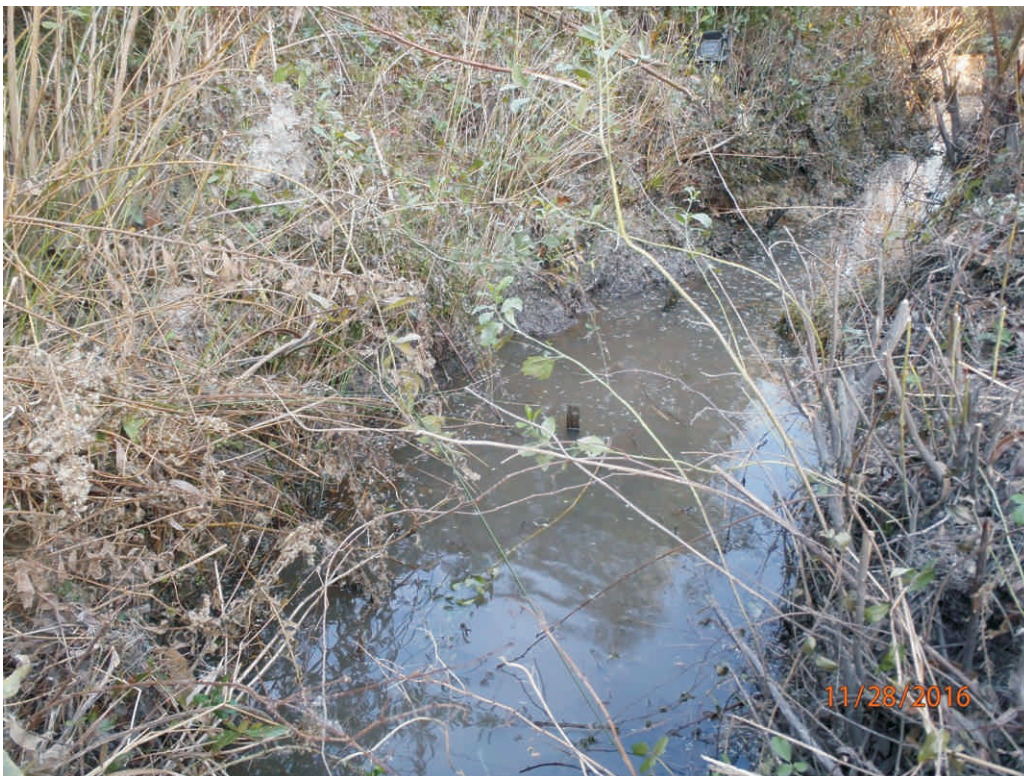
Reach 1A - Stream Problem Areas #18 & 19; Scour & Mass Wasting
