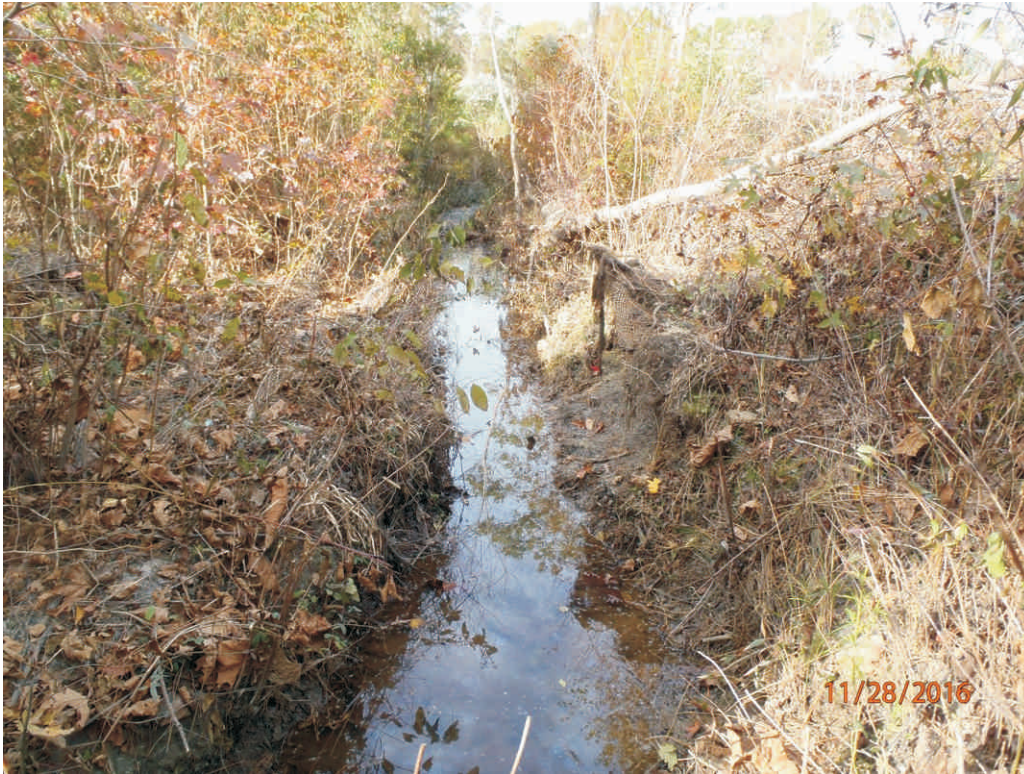
Reach 1A - Stream Problem Area #23; Degradation
