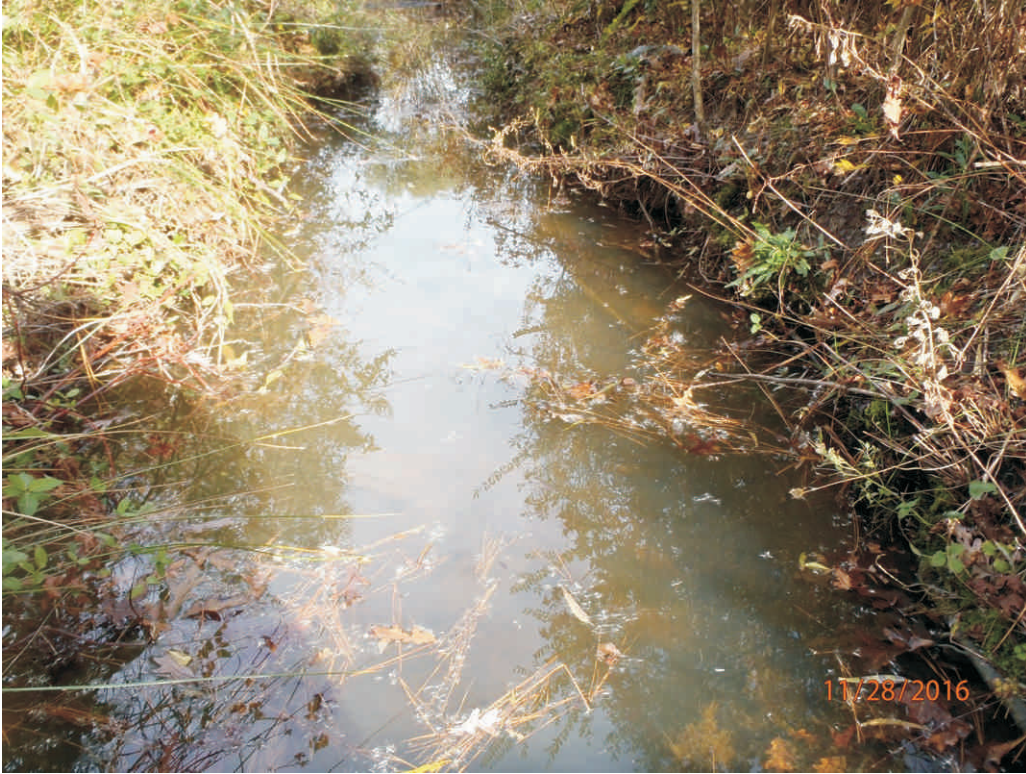
Reach 1A - Stream Problem Area #11; Log Vane Undercut becoming scour
