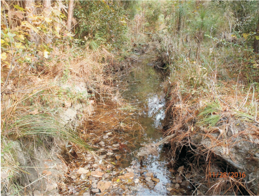
Reach 2A - Stream Problem Areas #38 & 39; Long Degradation and Undercut
