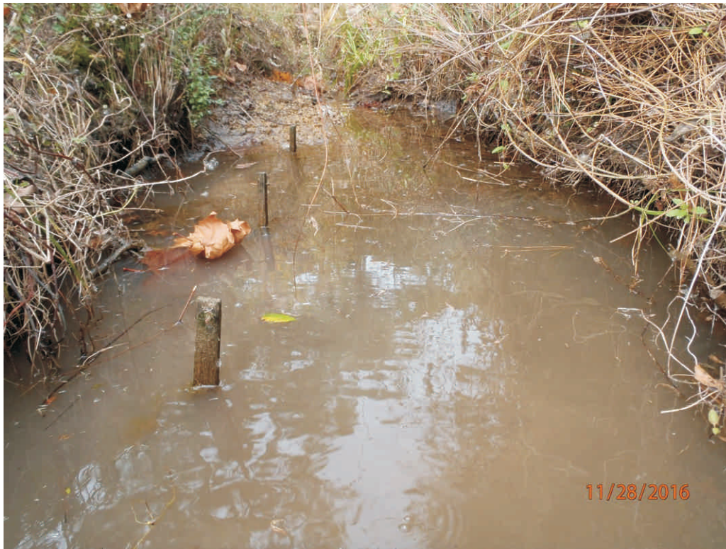
Reach 1A - Stream Problem Area #4; bank undercut
