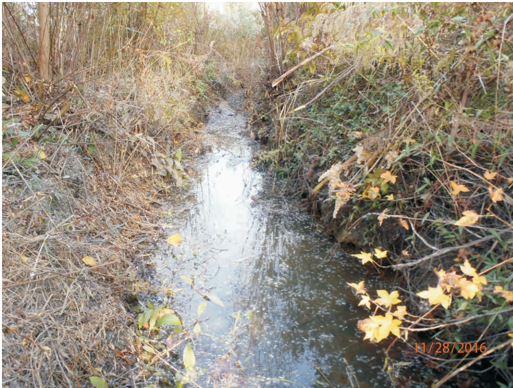
Reach 1A - Stream Problem Area #17; Degradation
