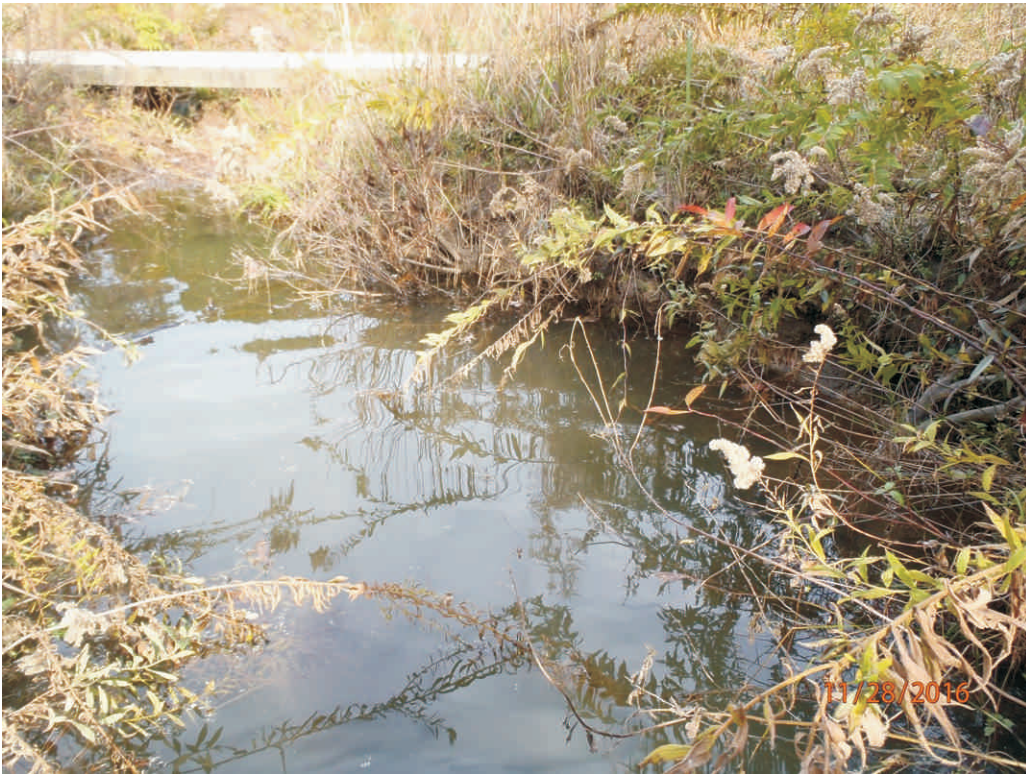
Reach 1A - Stream Problem Area #12; Scour
