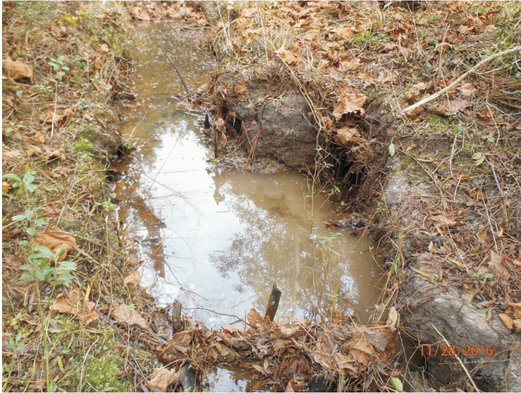
Reach 2A - Stream Problem Area #33; Scour
