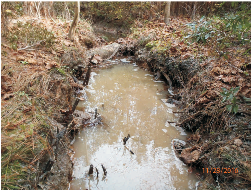
Reach 2A - Stream Problem Area #30; Log Vane Scour
