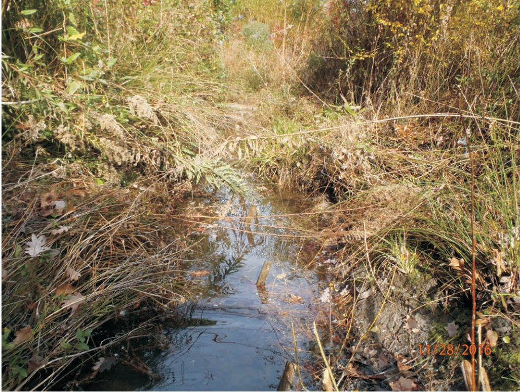
Reach 1A - Stream Problem Area #9; Degradation
