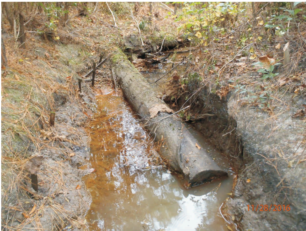
Reach 2A - Stream Problem Area #35a; Log Vane Scour
