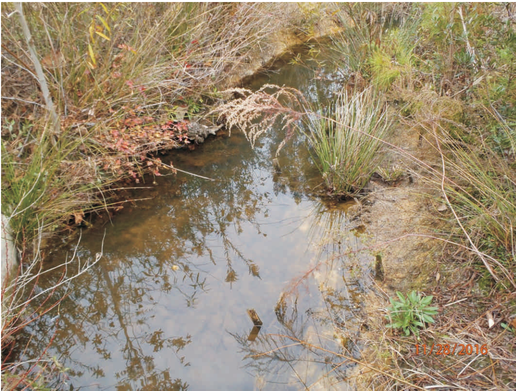
Reach 2A - Stream Problem Areas #47-48; Scour
