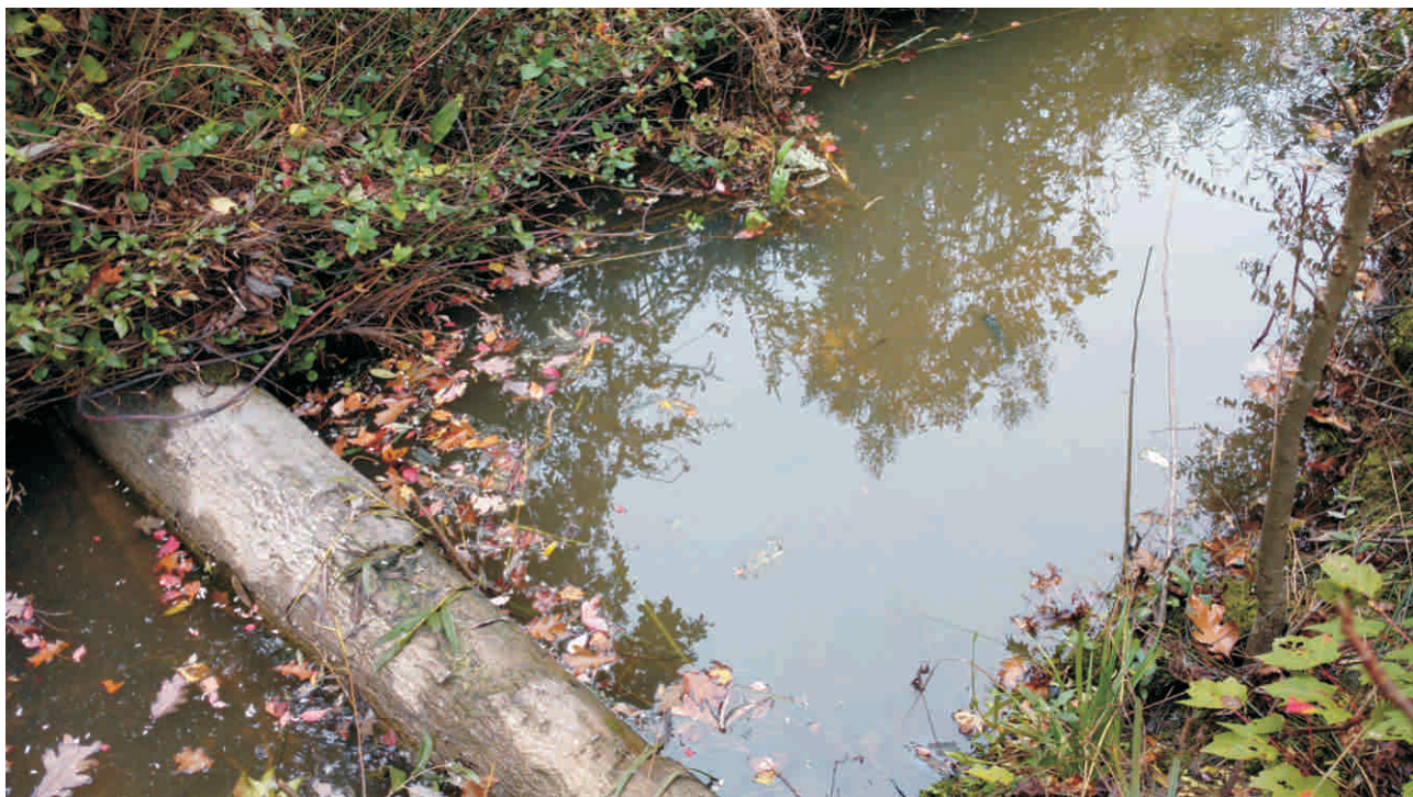
Reach 1A - Stream Problem Area #11; Log Vane Undercut becoming scour
