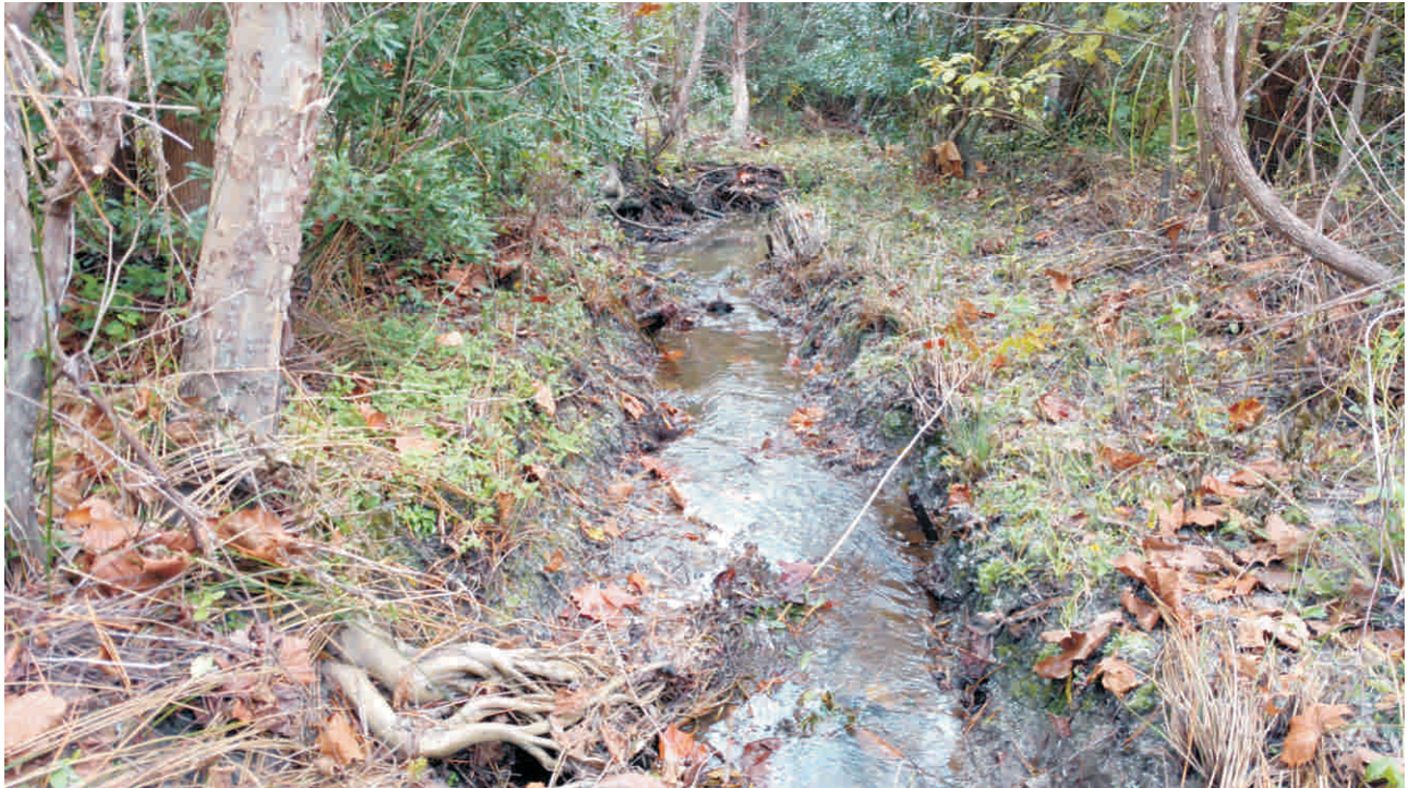
Reach 2A - Stream Problem Area #28; Degradation
