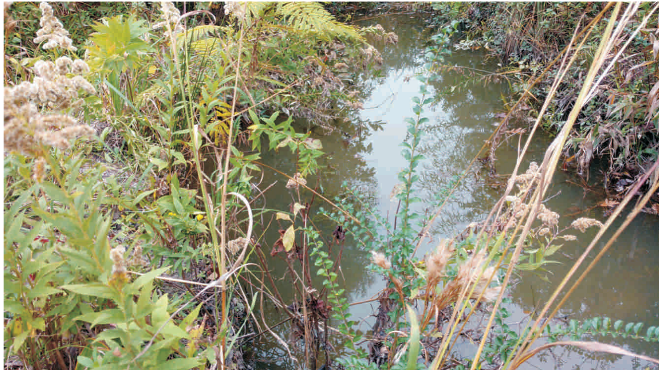
Reach 1A - Stream Problem Area #12; Scour
