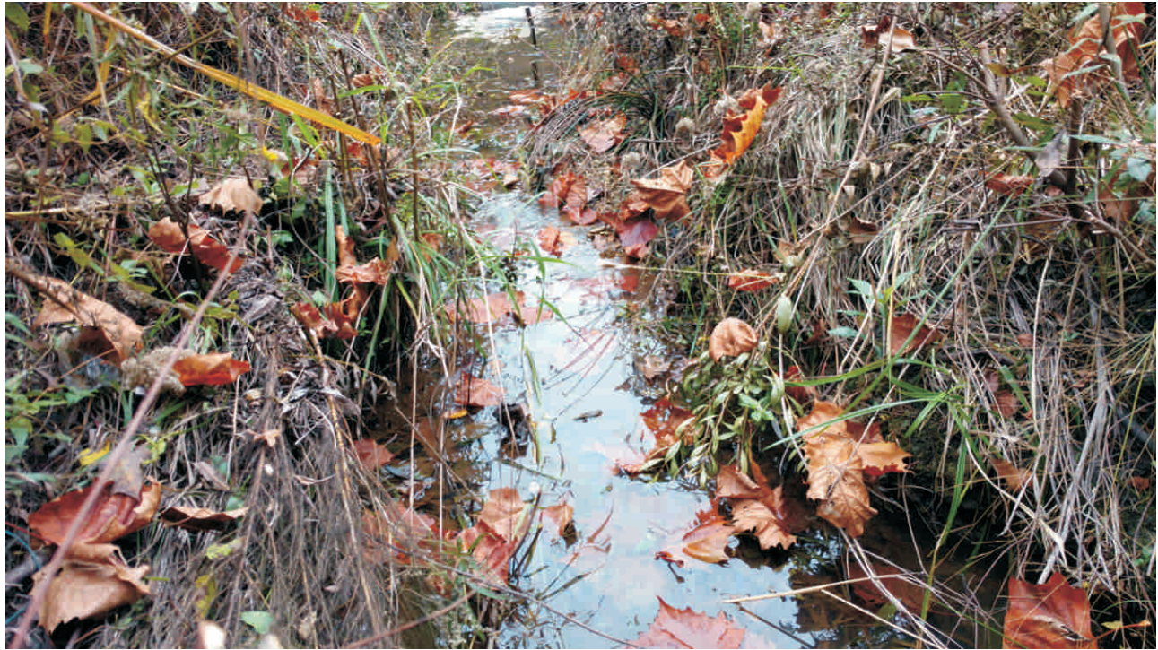
Reach 1A - Stream Problem Area #4; bank undercut
