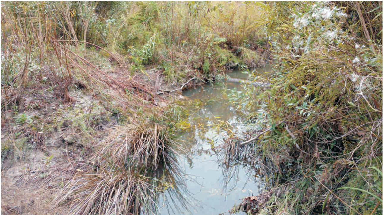
Reach 2A - Stream Problem Areas #47-48; Scour
