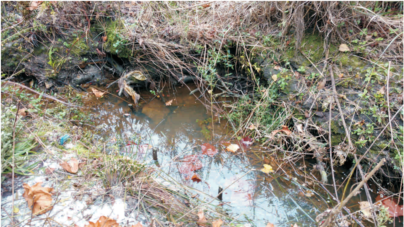
Reach 1A - Stream Problem Area #5; scour
