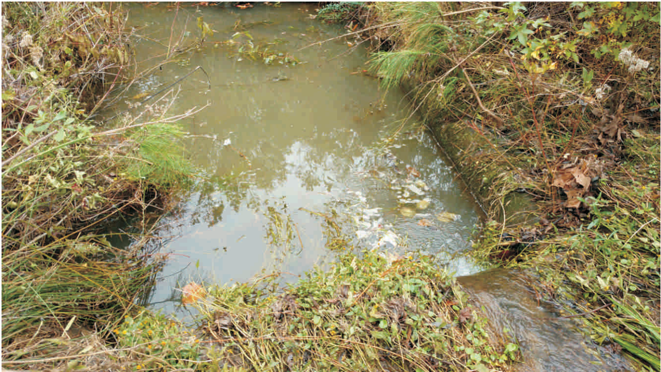
Reach 2A - Stream Problem Area #50a; Scour below Log Vane
