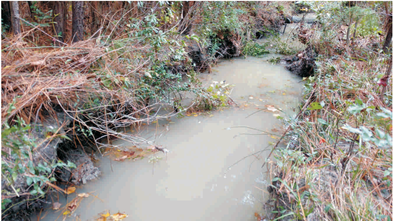
Reach 2A - Stream Problem Areas #38 & 39; Degradation and Undercut
