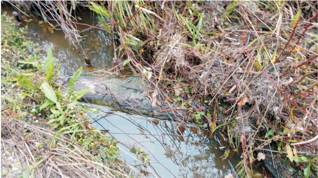
Reach 1A - Stream Problem Area #2a; scour along bank near log vane structure.
