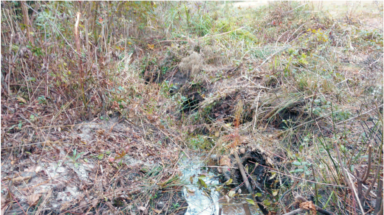
Reach B - Stream Problem Area #53; Undercut
