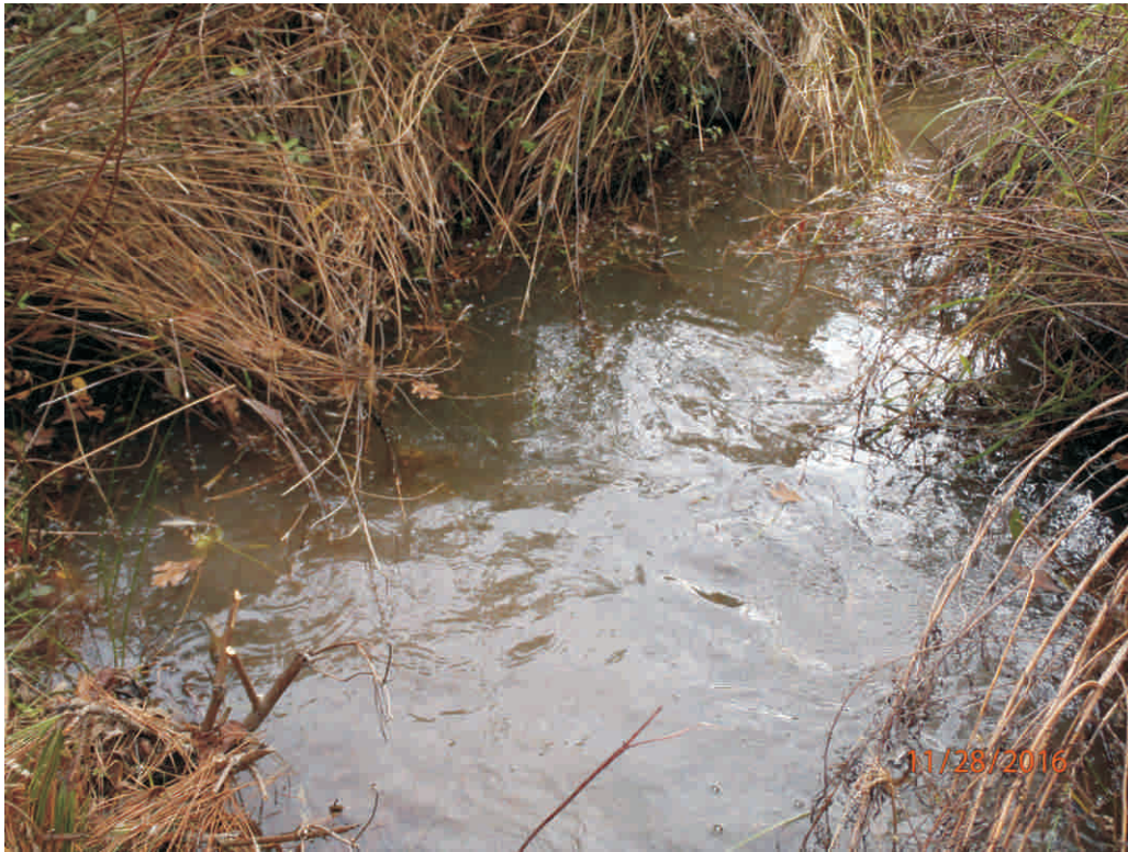
Reach 1A - Stream Problem Area #3a; scour
