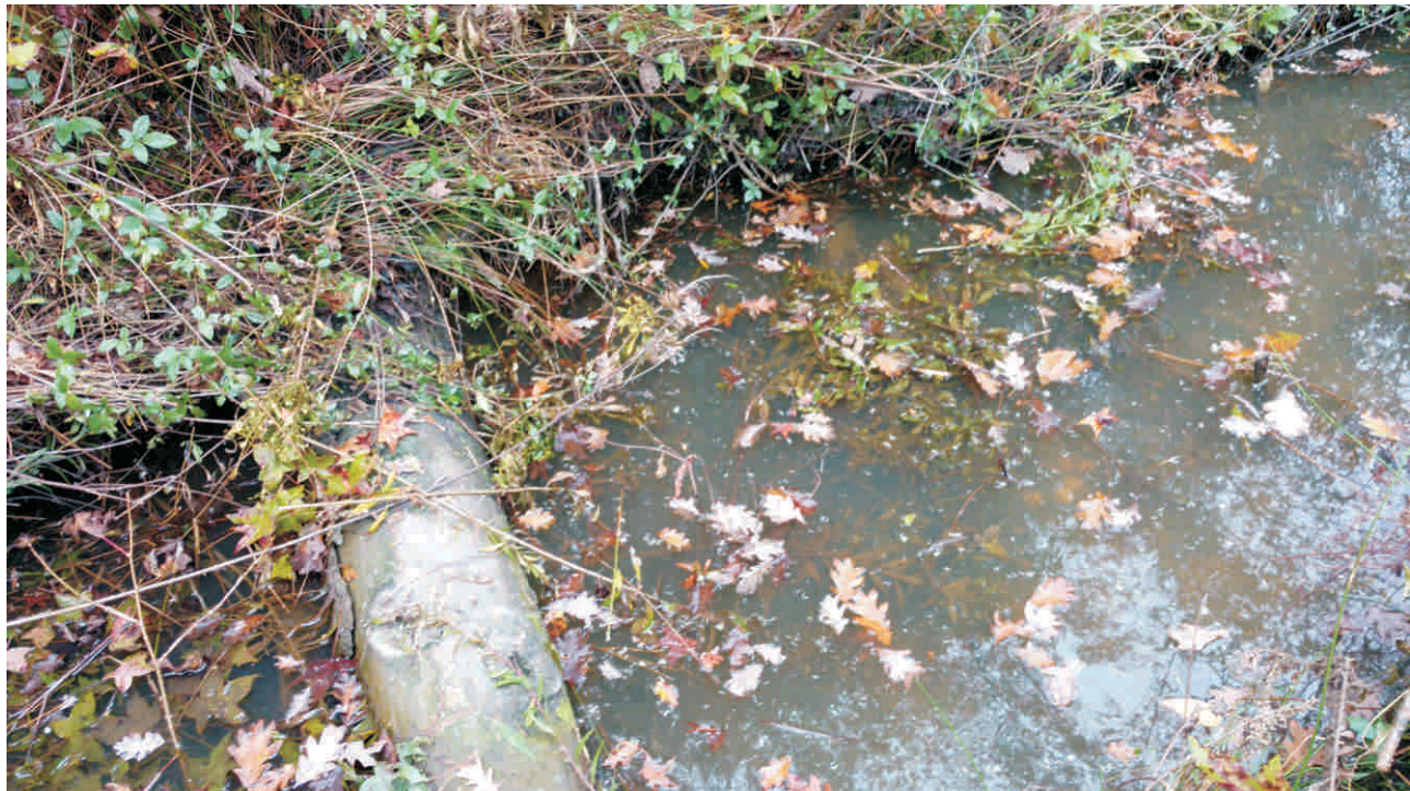
Reach 1A - Stream Problem Area #10; Log Vane Undercut becoming scour
