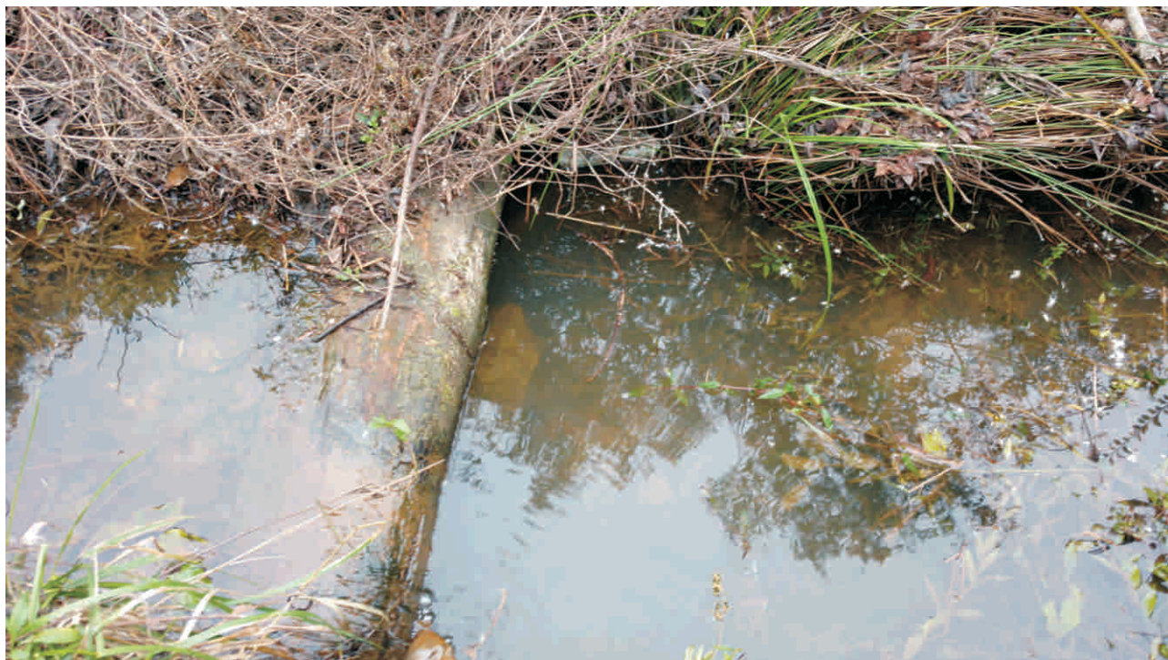
Reach 1A - Stream Problem Area #13aa; Log Vane Undercut
