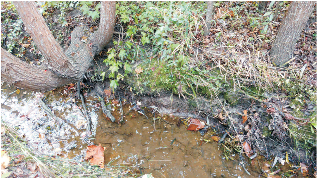
Reach 1A - Stream Problem Area #21; Bank Undercut
