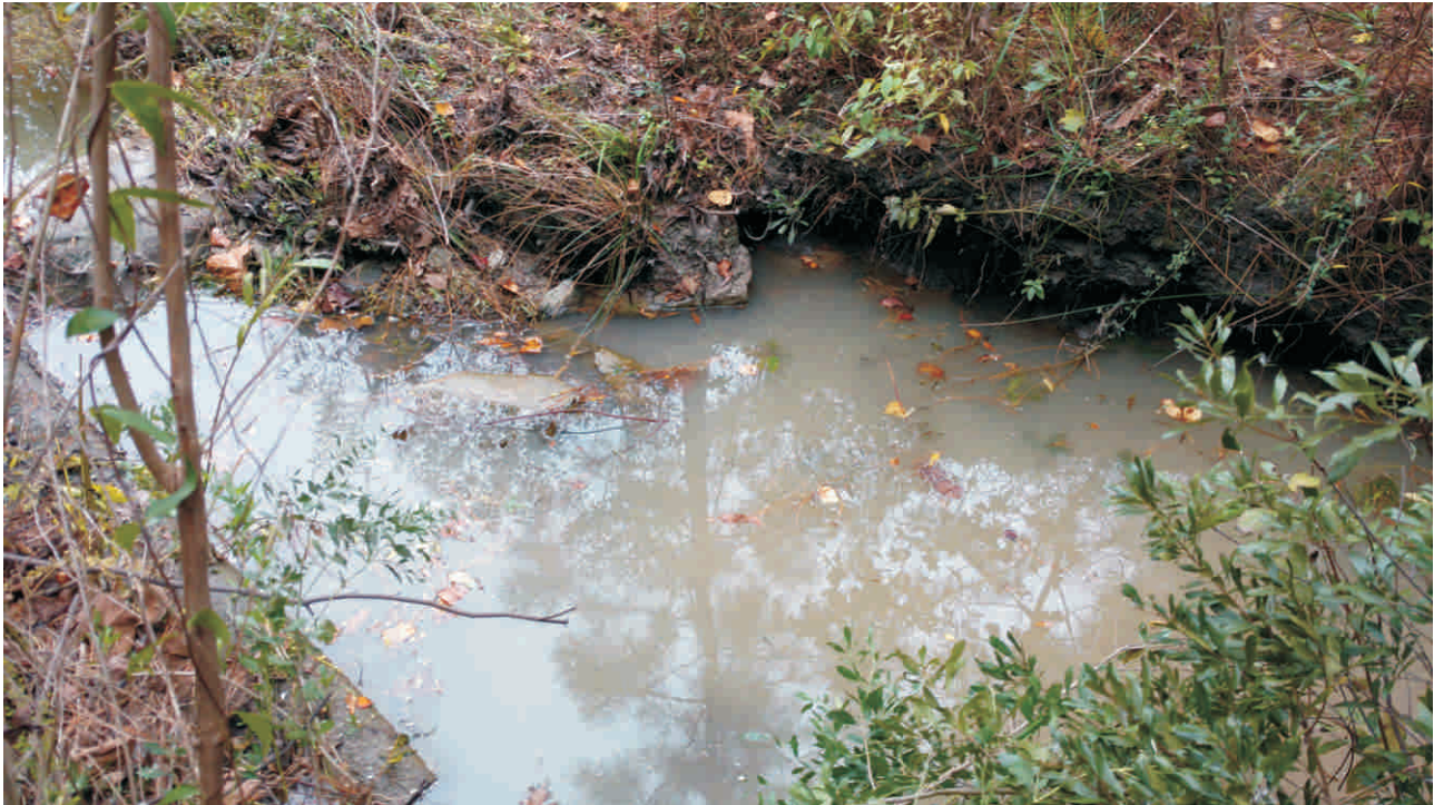
Reach 2A - Stream Problem Area #41; Scour
