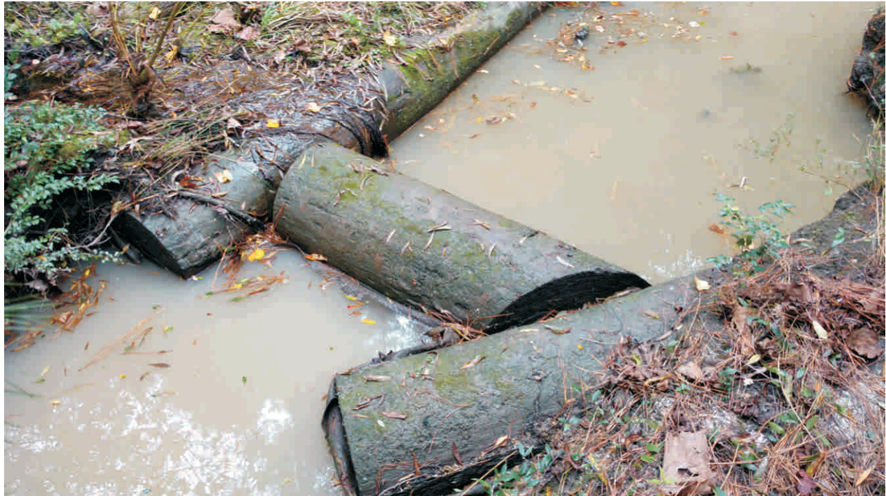
Reach 2A - Stream Problem Area #40; Log Vane Scour
