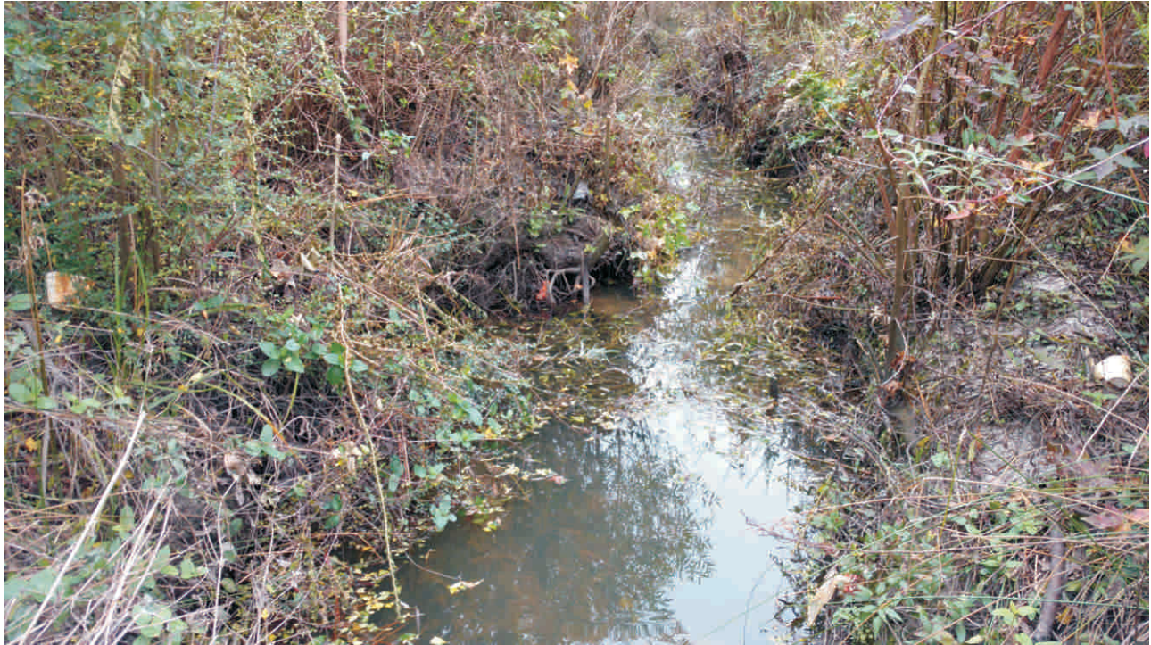
Reach 1A - Stream Problem Area #14; Scour
