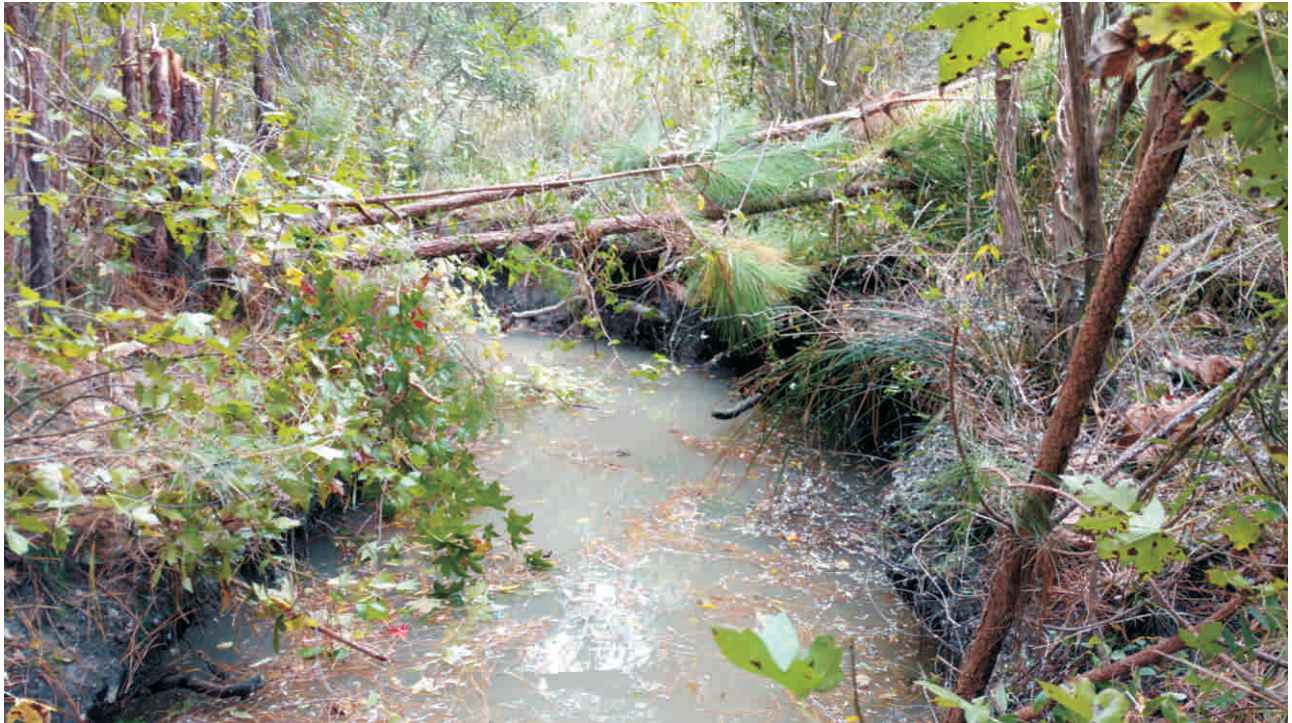
Reach 2A - Stream Problem Area #37; Undercut turning into Mass Wasting
