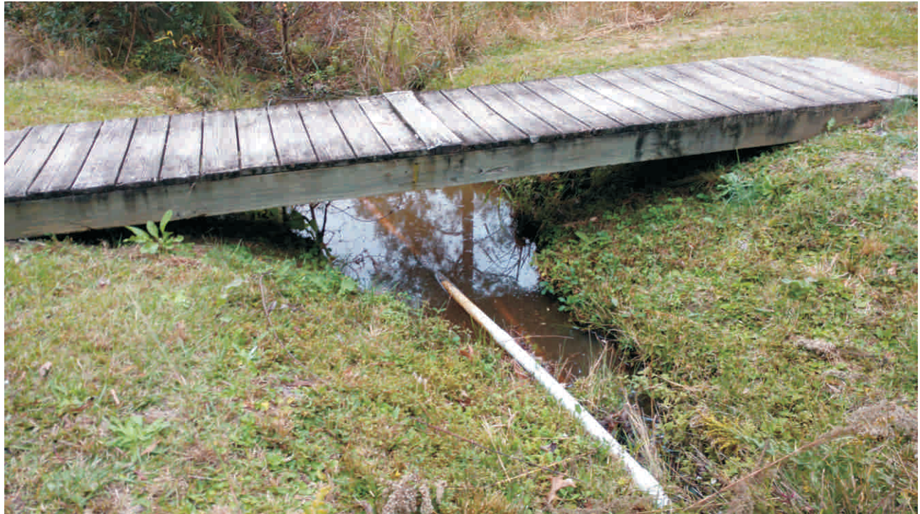
Enhancement Reach - Stream Problem Area #57a; Scour
