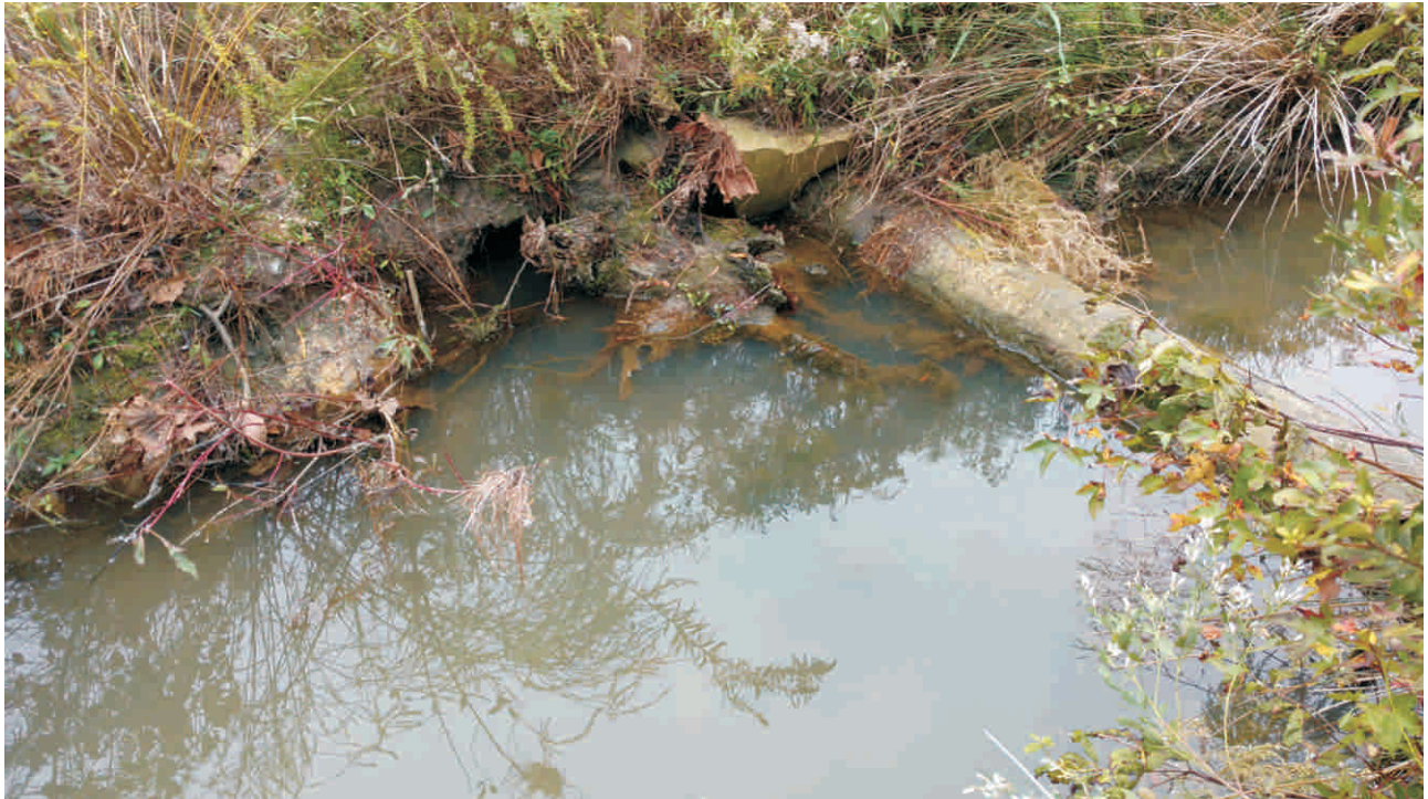
Reach 2A - Stream Problem Area #45a; Log Vane Scour
