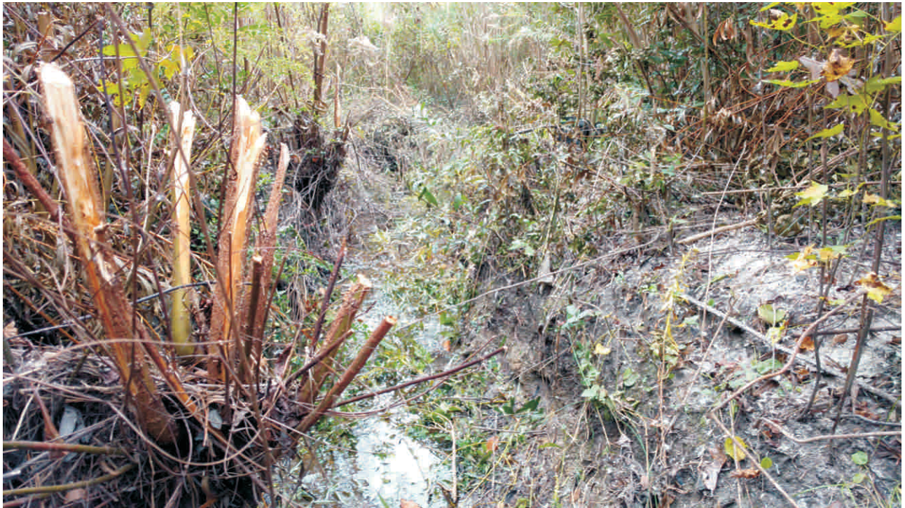
Reach 1A - Stream Problem Area #20a; Scour
