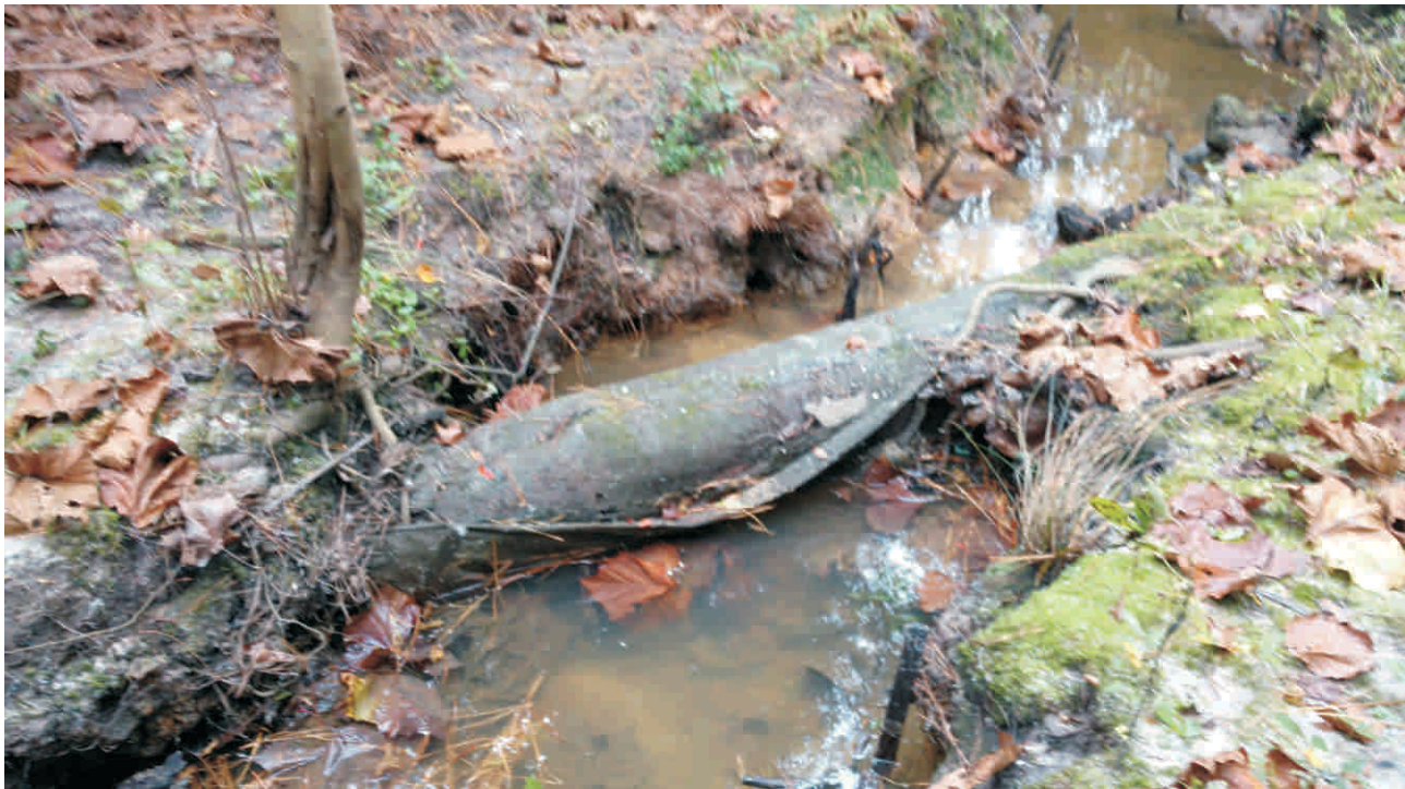
Reach 2A - Stream Problem Area #30 & 31; Log Vane Scour
