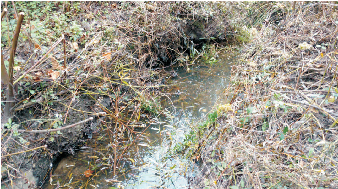
Reach 1A - Stream Problem Area #16; Scour
