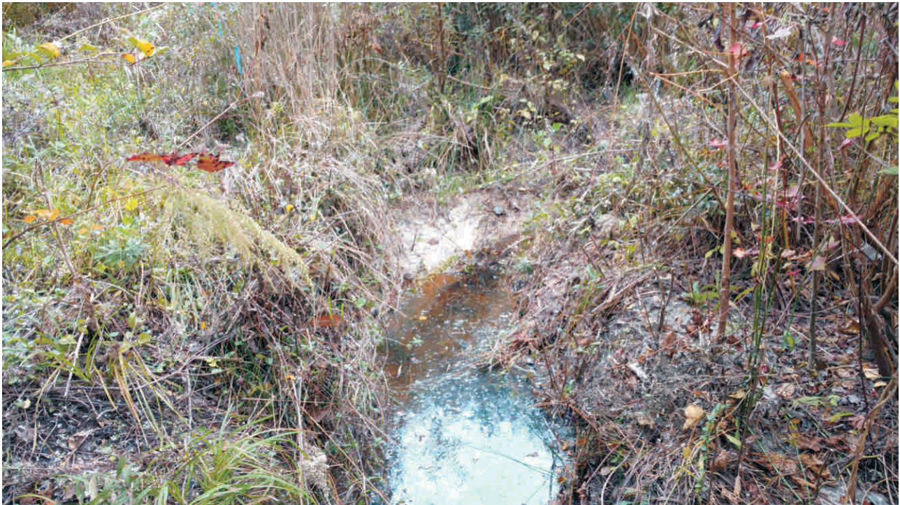
Reach B - Stream Problem Area #52; Mass Wasting
