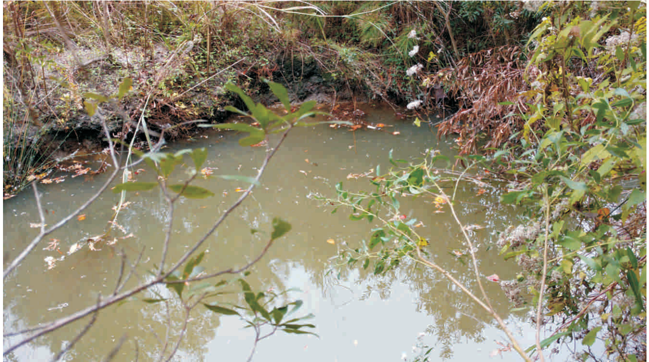
Reach 2A - Stream Problem Area #43a; Scour
