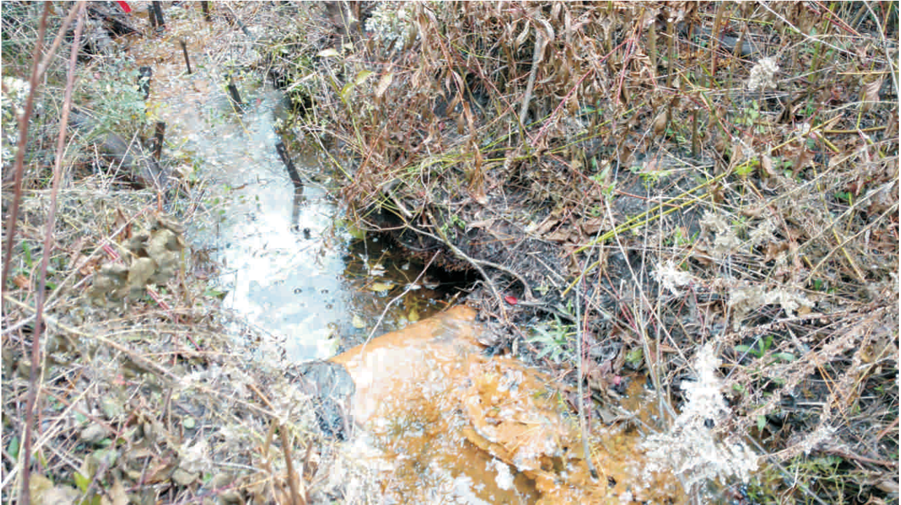
Reach B - Stream Problem Area #52a; Log Vane Undercut
