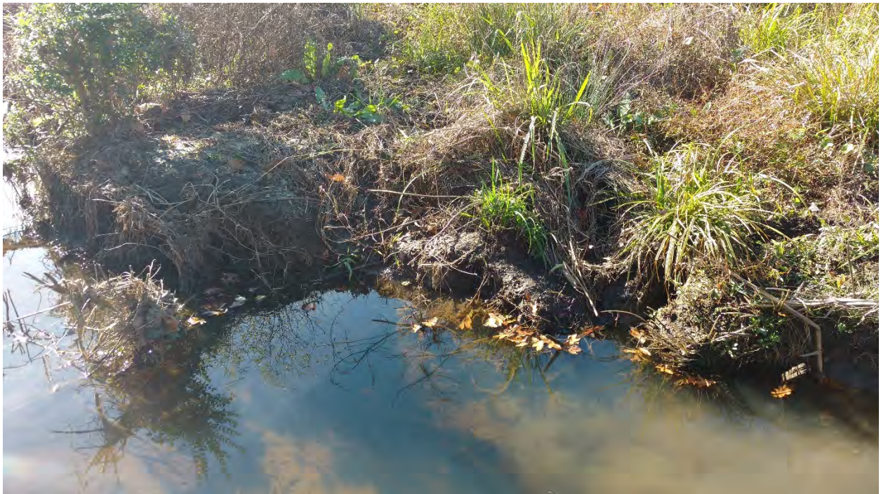
Reach C: Stream Problem Area 63 – Mass Wasting
