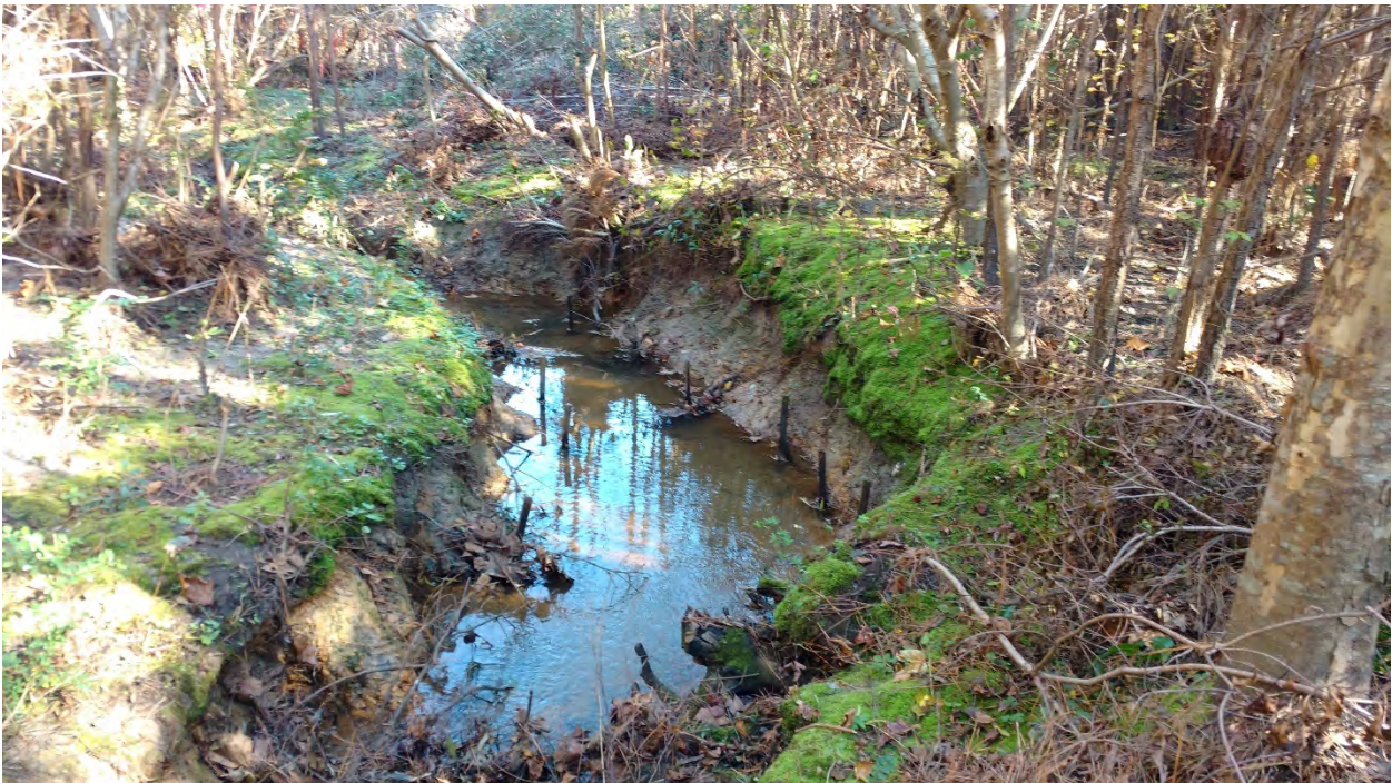
Reach 2A: Stream Problem Area 31 – Scour
