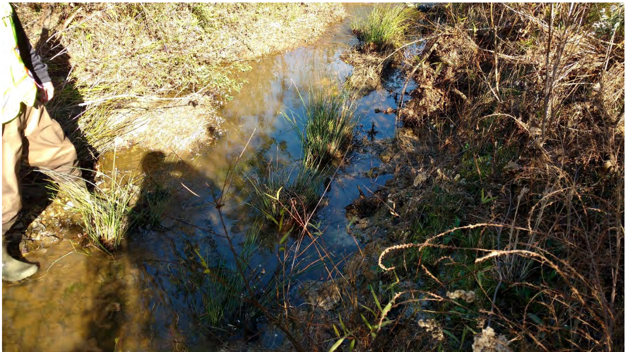
Reach 2A: Stream Problem Area 47 – Scour
