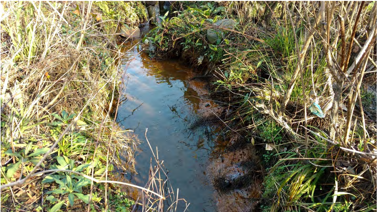
Reach 1A: Stream Problem Area 2 – Undercut near Log Vane Structure
