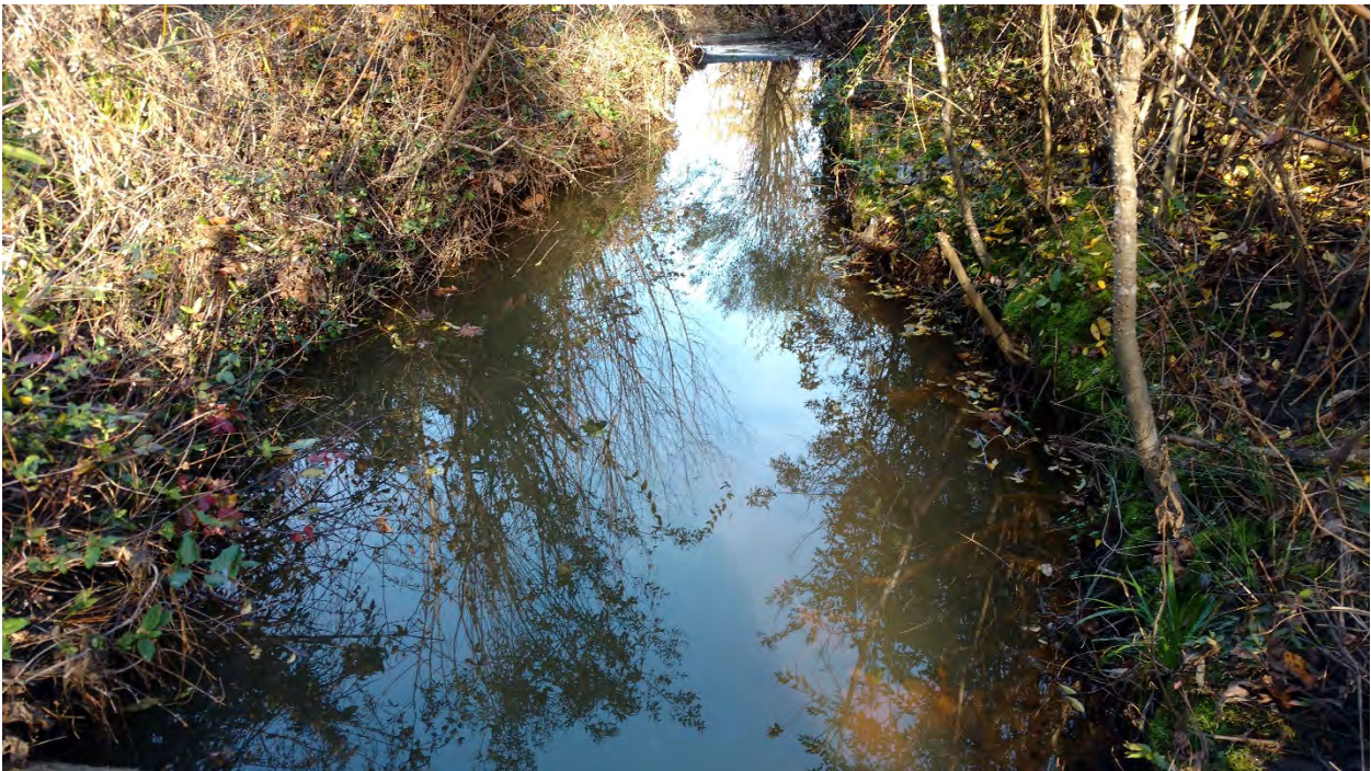
Reach 1A: Stream Problem Area 10 – Scour
