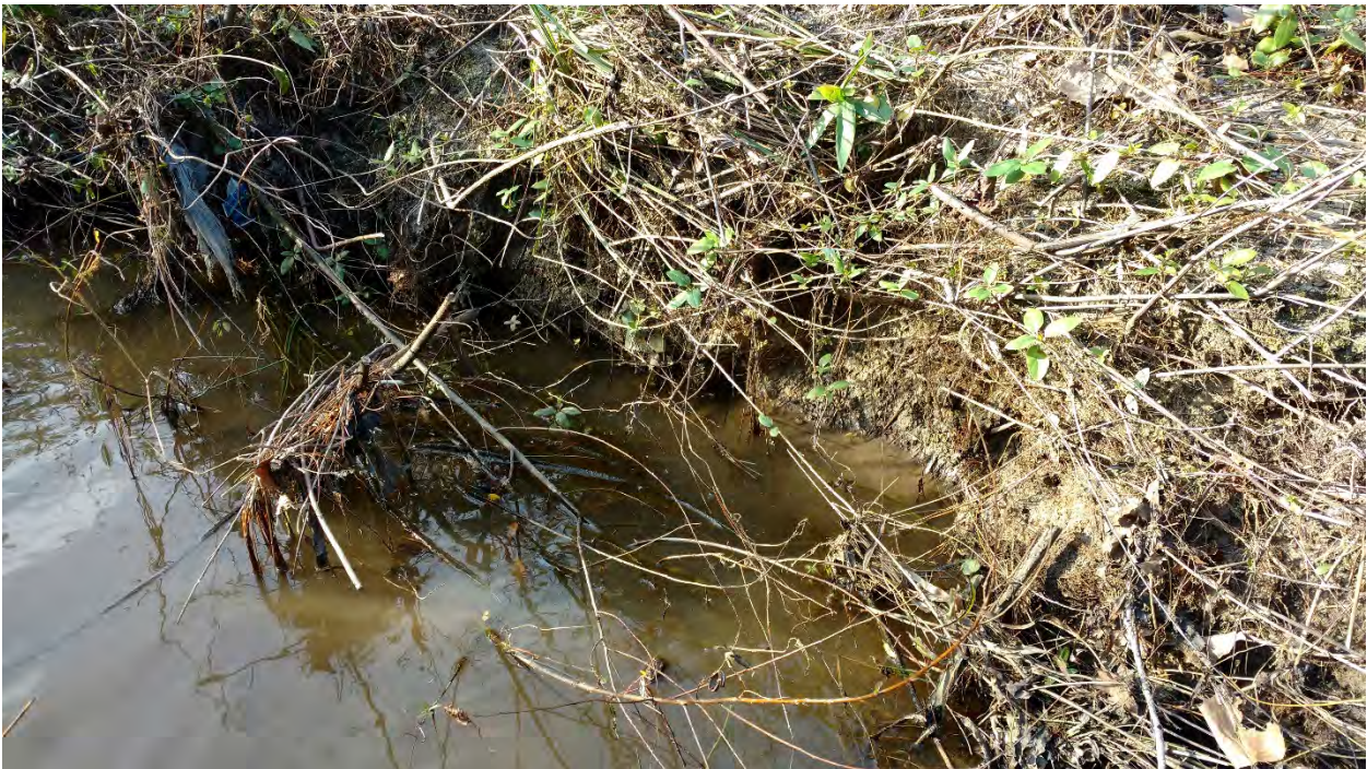
Reach 1A: Stream Problem Area 13a – Scour
