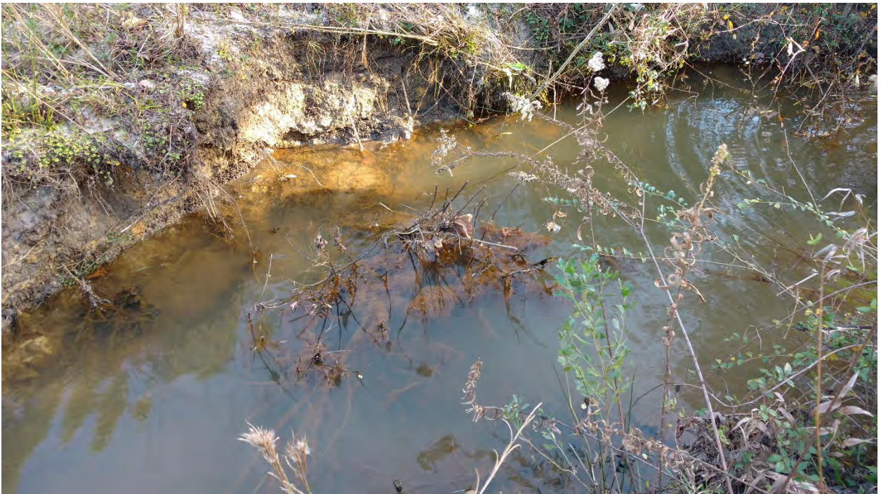
Reach 1A: Stream Problem Area 12 – Mass Wasting
