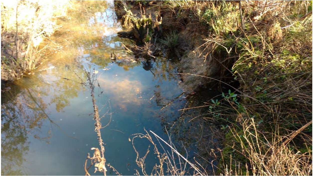
Reach 2A: Stream Problem Area 44 – Scour
