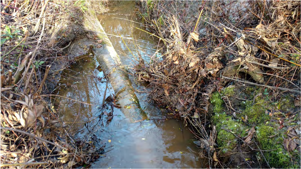
Reach 1A: Stream Problem Area 16 – Scour after log vane structure. Structure appears to be failing.
