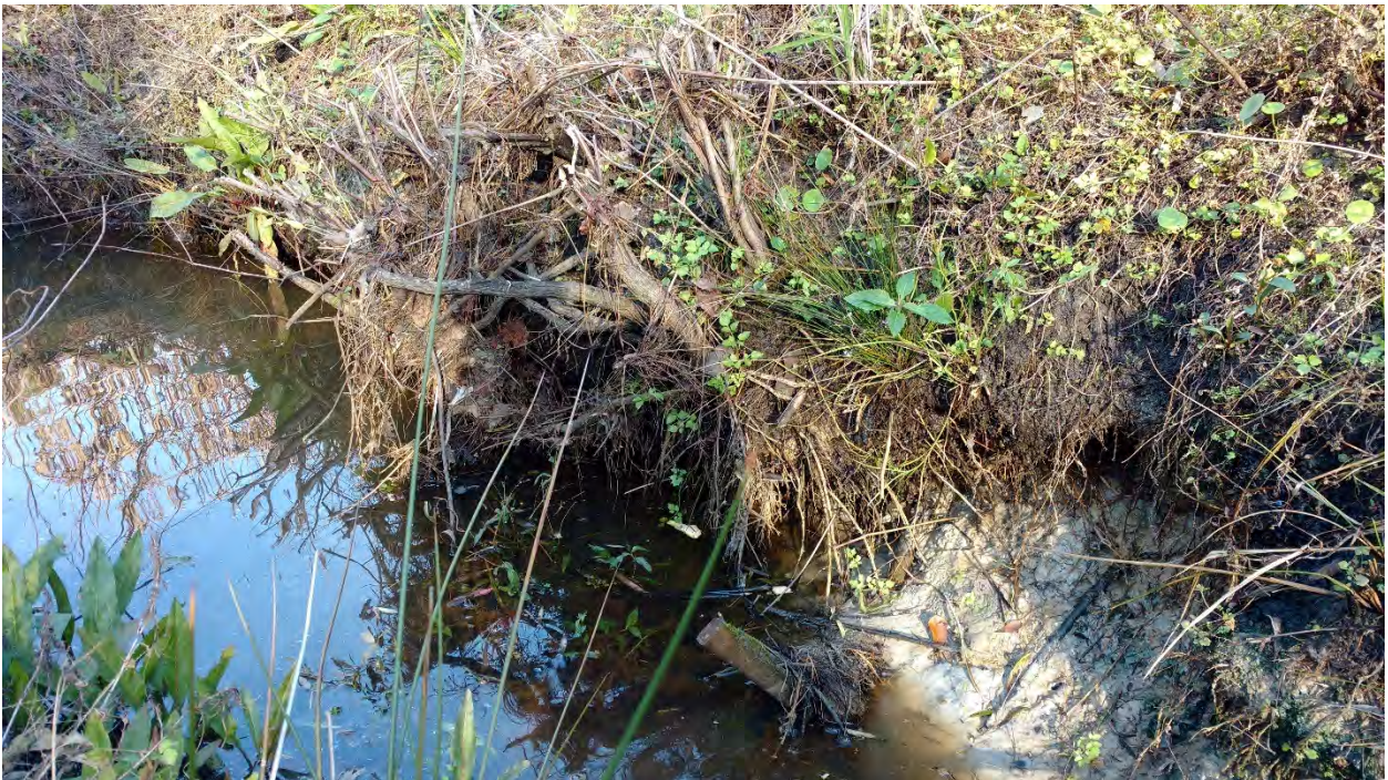
Reach 1A: Stream Problem Area 2c – Undercut/Scour
