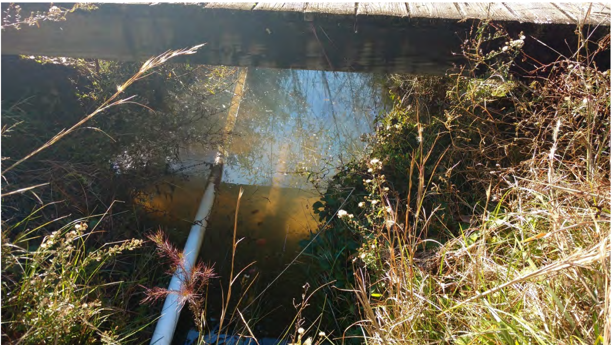
Enhancement Reach: Stream Problem Area 57a – Scour near footbridge
