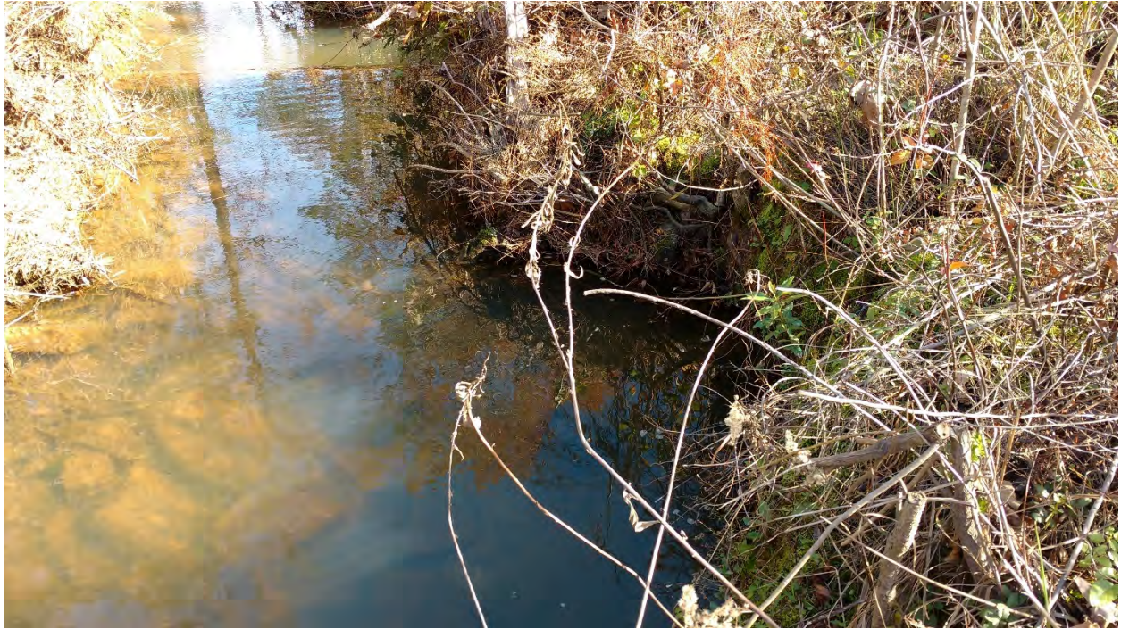
Reach 2A: Stream Problem Area 50 – Mass Wasting
