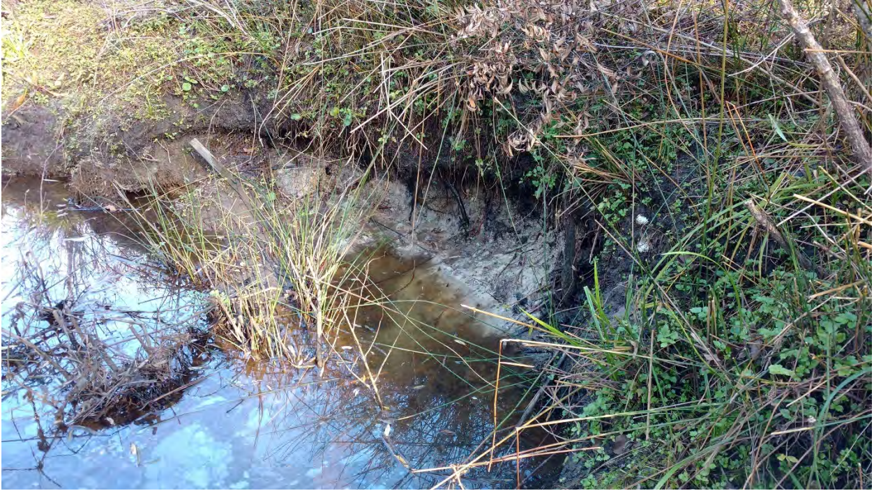
Reach 1A: Stream Problem Area 2a – Scour near Log Vane Structure
