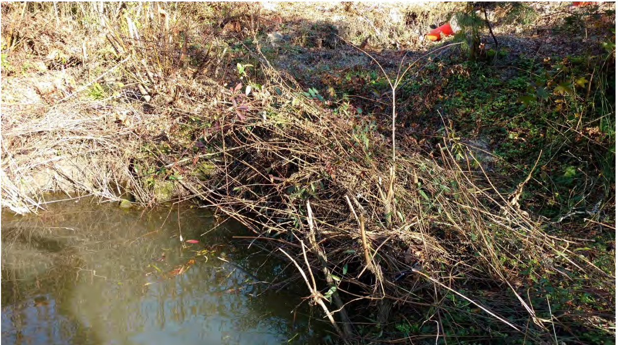
Reach 1A: Stream Problem Area 4 – Mass Wasting
