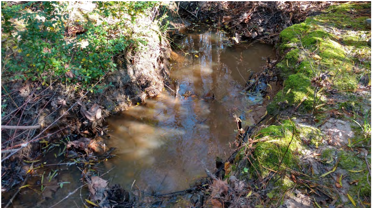
Reach 2A: Stream Problem Area 29 – Scour
