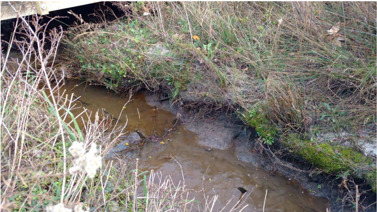
Reach 1A: Stream Problem Area 20a – Scour
