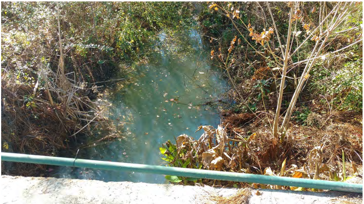
Enhancement Reach: Stream Problem Area 56d – Scour
