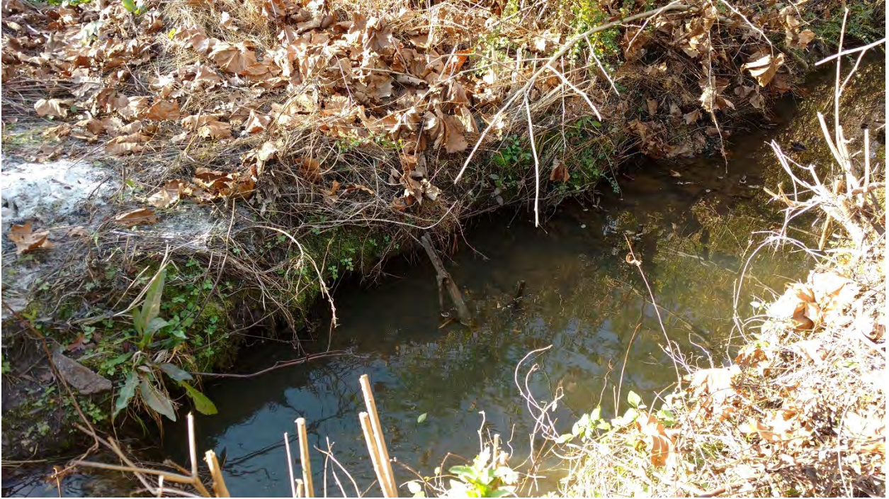
Reach 1A: Stream Problem Area 5 – Scour
