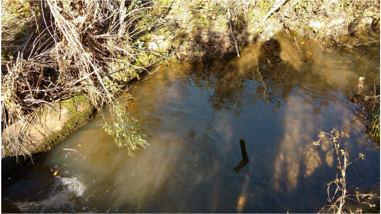
Reach 2A: Stream Problem Area 48 – Scour
