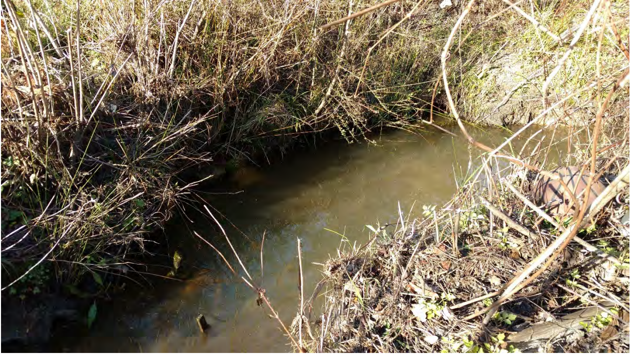
Reach 1A: Stream Problem Area 3b – Undercut on both sides of channel
