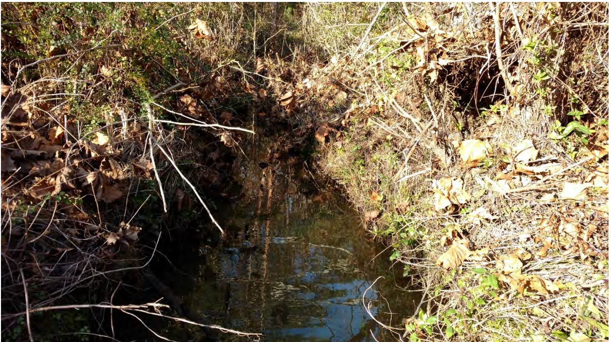
Reach 1A: Stream Problem Area 6 – Degradation
