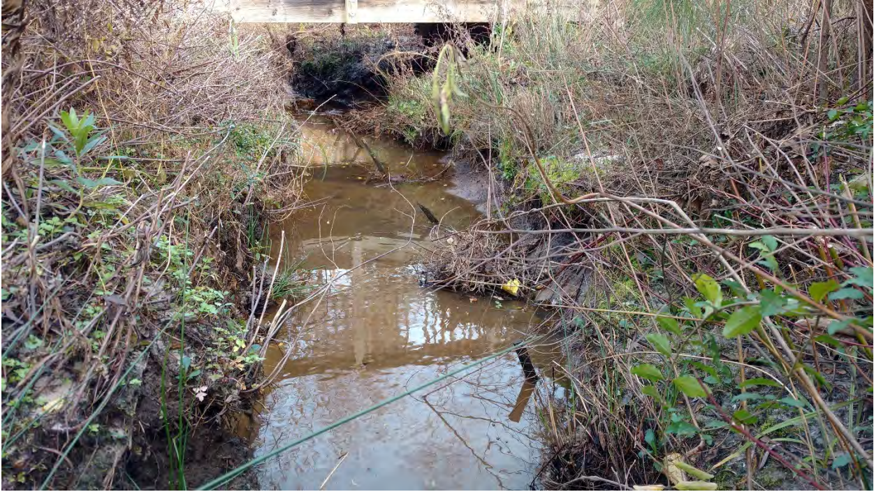
Reach 1A: Stream Problem Area 20 – Degradation
