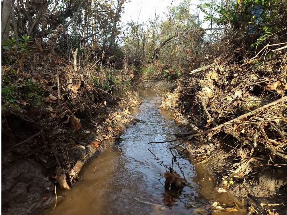
Reach 1A: Stream Problem Area 23– Degradation
