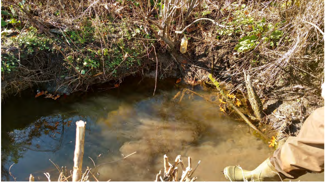
Reach C: Stream Problem Area 62 – Under Cut
