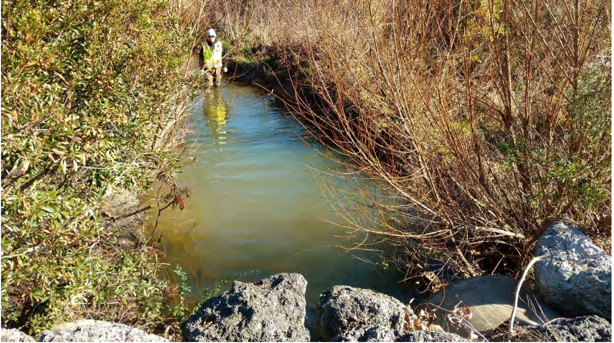
Reach 2A: Stream Problem Area 25 – Scour off of road
